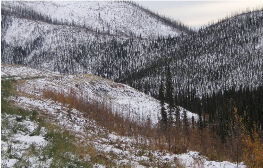
Photo 15: View of the slope instability below the Lucky Dump haul road taken from just east of the haul road crossing of Lucky Creek. Due to the snowfall/excessive vegetation, an inspection for tension cracks or recent ground movements could not be completed.
