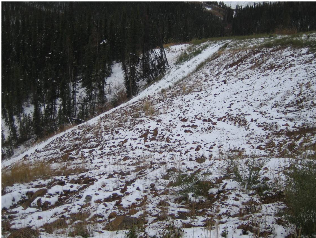
Photo 16: View of the second failure location by the Lucky Dump haul road above the Bohemian Access Trail, taken from “Photo Hub #4”.
