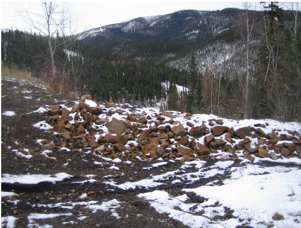
Photo 4: Rip-rap placed in 2009 near the outlet of the surface runoff collection ditch at the toe of the Blue Dump (1 of 2 locations). The outside bank was armoured for approx. 15m with a 30 cm thick layer with an average diameter of approx. 20cm.
