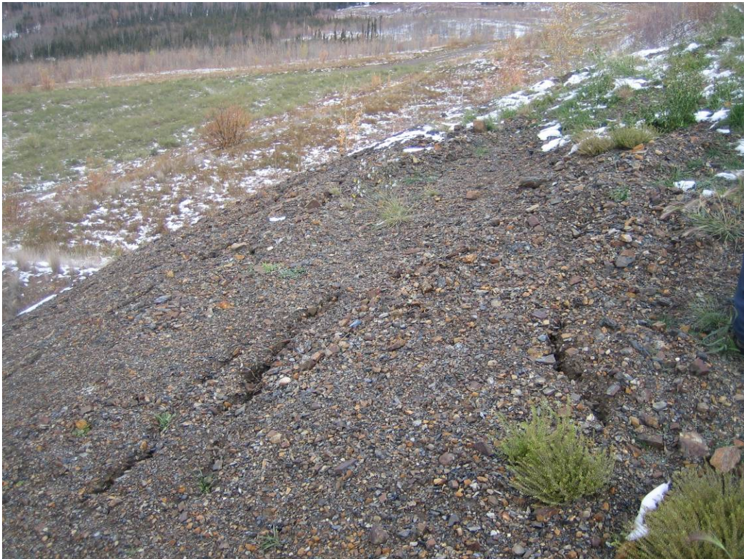
Photo 26: View of Tension cracks by the heap leach dyke near the breach location.
