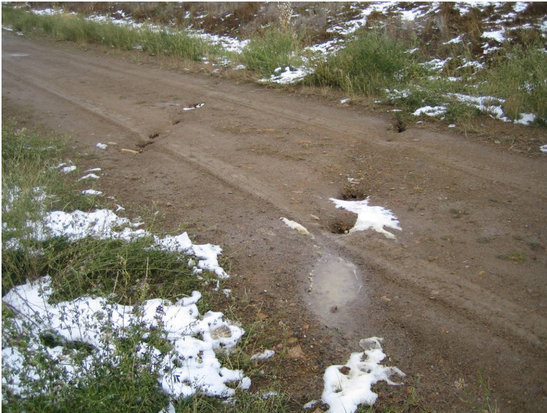
Photo 23: View of possible sinkhole cracking across the access road approx. 10m east of the Pacific Pit overflow. Photo taken looking towards the north side of the road.
