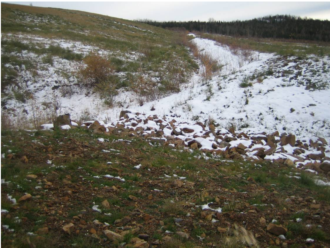
Photo 24: View of breach completed in 2009 of the heap leach pad dyke at the former emergency spillway location.
