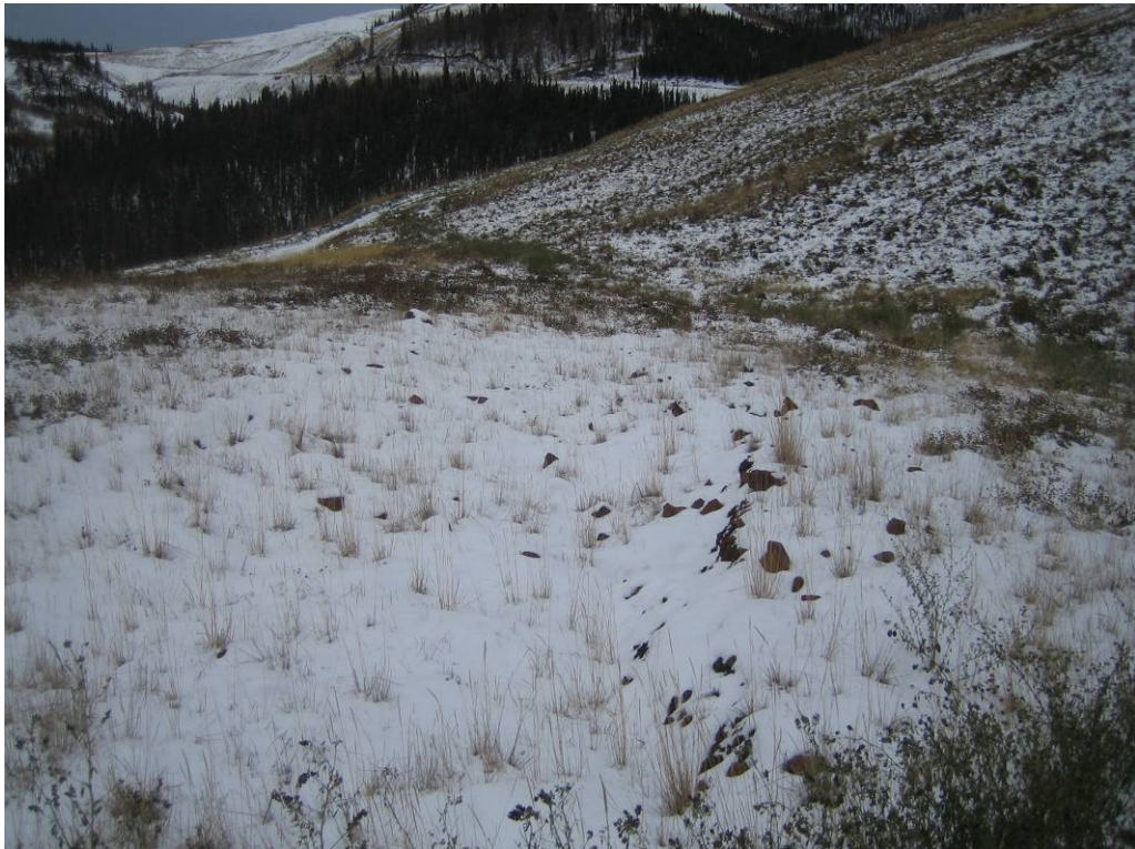
Photo 20: View of the “saddle area” of the Lucky WRSA where large differential settlements have occurred. Differential Settlement of approximately 0.5 m has occurred in the snowy area near the center of the photograph.
