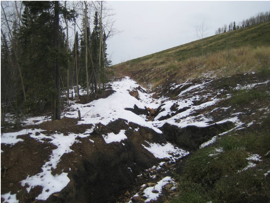
Photo 8: View of the eroded runoff collection ditch upstream of the 2 nd rip-rap location.
