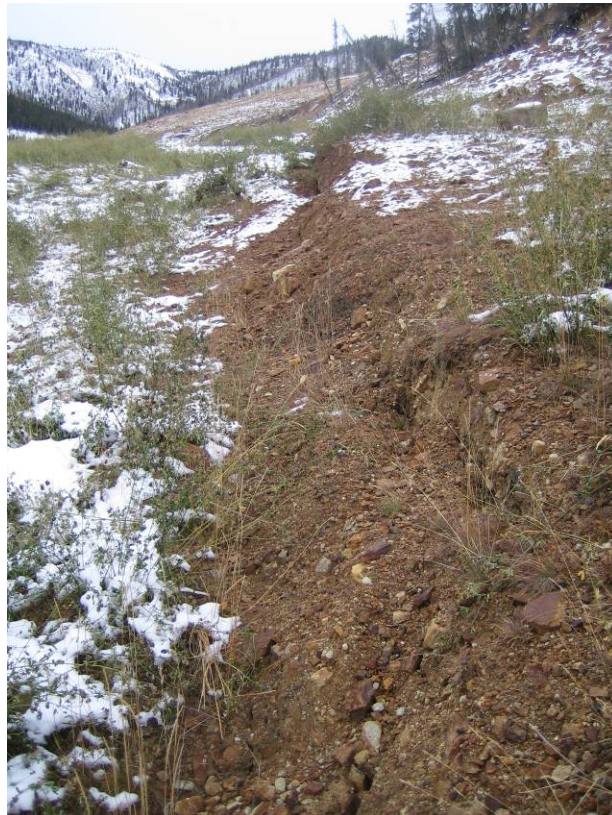
Photo 18: Second view of the scarp at the second failure location.
