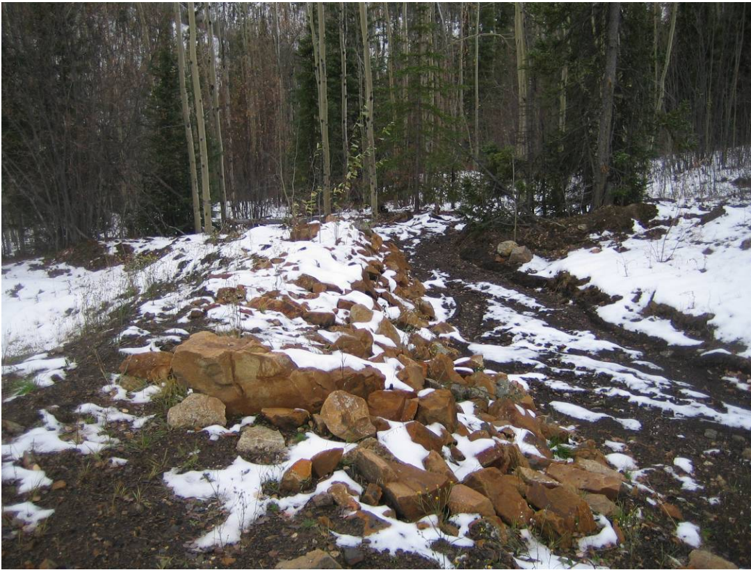
Photo 5: View of outfall looking downstream (south). Runoff is directed into the trees. No signs of erosion were visible downstream of the outfall.
