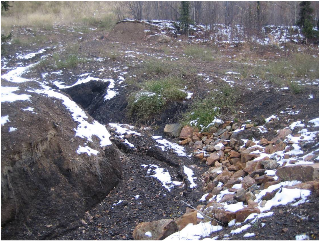
Photo 7: View of rip-rap placement on the outside bank of the surface collection ditch.
