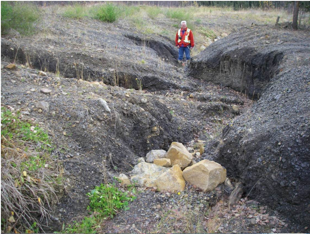
Photo 7: View of the eroded runoff collection ditch upstream of the 2 nd rip-rap location (looking downstream).
