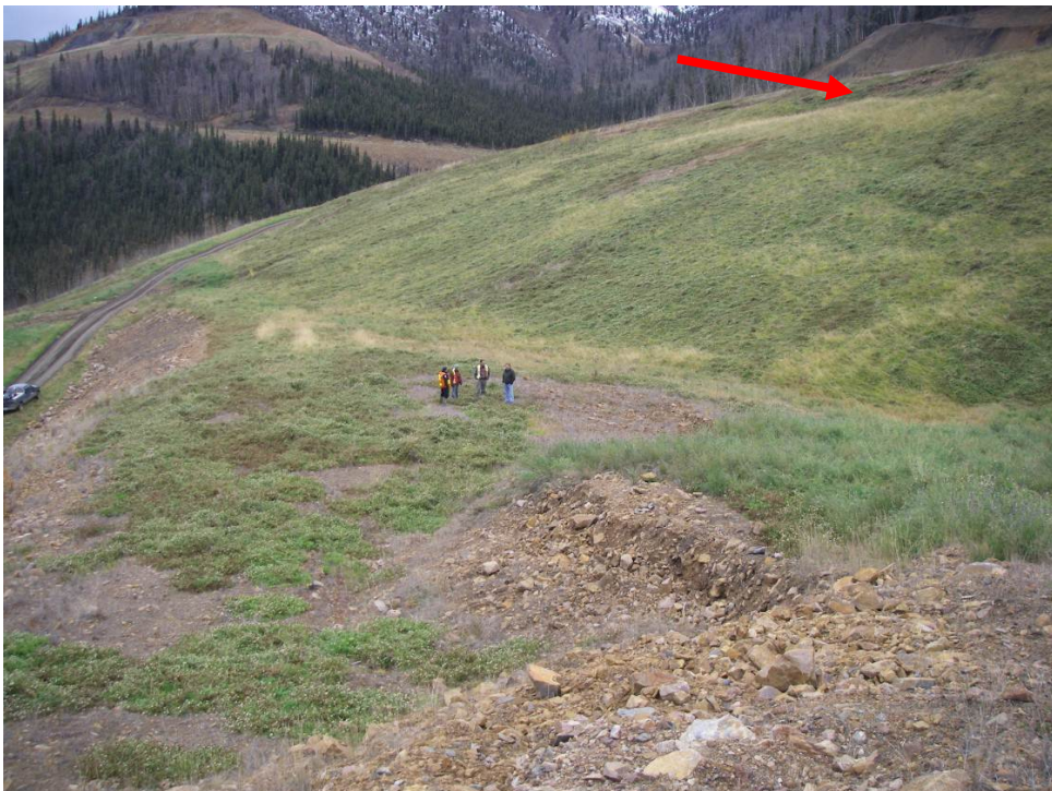
Photo 16: View from same location as Photo 15. Possible slope movement on the waste rock dump further to the west, noted by the arrow. Area was covered in snow during the 2010 inspection.
