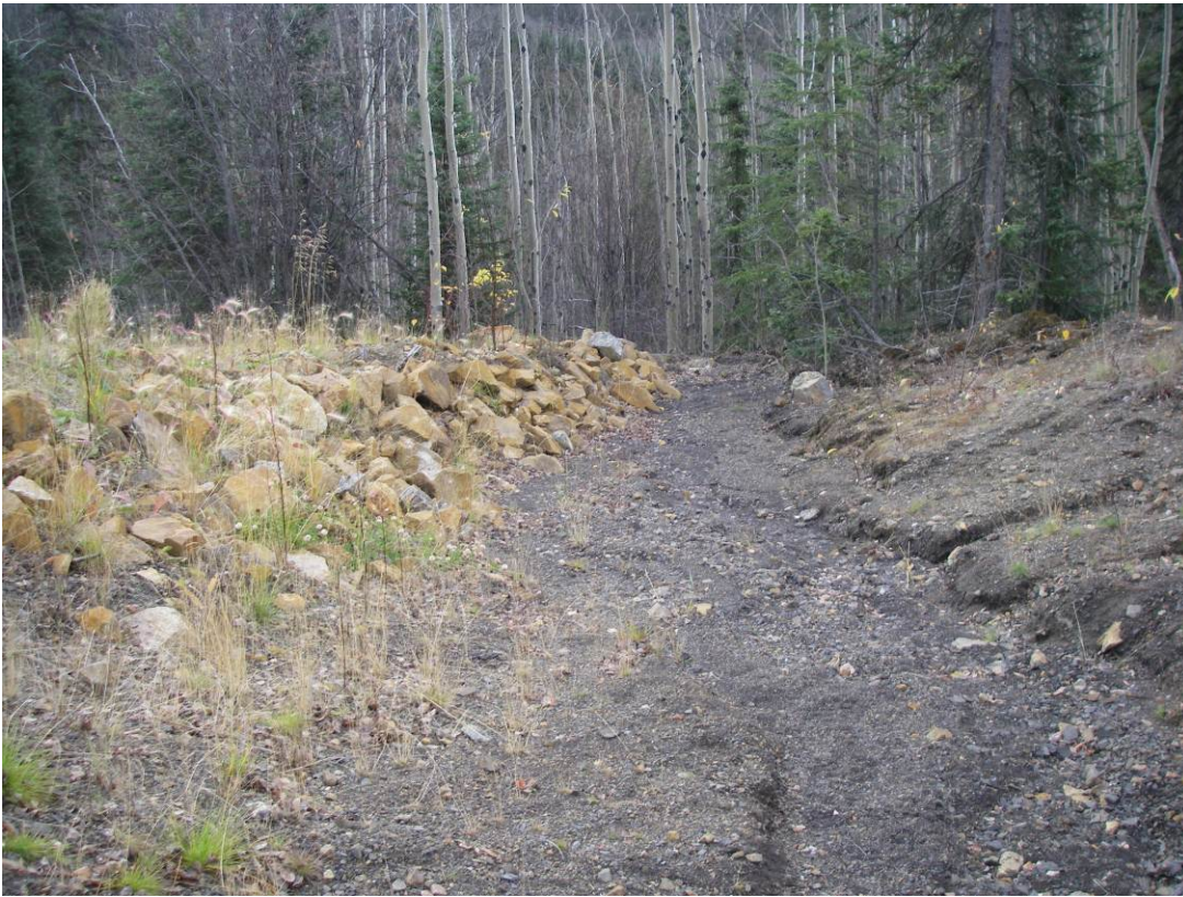
Photo 5: View of outfall looking downstream (south). Runoff is directed into the trees.
