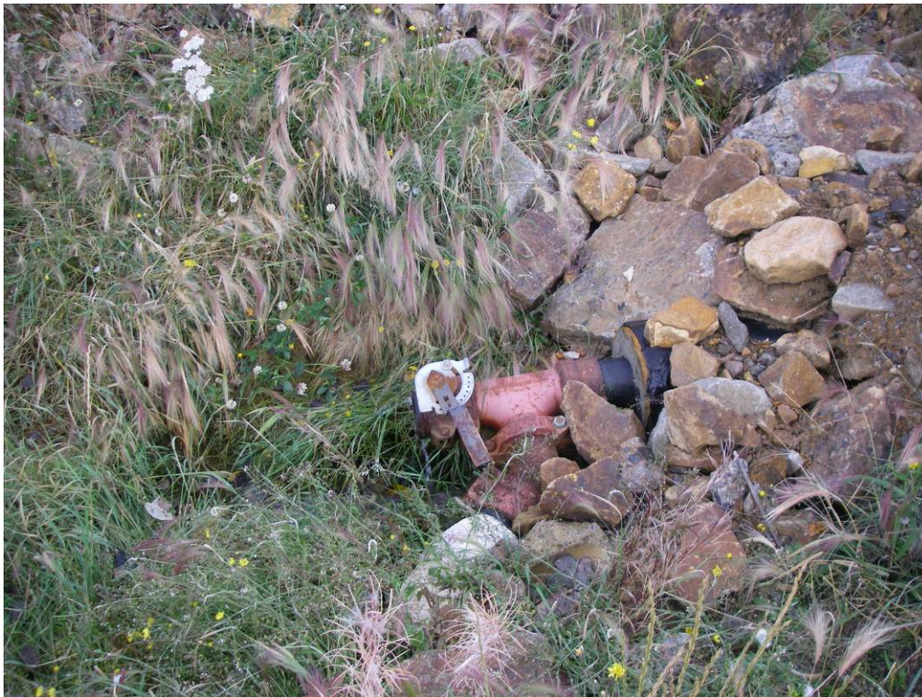
Photo 22: View of the valve controlling flow from the heap leach pad collection system to the Barren Pond. Valve is in the closed position. In the open position, water is directed into the Pregnant Pond.
