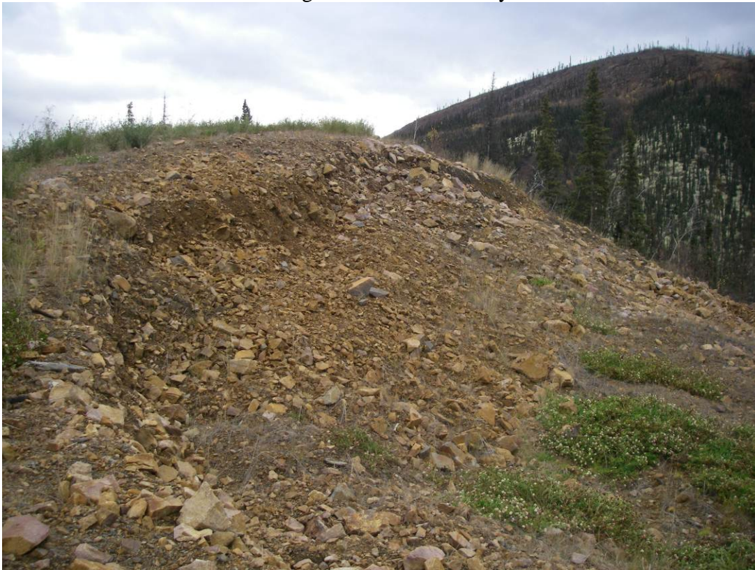
Photo 14: View of scarp in the ‘saddle area’. Looking east, settlement is orientated towards the north towards the 2 nd failure location in photos 10 to 12.
