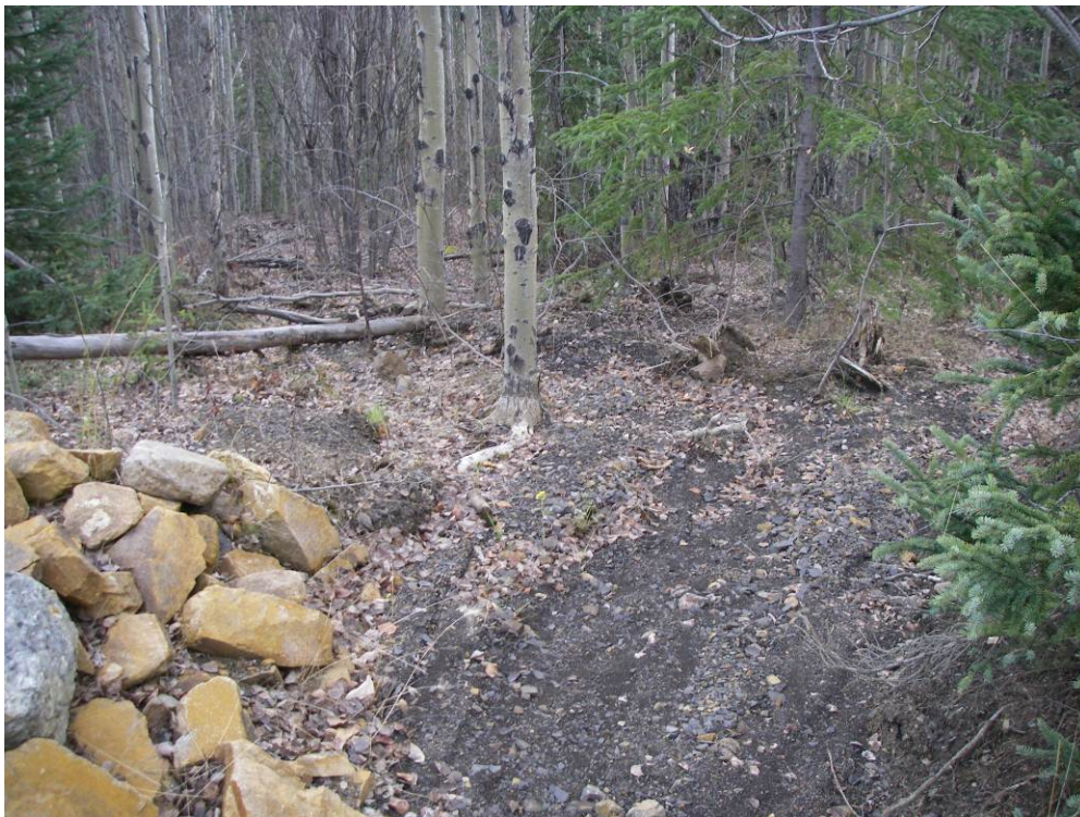
Photo 6: View of outfall looking into the trees. The deposition of eroded materials was followed for ~25m downstream of outfall. The end of the deposition zone was not found, the ground slope increased at that point from a gentle to moderate slope.
