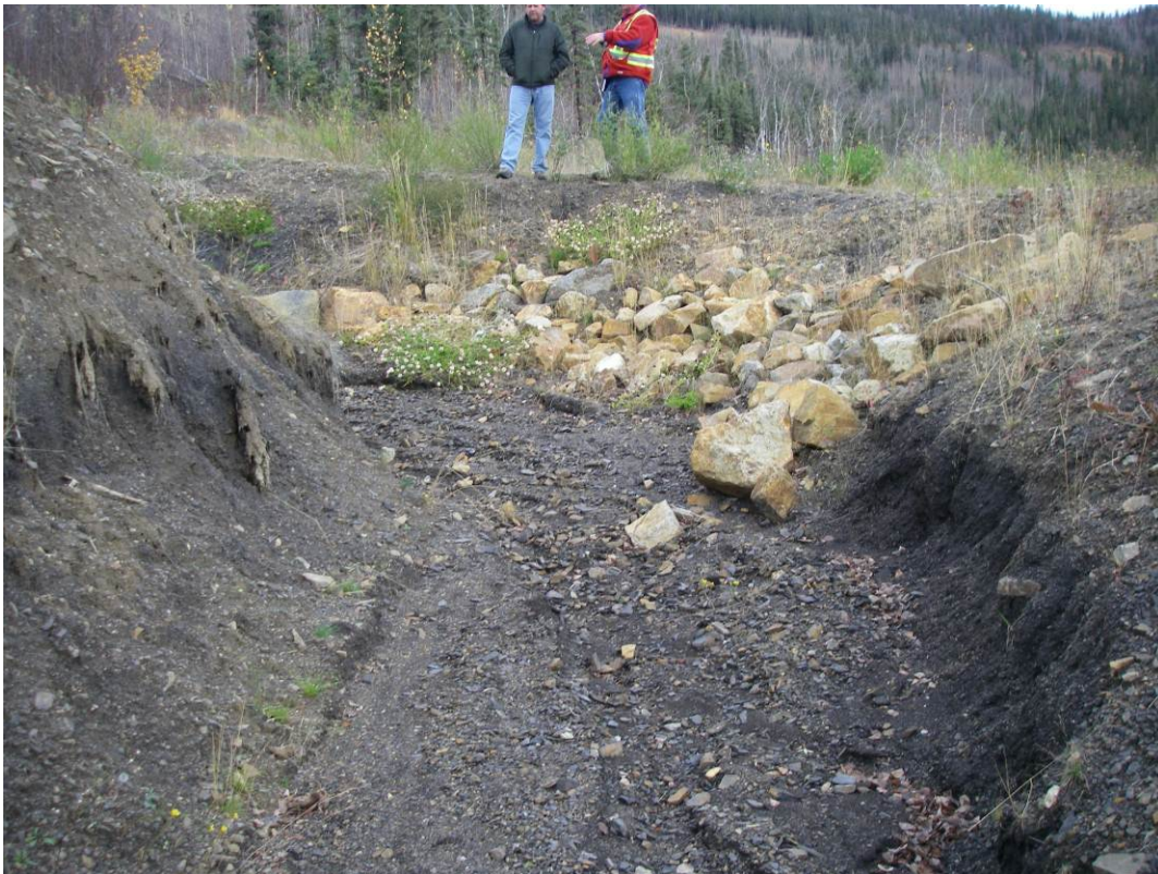
Photo 4: Rip-rap placed in 2009 near the outlet of the surface runoff collection ditch at the toe of the Blue Dump (1 of 2 locations). Compared to 2010 inspection photos, no further erosion observed.
