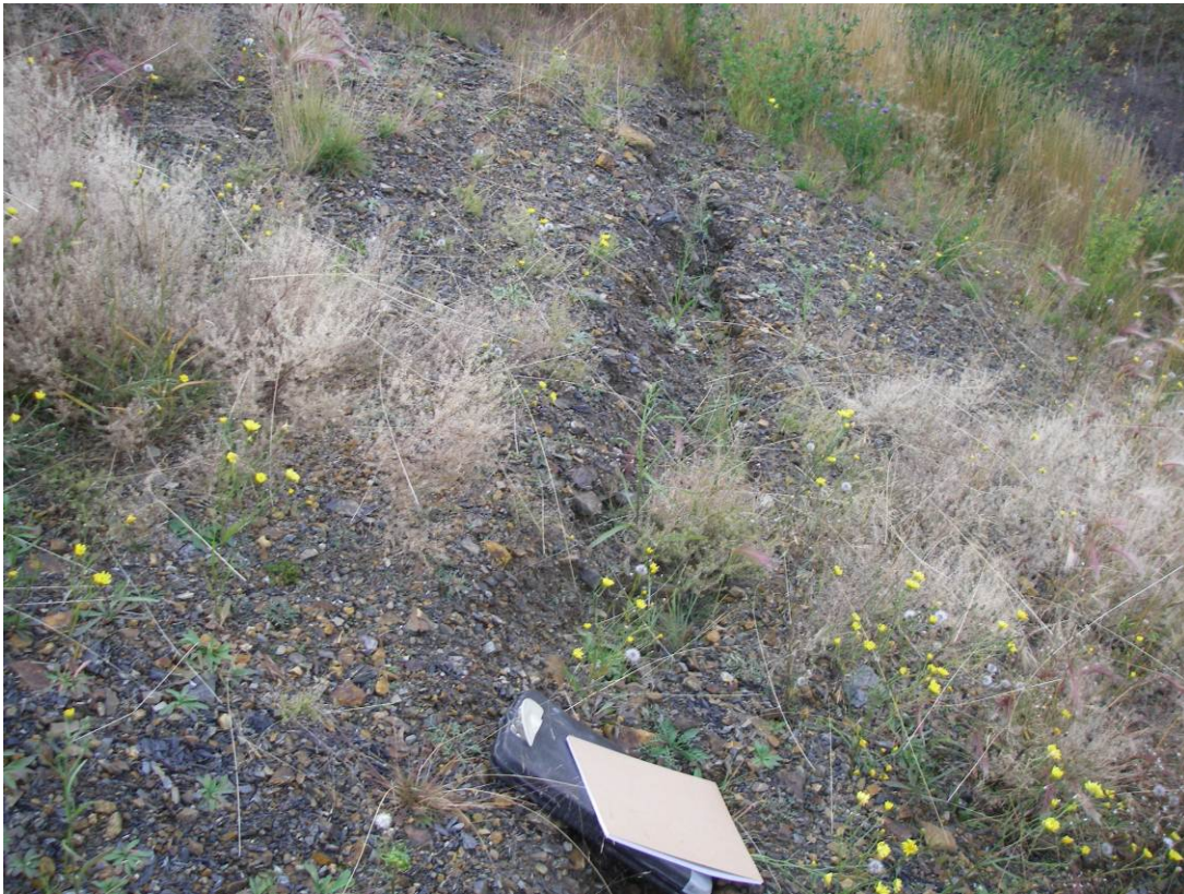
Photo 19: View of Tension cracks by the heap leach dyke near the breach location noted in the 2010 inspection. Vegetation is establishing within the crack indicating no further movement.
