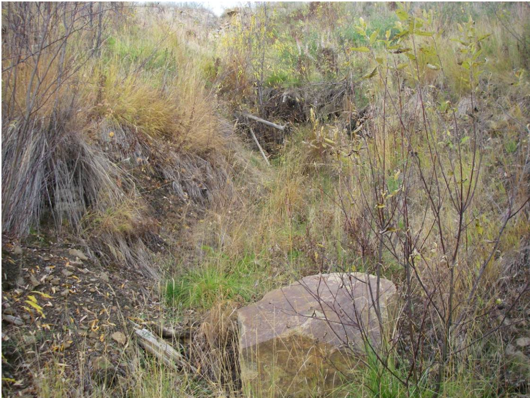
Photo 2: View of the largest gully at the toe of the Blue Dump. Vegetative growth is occurring within the rills indicating the gullies are stabilizing. No change in appearance since the 2010 inspection.
