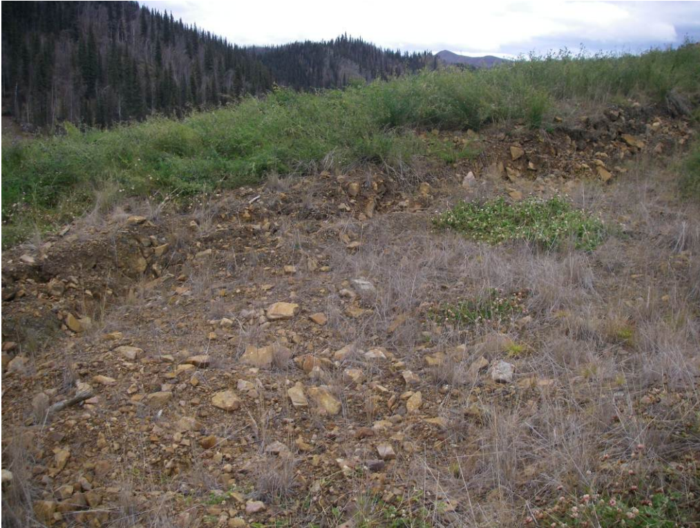
Photo 13: View of the “saddle area” of the Lucky WRSA where large differential settlements have occurred. Looking North towards Lucky Pit
