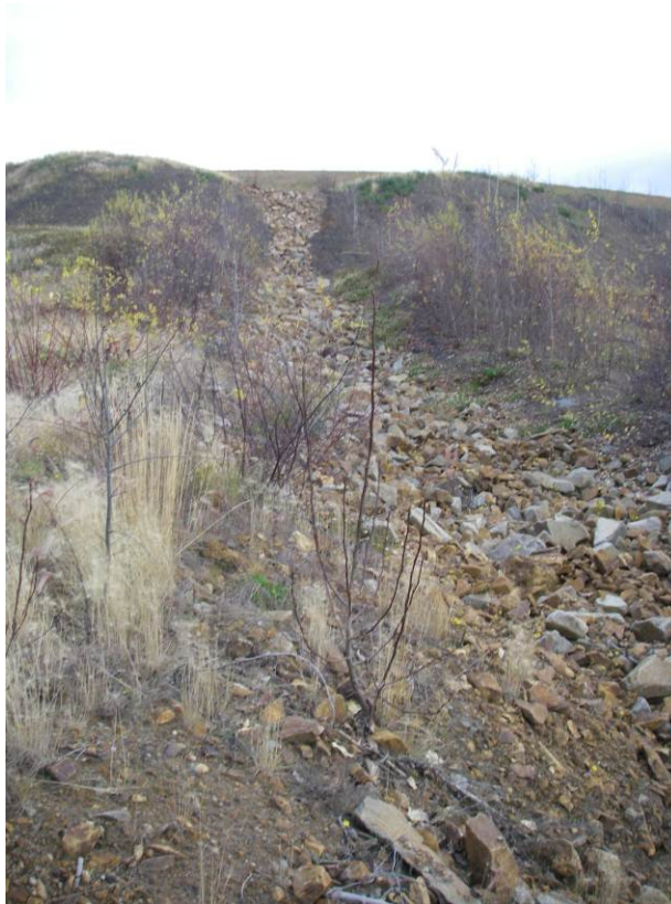
Photo 21: View of the rip-rap lined channel below the breach leading to the former Pregnant Pond.
