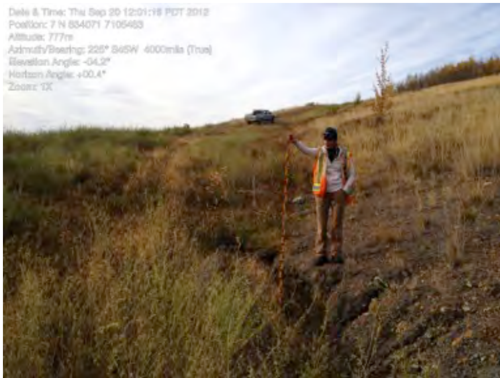
Plate 18: Erosion Channel Adjacent to Access Road at Blue Pit
