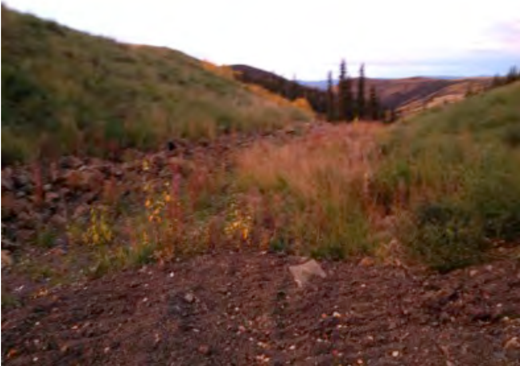
Plate 7 Haul Road Swale KP 1.8 - Repaired Washout
