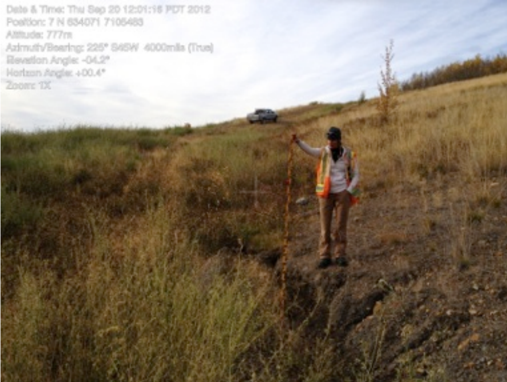
Plate 27: 2012 Erosion Channel Adjacent to Access Road at Blue Pit
