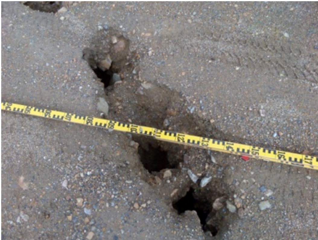
Plate 24: 2014 Haul Road Sinkhole At Pacific Pit Overflow Width 0.3m
