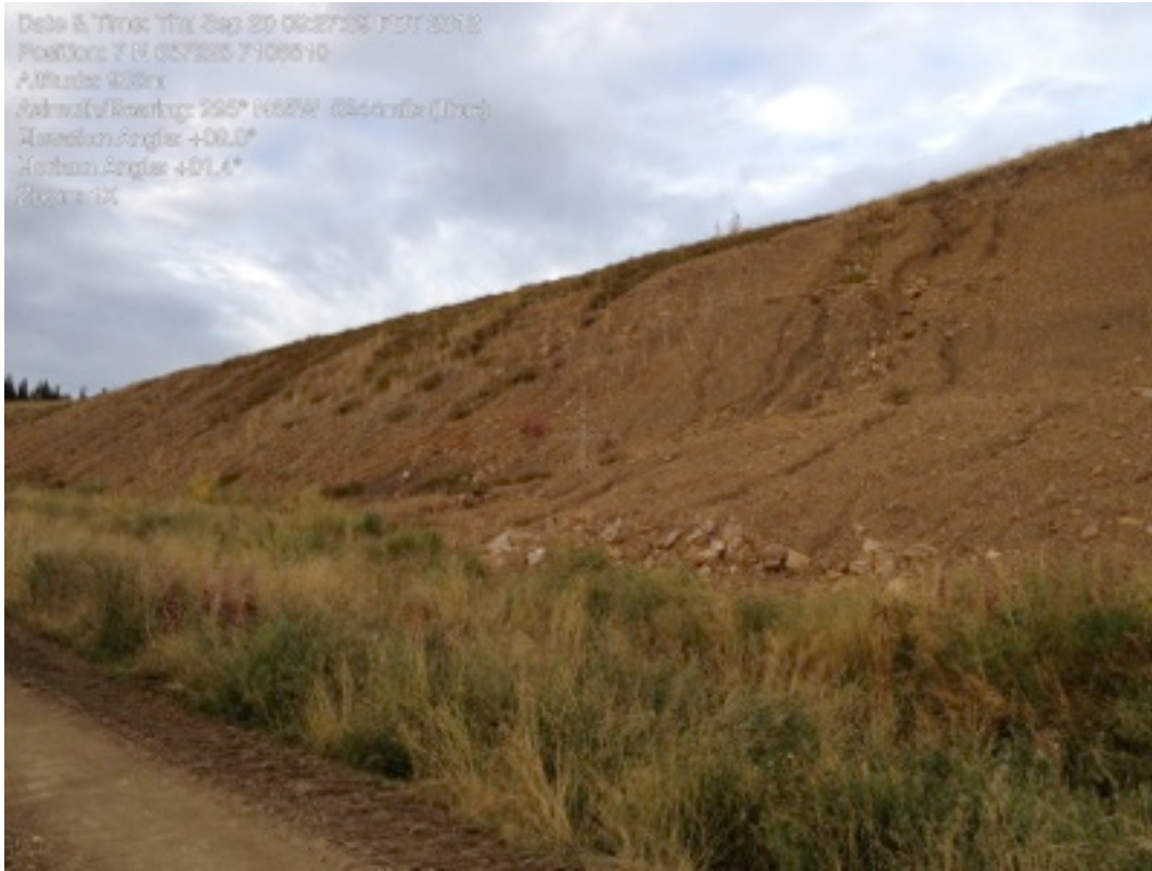
Plate 41: 2012 Erosion NW Corner North Golden Waste Dump
