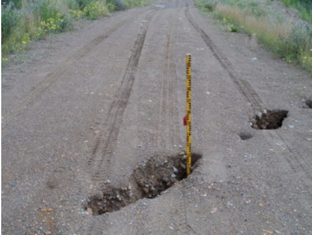
Plate 23: 2014 Haul Road Sinkhole At Pacific Pit Overflow Depth 1.2m
