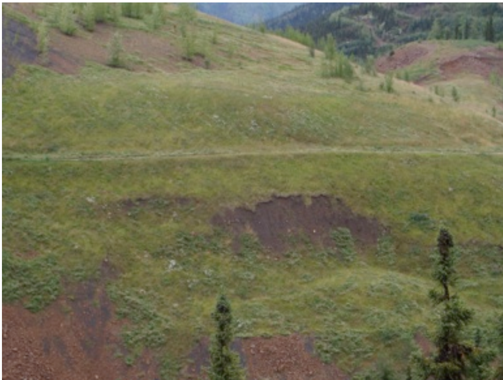
Plate 18: 2014 Road Embankment at Lucky Haul Road
