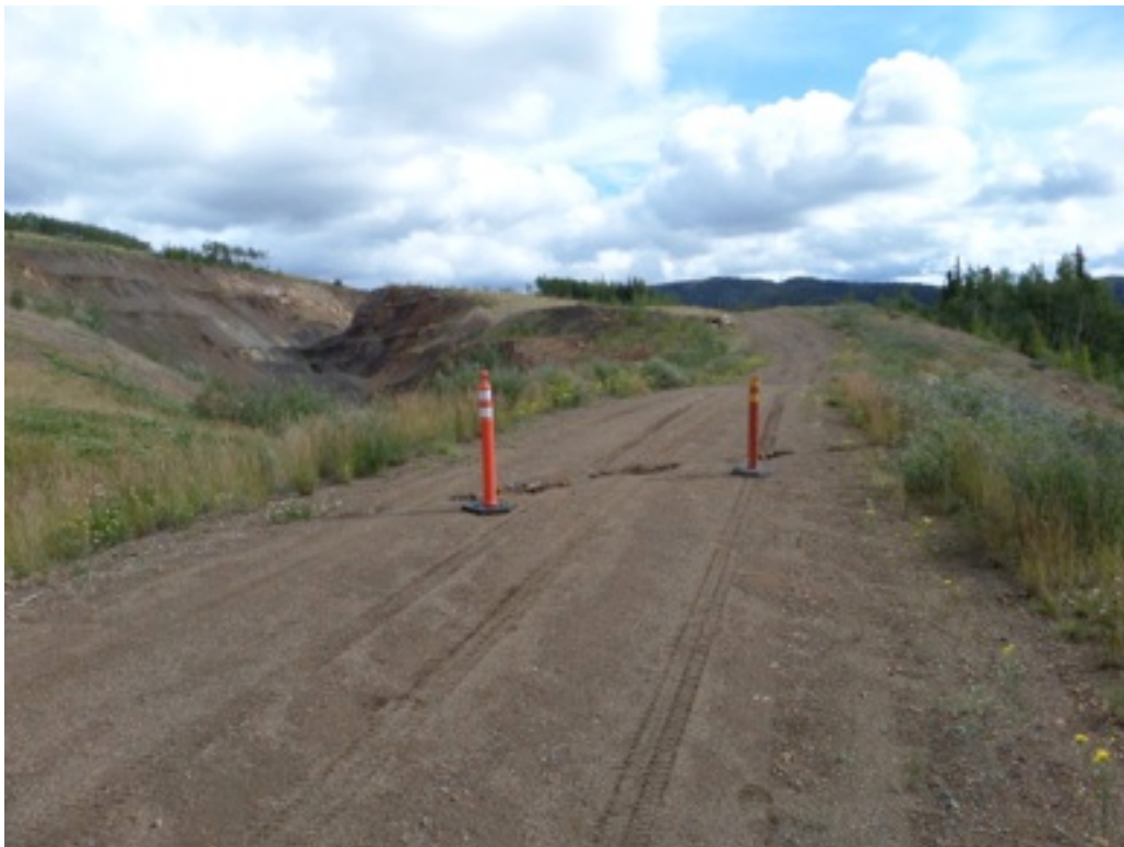
Plate 22: 2014 Sinkholes in Haul Road at Pacific Pit Overflow
