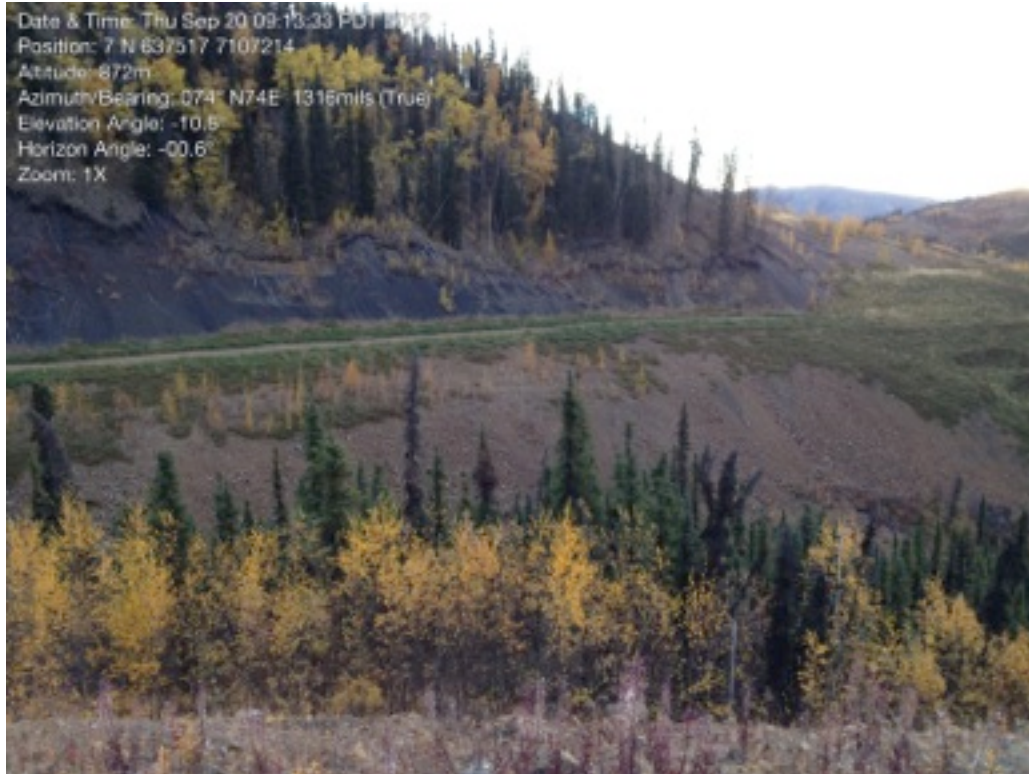
Plate 15: 2012 Road Embankment at Lucky Haul Road
