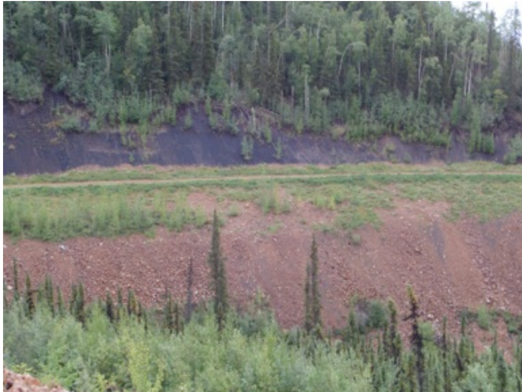
Plate 16: 2014 Road Embankment at Lucky Haul Road
