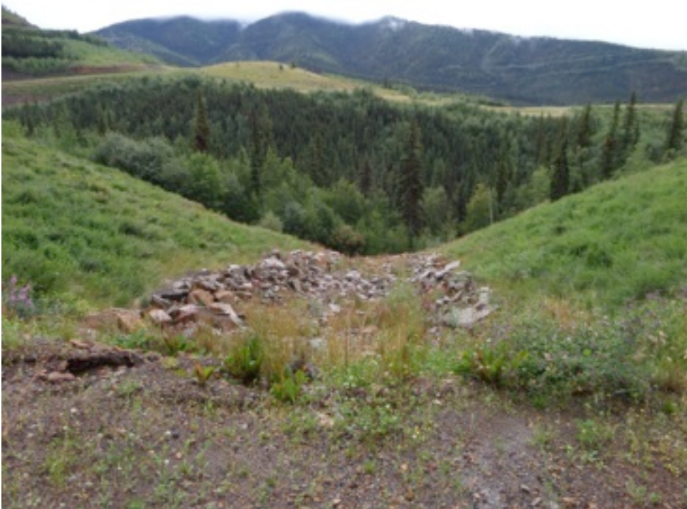
Plate 6 2014 Haul Road Swale KP 2.8 (Old Marker KP 1.2)
