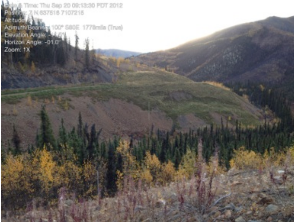
Plate 17: 2012 Road Embankment at Lucky Haul Road
