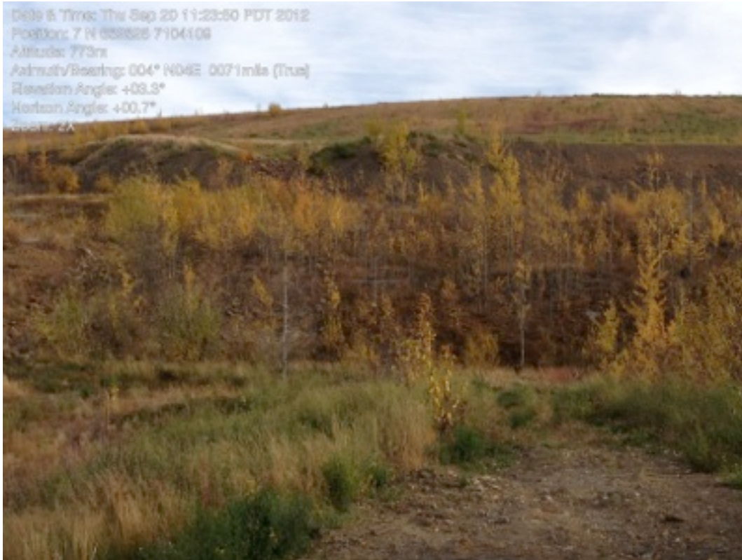
Plate 59: 2012 Breach in Heap Leach Containment Dyke above Pregnant Pond
