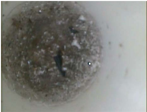
Photo 1: Blockage in monitoring well MH-12-03
