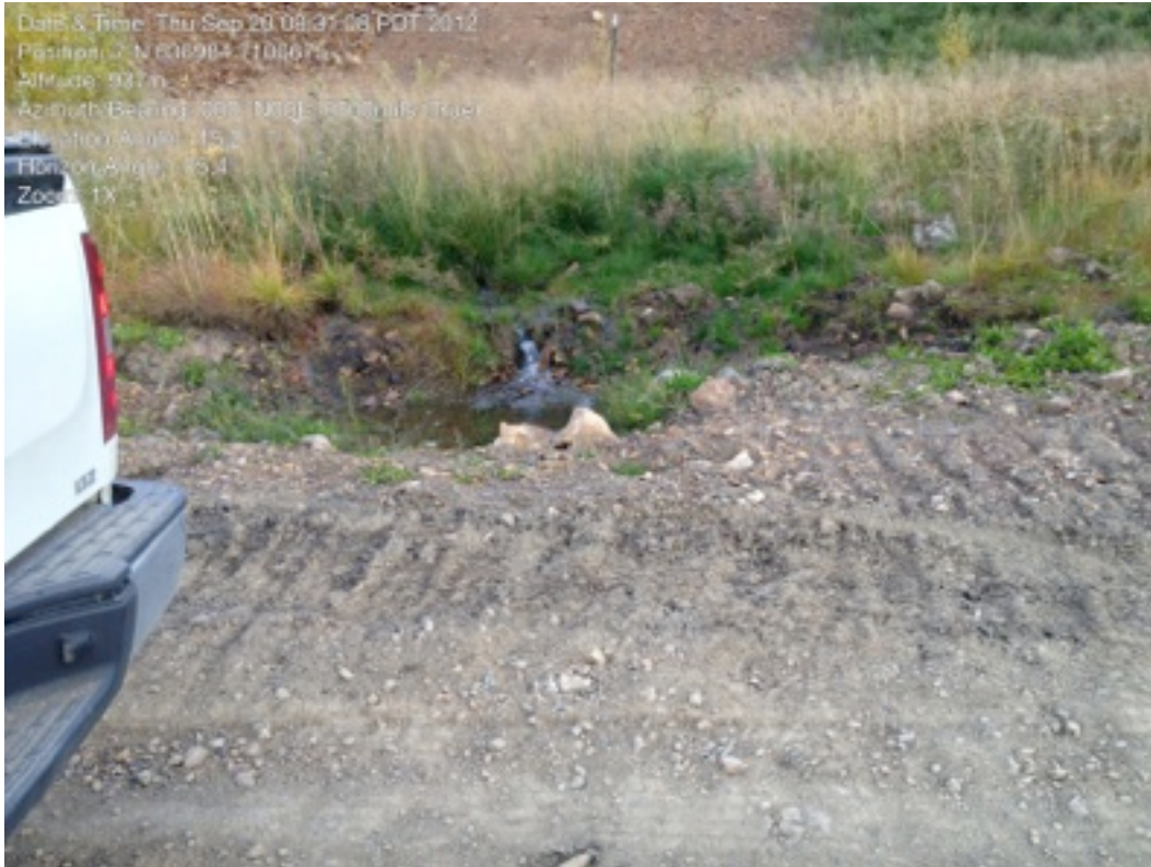
Plate 14: 2012 Haul Road Drainage KP 6.3 (Old KP 4.5) 150mm HDPE Pipe
