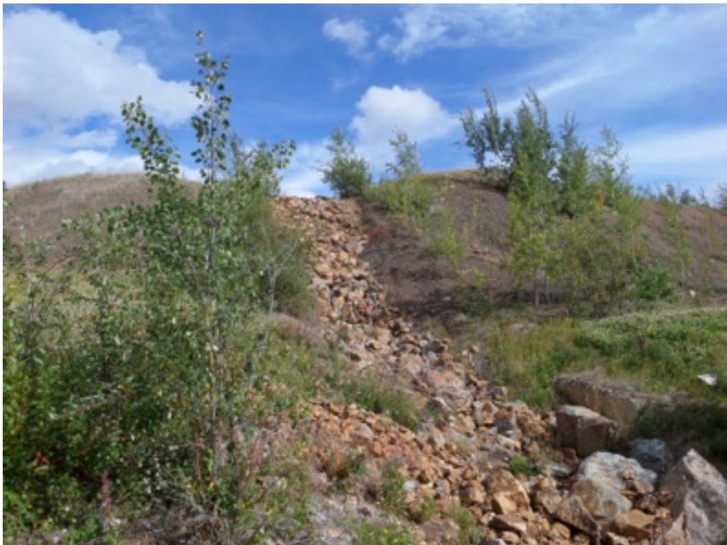
Plate 60: 2014 Breach In Dyke Erosion Protection Armour & Geotextile
