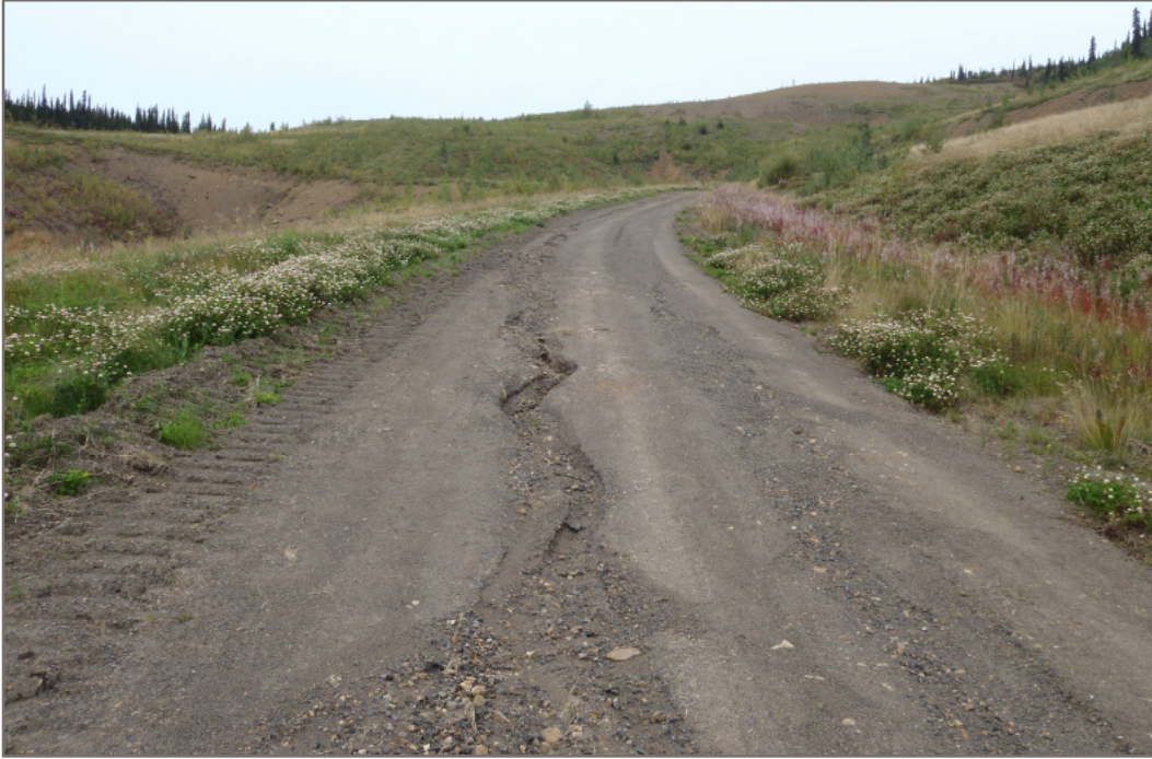
Photo 1: Primary Haul Road Surficial erosion near Golden pits Facing west — August 23, 2016
