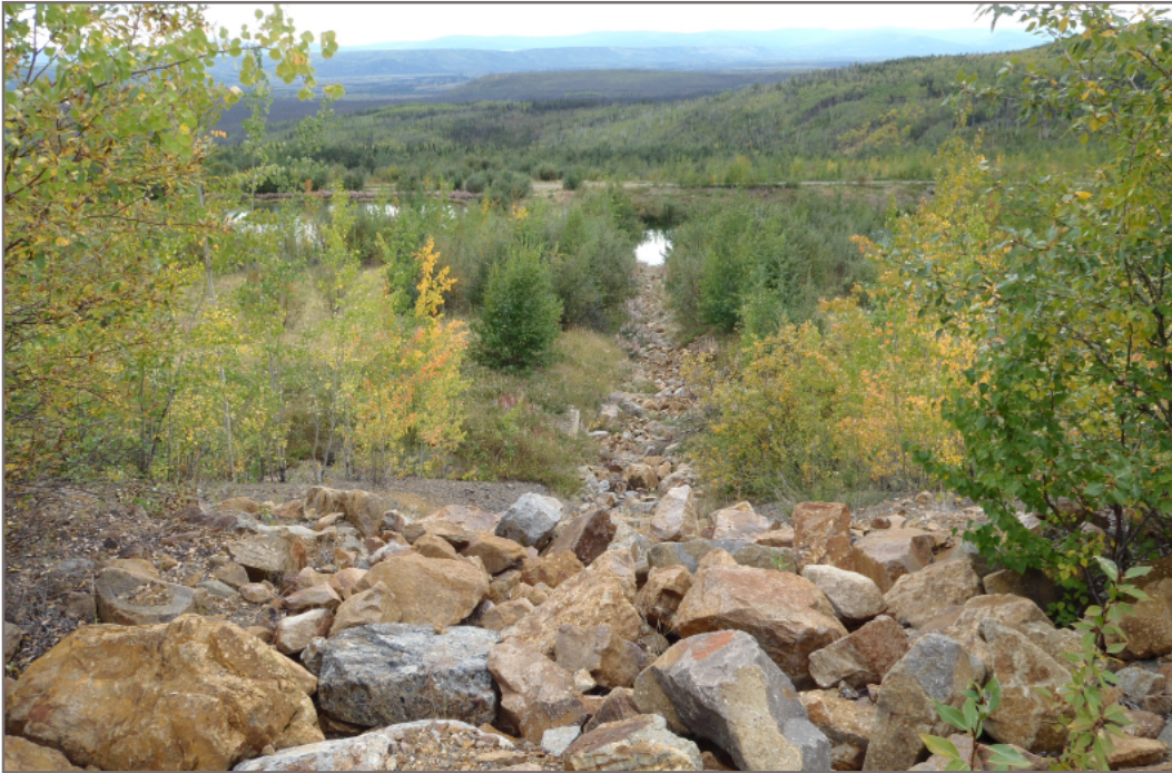
Photo 9: Containment Dyke Armoured breach channel above process ponds Facing southwest — August 23, 2016
