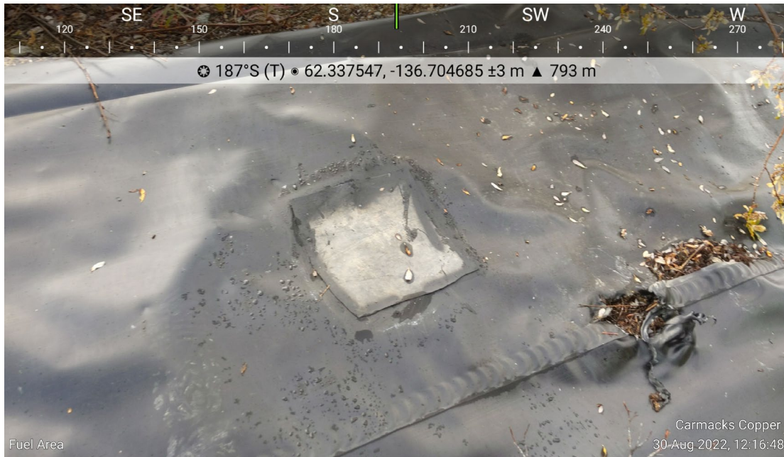
Photo 11: Patch in fuel bund liner
