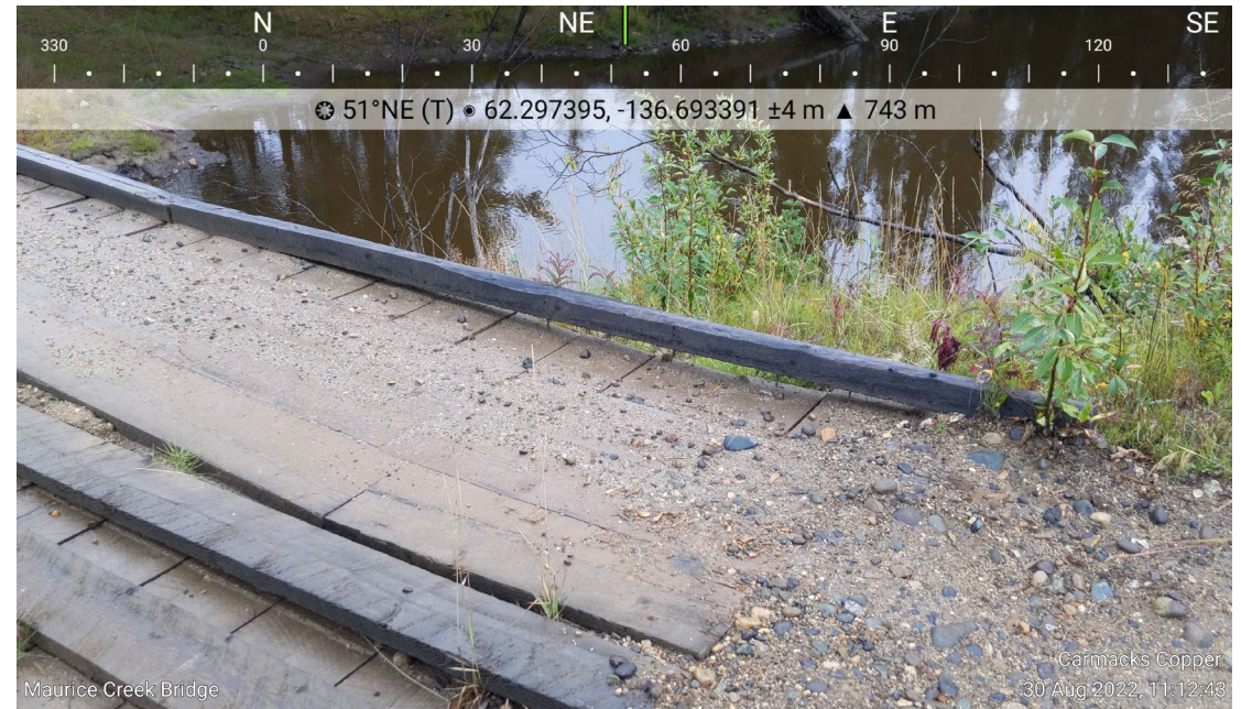
Photo 18: Damaged bridge rail – rail should be reattached to the bridge deck
