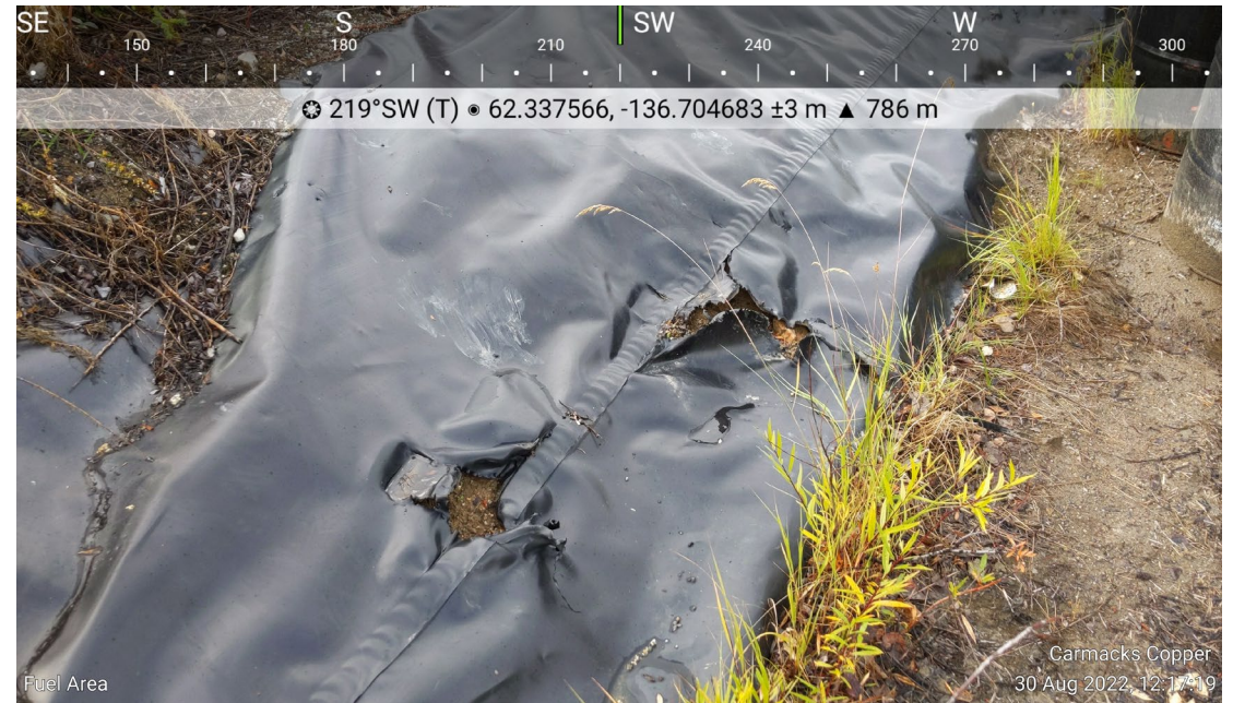
Photo 12: Hole in fuel bund liner
