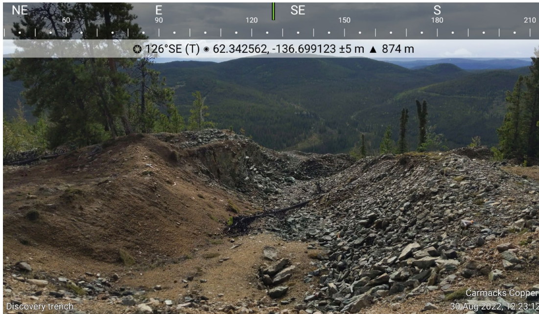
Photo 3: Discovery trench – sides of trench are sloped, trench is in satisfactory condition
