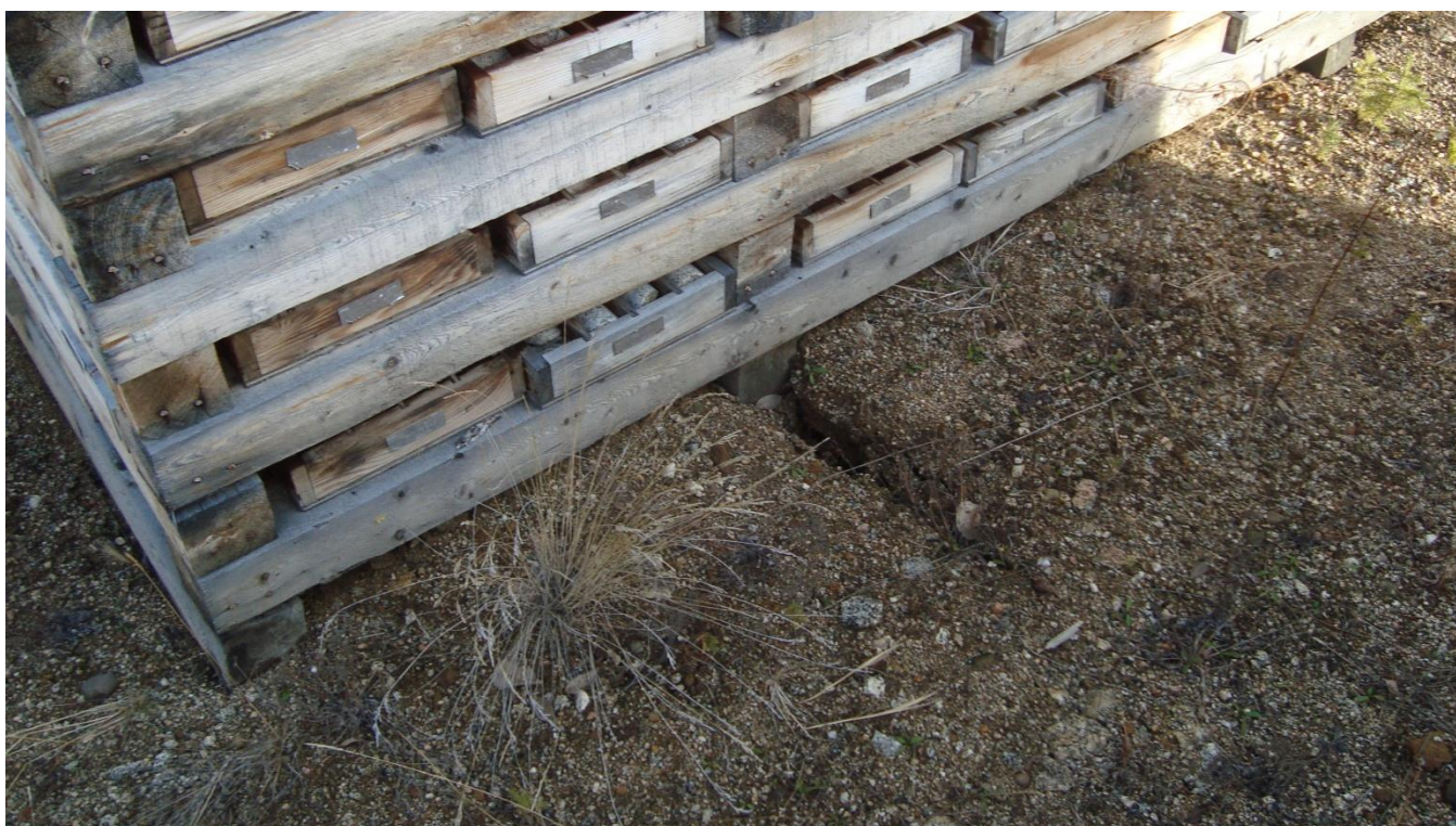
Photograph 4: Cracking in pad at southwest core rack area
