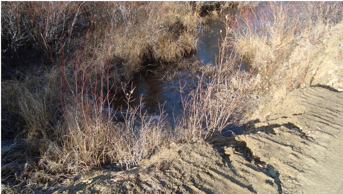
Photograph 15: View looking north of ponded water and erosion above culvert on access road at North Williams Creek
