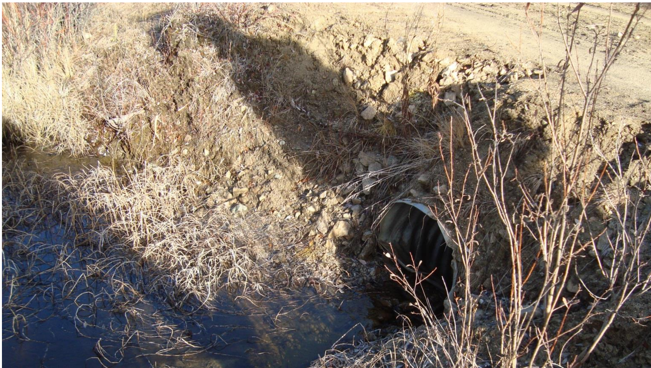
Photograph 16: View looking east of erosion above culvert on access road at North Williams Creek
