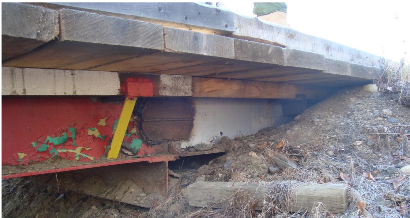
Photograph 20: Site access road crossing Merrice Creek, view of extension and bridge abutment nearest to Carmacks
