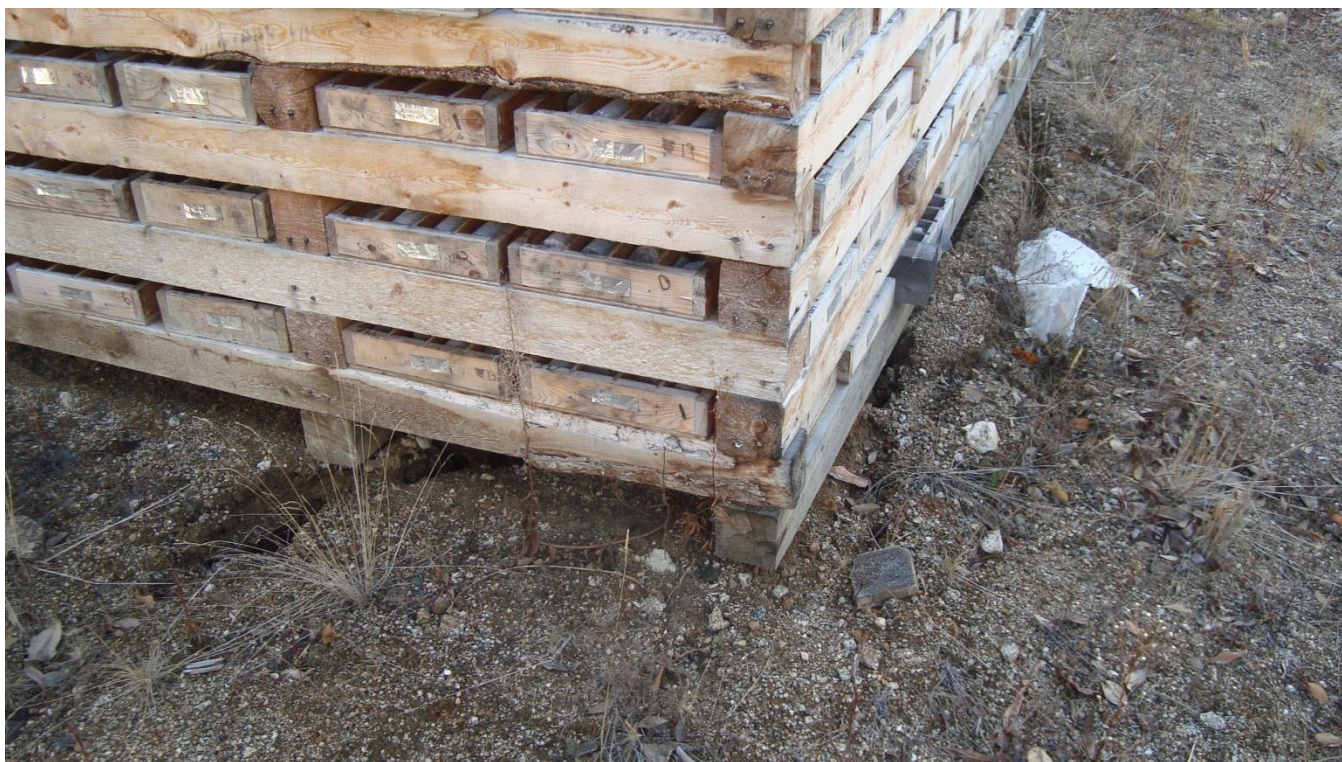
Photograph 3: Cracking in pad at southwest core rack area
