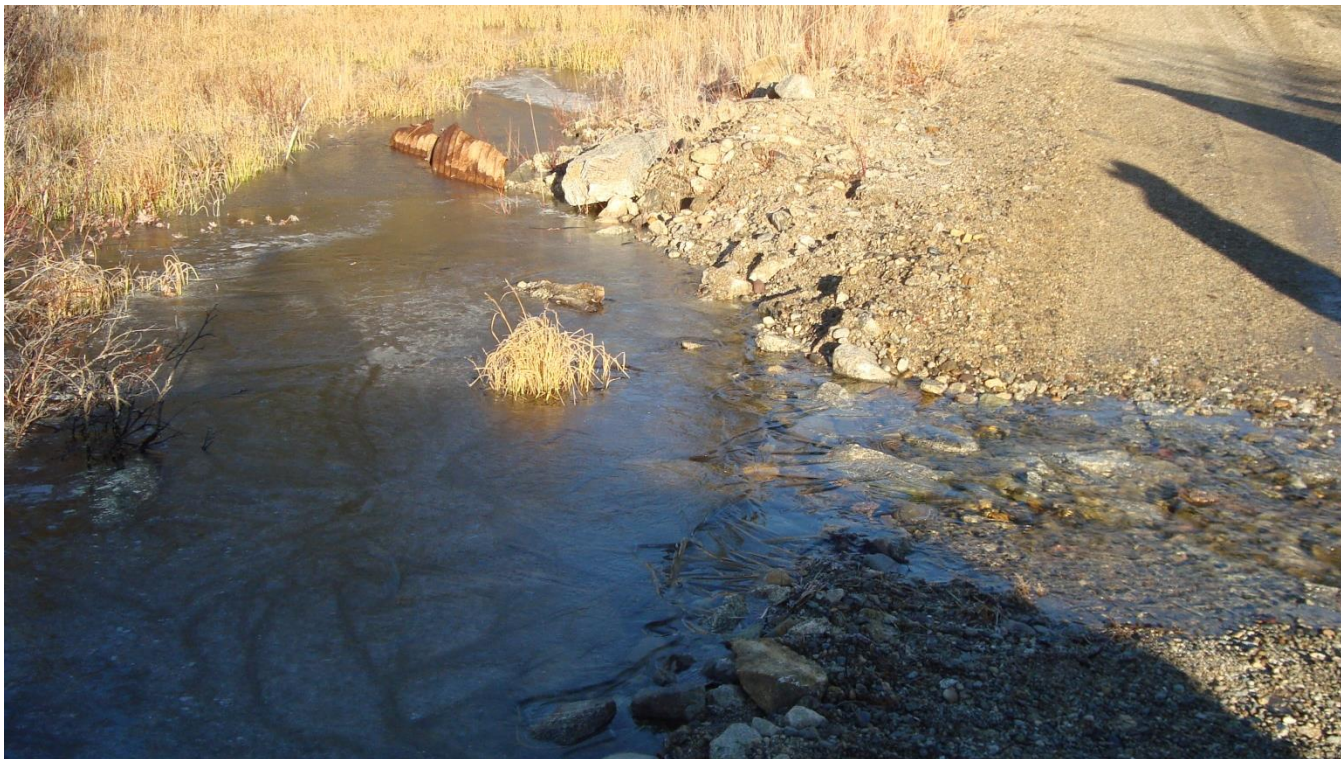
Photograph 18: View looking north of ponded water behind 'ford' on access road at Williams Creek crossing
