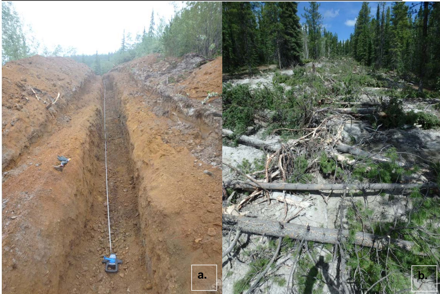
Figure 2. Typical trench conditions before (a. Trench TR-15-32A) and after (b. Trench TR16-26) reclamation.
