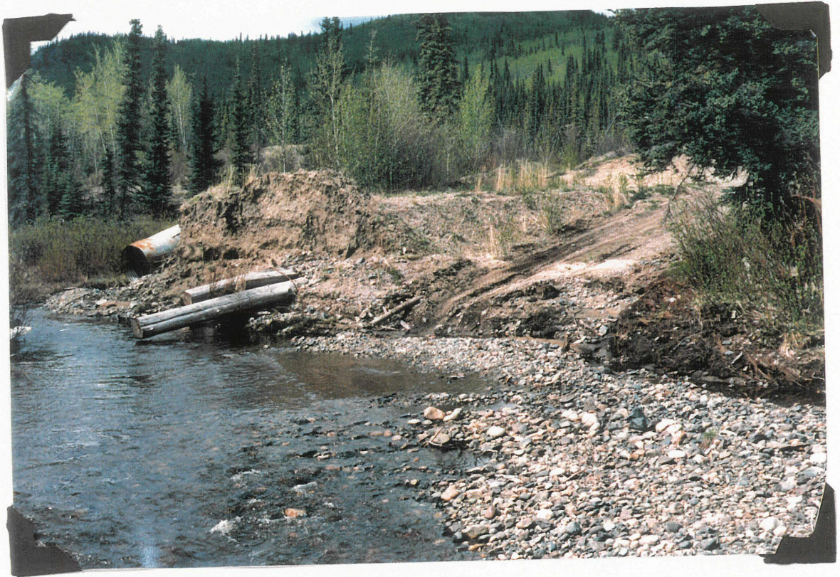
May 30, 1994. Merrice Creek road crossing - minor erosion to north bank
