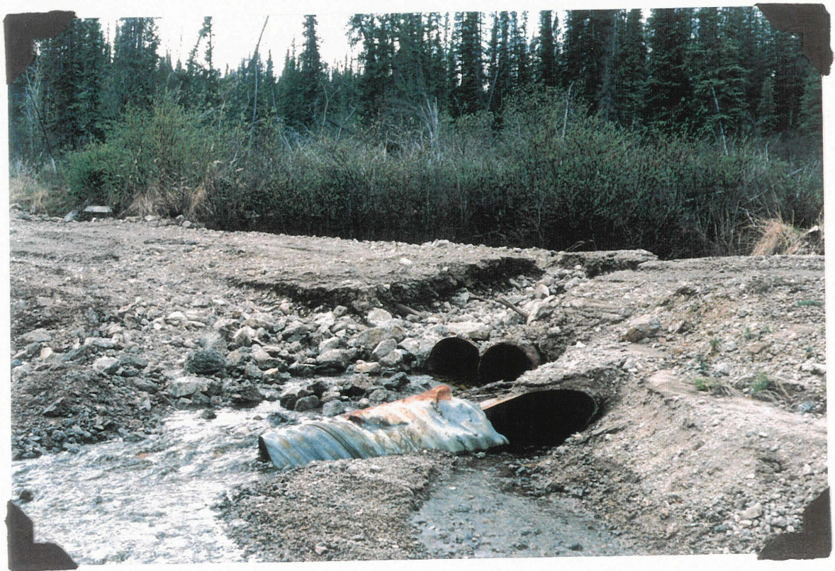
May 30, 1994. Williams Creek road crossing - minor erosion to road bed during freshet.
