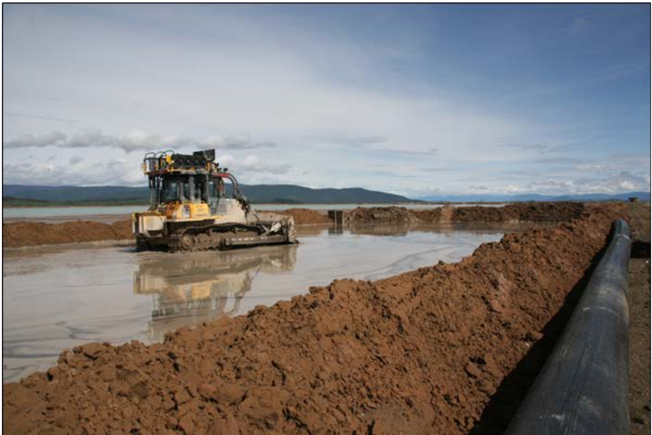
Figure A.4.9-2 Typical sand cell construction showing cyclone underflow contained by berms and compacted by dozer.
