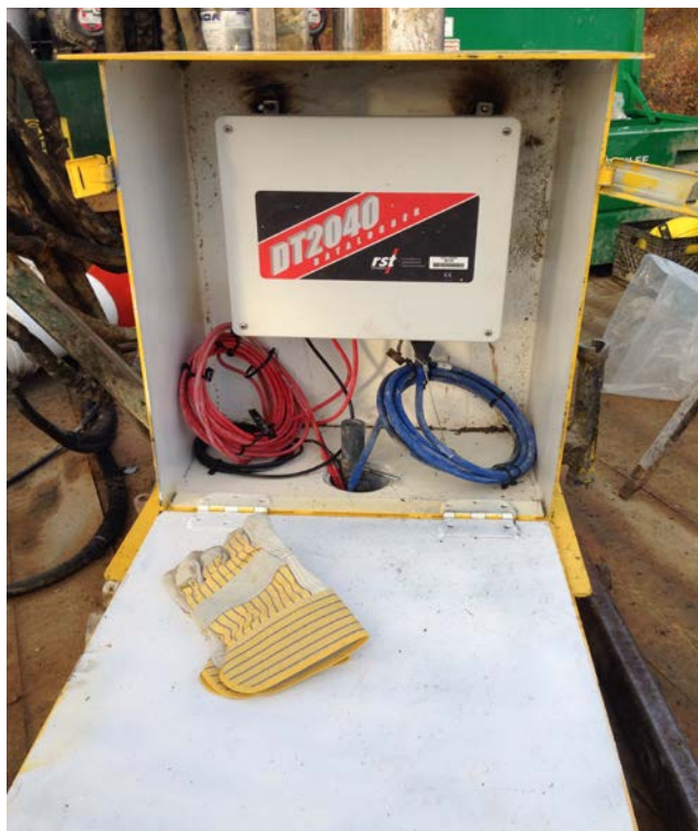
Figure 3: Datalogger and Steel Enclosure at MW16-01T.
