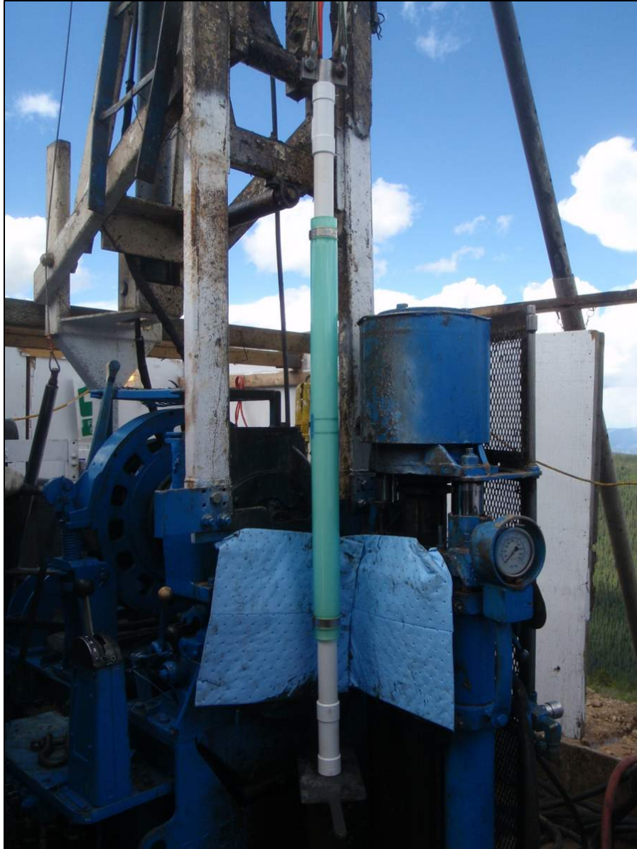
Figure 3-4: Westbay installation at MW15-06T (BH5) using the Boyles 37 diamond drill rig. Blue gland is packer element which is inflated downhole with a 3:1 dilution of propylene glycol. PVC is 1.5" Sched 80 with ends machined to mate with Westbay System couplings incorporating a shear-rod connection and an o-ring seal (no glue).
