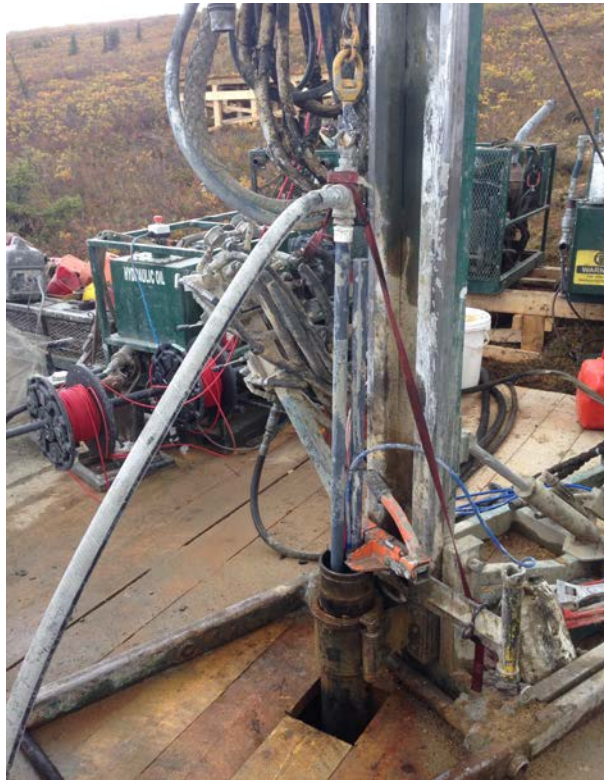
Figure 2: Grouting of MW16-01T Through 1" PVC Tremie. Both Tremie lines visible, with active pumping into the second line
