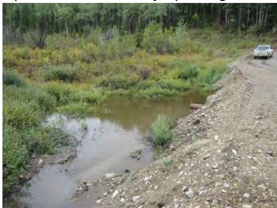
Upstream view with major ponding
