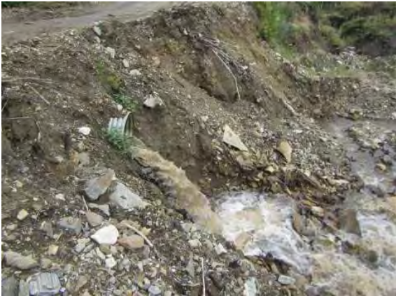
Perched culvert drop
