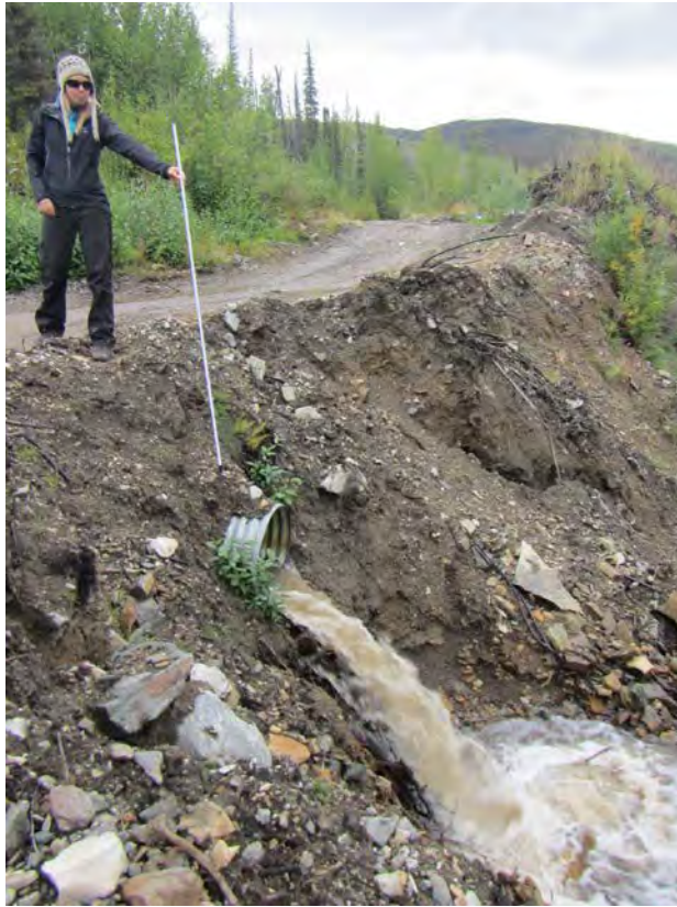
Photo 3 – Perched culvert crossing (#75) on side channel of Maisy May Creek.
