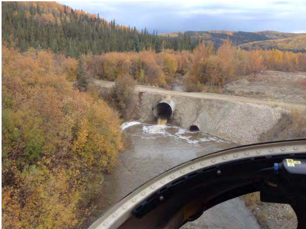
Photo 1 – Road crossing (#48) at Sulphur Creek on September 9, 2015. Showing hanging culvert and smaller overflow culvert.
