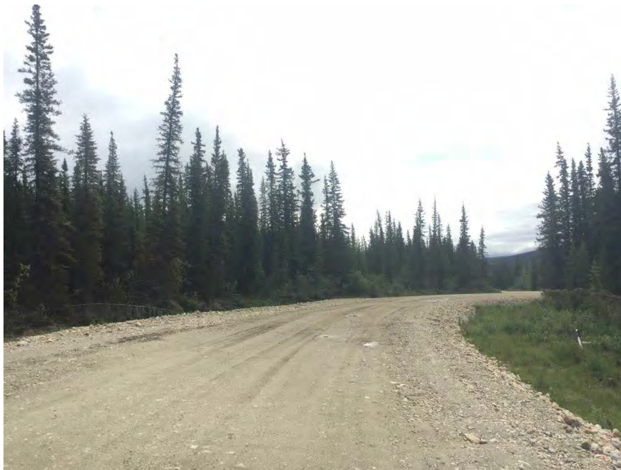
Figure 2 Photo of Existing Road on the Sulphur Section Typical of the Minor Upgrade Category
