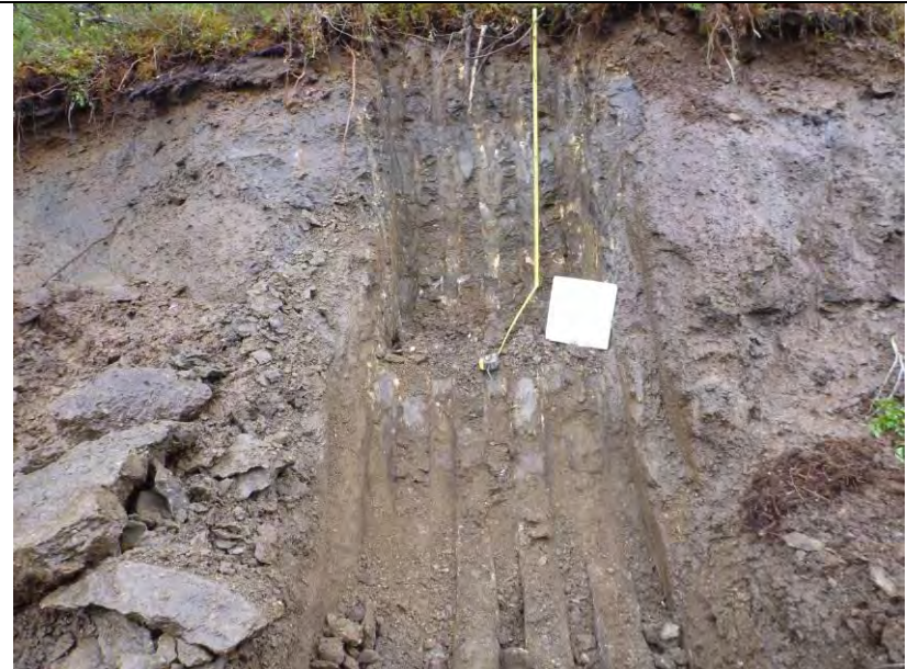
TP-BGC11-60 – Cut slope and test pit; pit completed at depth of 2.7 m.
