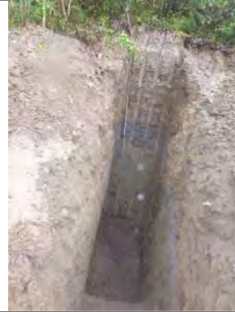
TP-BGC11-136 – Back wall of test pit; pit completed at a depth of 4.8 m.
