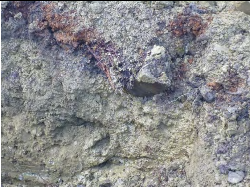
TP-BGC11-116 – Detail of seepage in pit wall.
