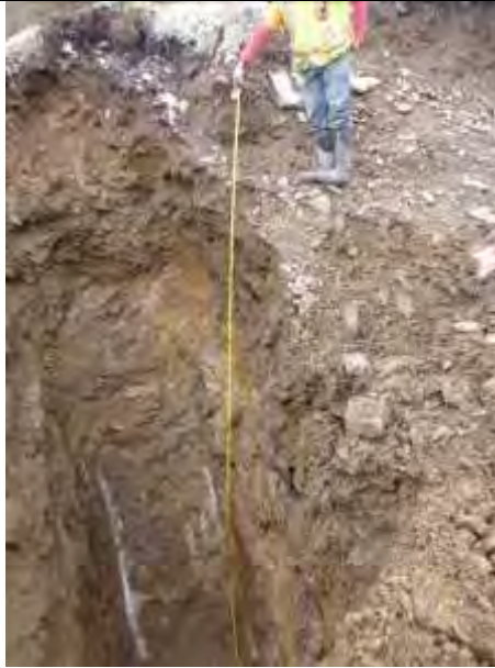
TP-BGC11-138 – Back wall of test pit; pit completed at a depth of 6.3 m.
