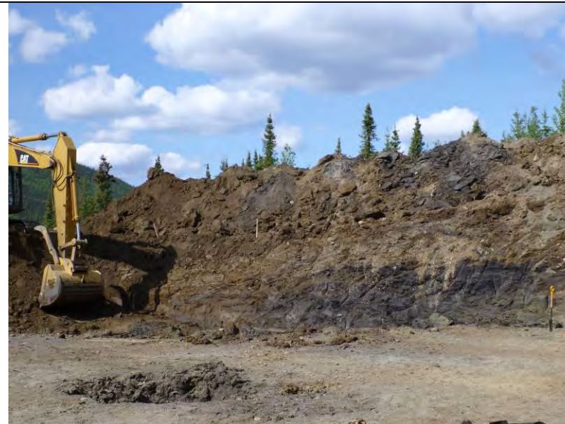
TP-BGC11-82 – Site photo; East wall.
