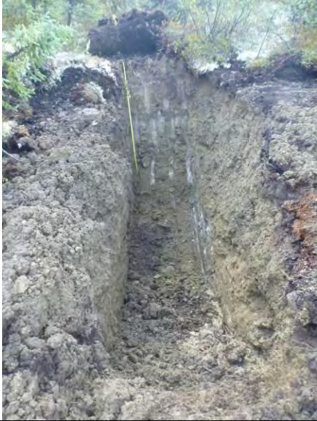
TP-BGC11-116 – Back wall of test pit; pit completed at a depth of 2.3 m.
