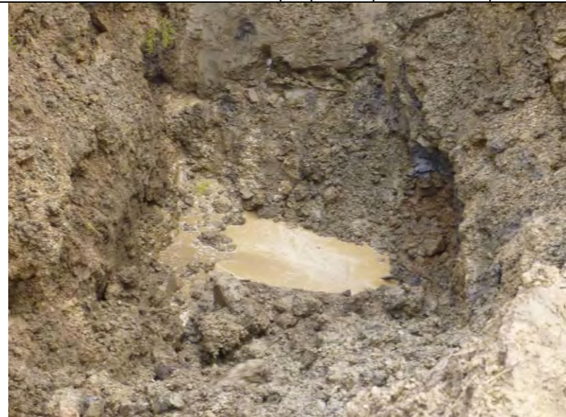
TP-BGC11-113 – Detail of seepage collecting in pit below 1.5 m.
