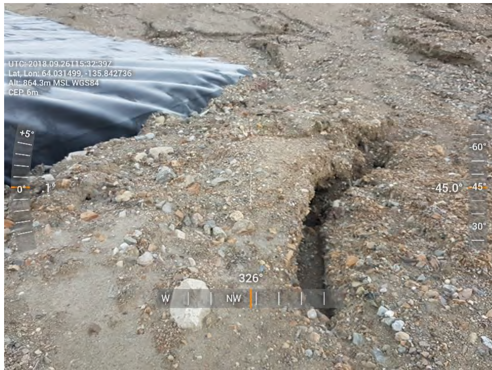
Figure 4: LDPS - Erosion at liner.
