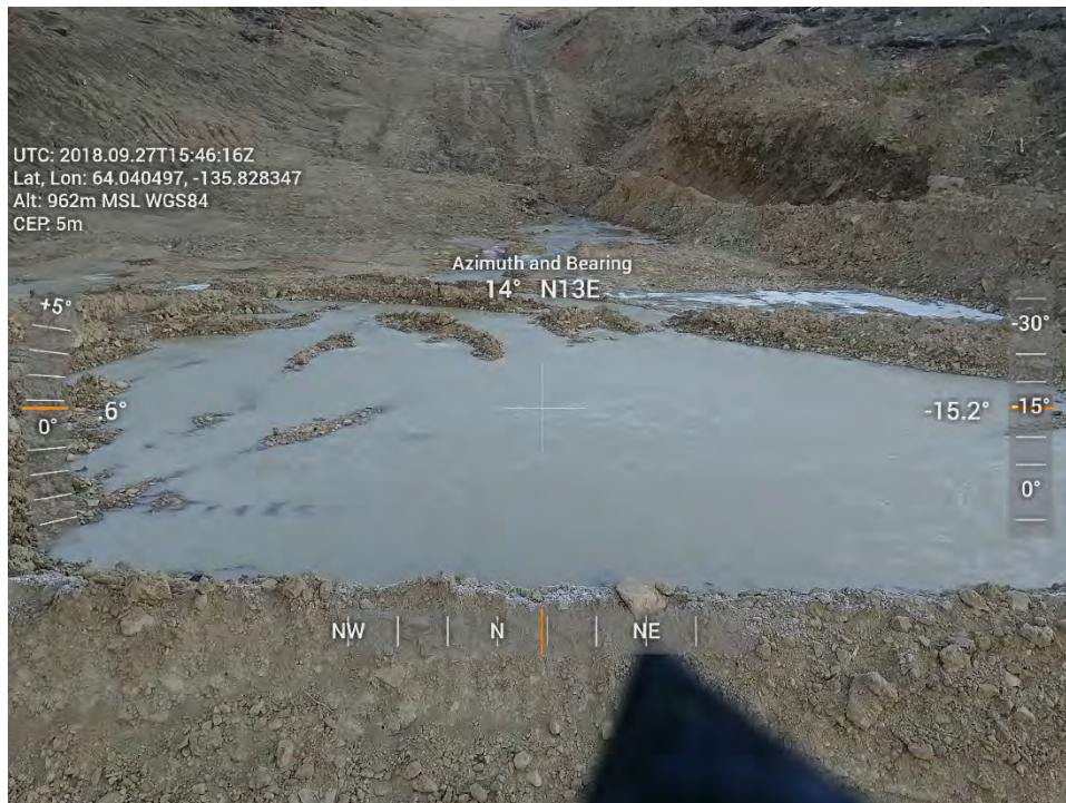
Figure 35: HLF - Pooling above collection ditch.
