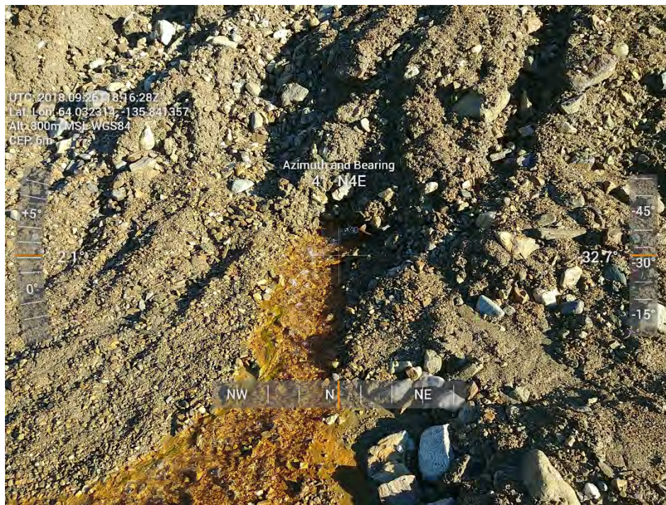
Figure 5: LDSP – Water flow from damaged culvert on northeast corner of pond.
