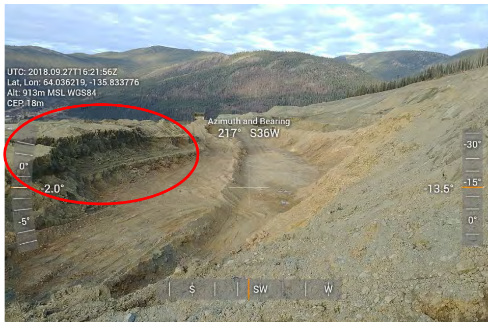
Figure 40: Event pond (facing west) – over steepened material.
