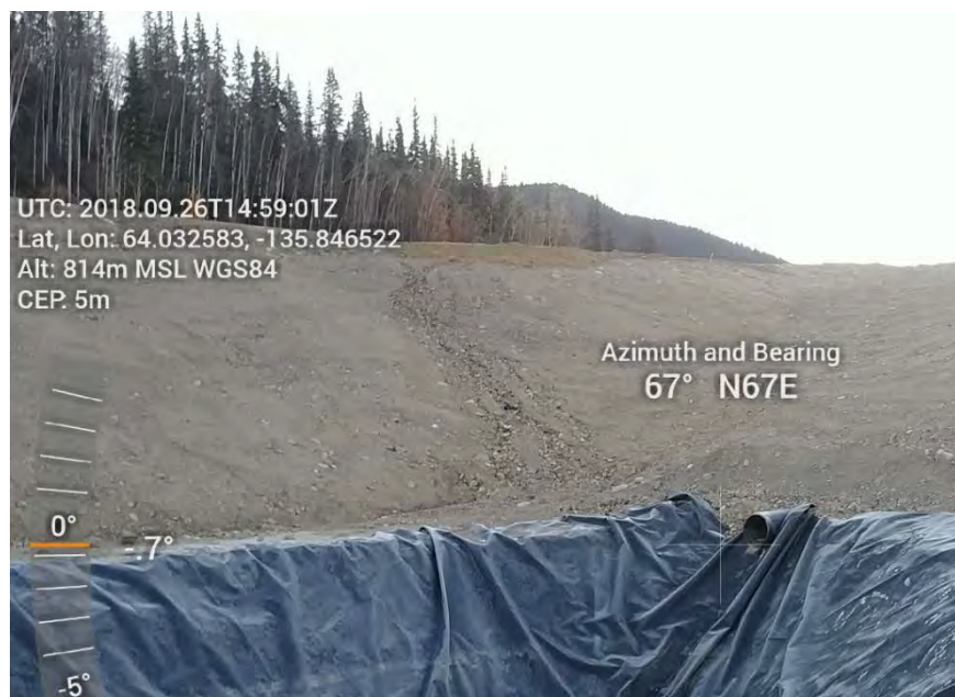
Figure 8: LDSP - Erosion at low level outlet pond.
