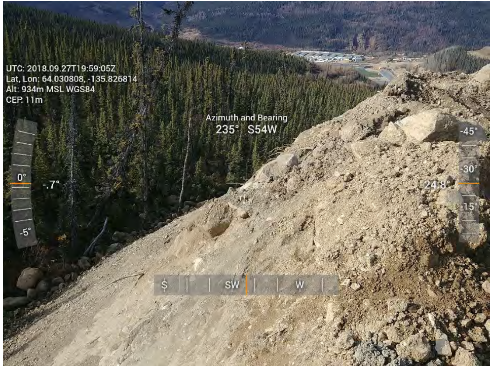
Figure 45: Stockpile B - Toe of slope encroaching on organics.
