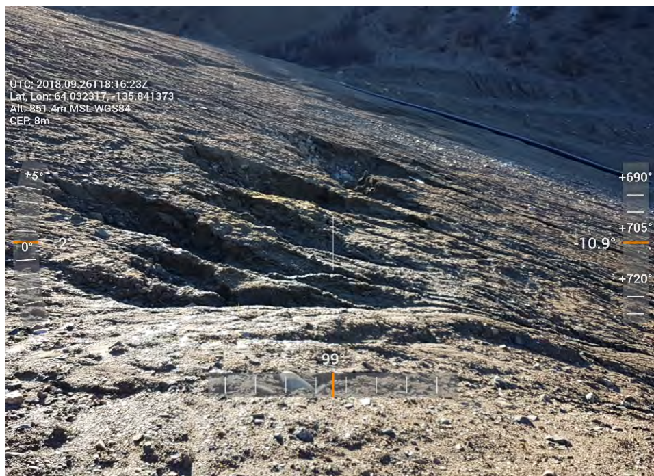
Figure 6: LDSP - Erosion on west slope of fore bay.
