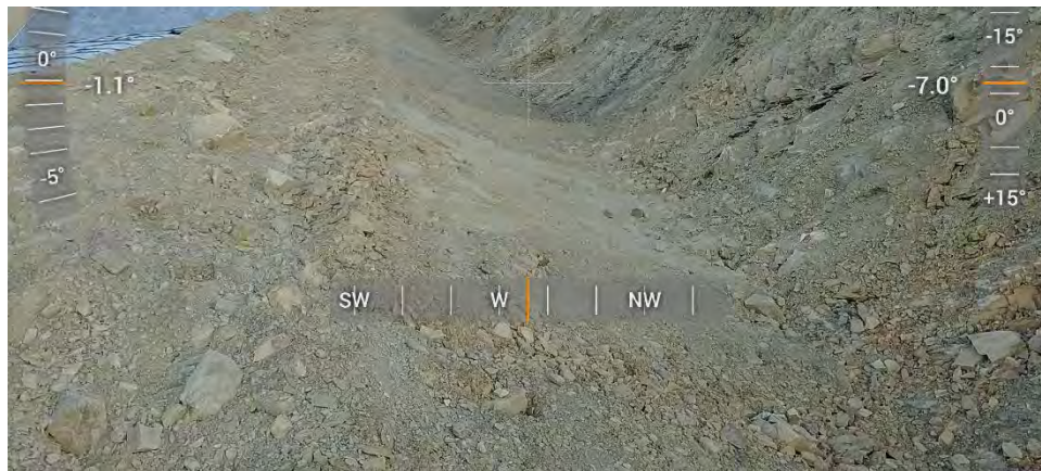
Figure 29: HLF – Collection ditch.
