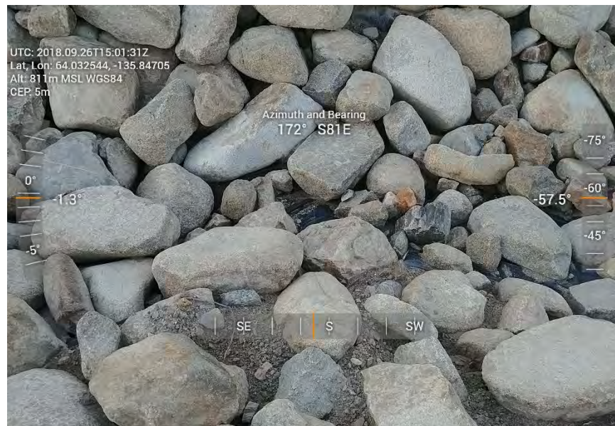
Figure 9: LDSP - Exposed liner in low level outlet channel.
