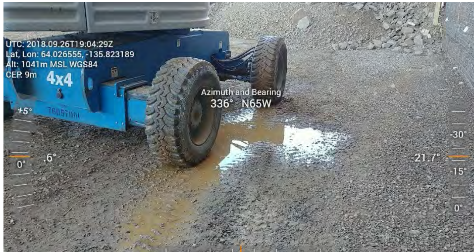
Figure 14: SC MSE - Minor ponding at base of MSE wall.
