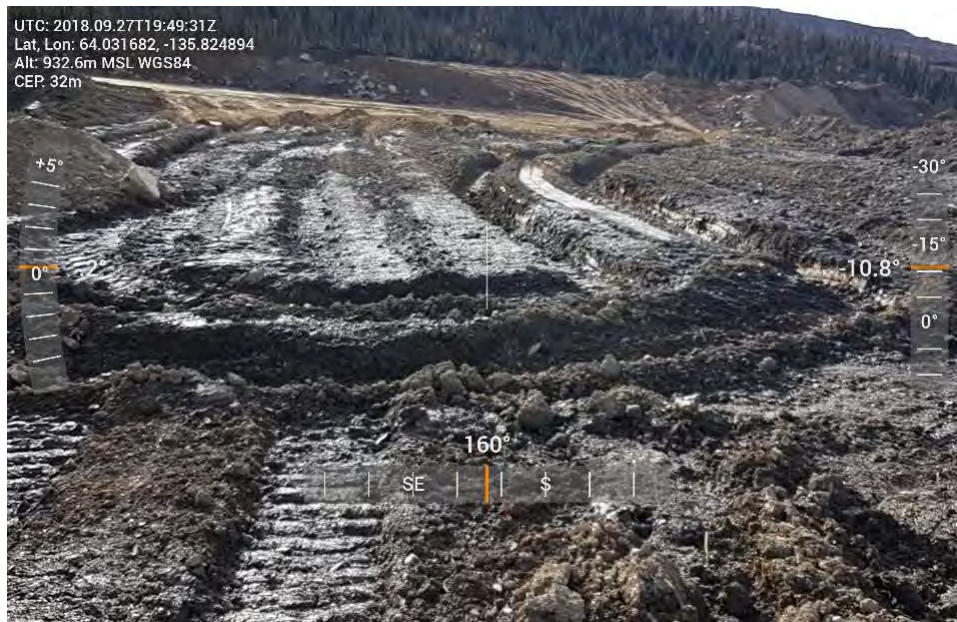
Figure 50: Stockpile B - North side saturated soils
