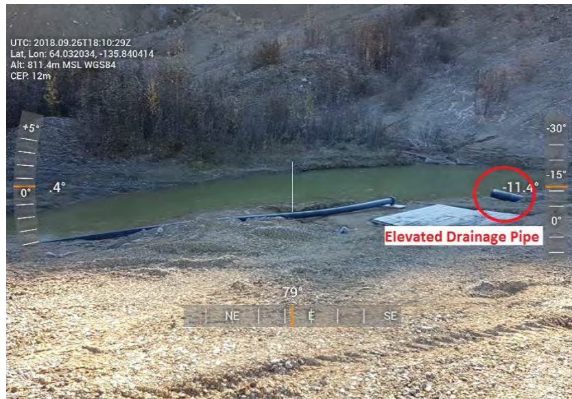
Figure 7: LDSP - Elevated Pond above Eastern side of fore bay
