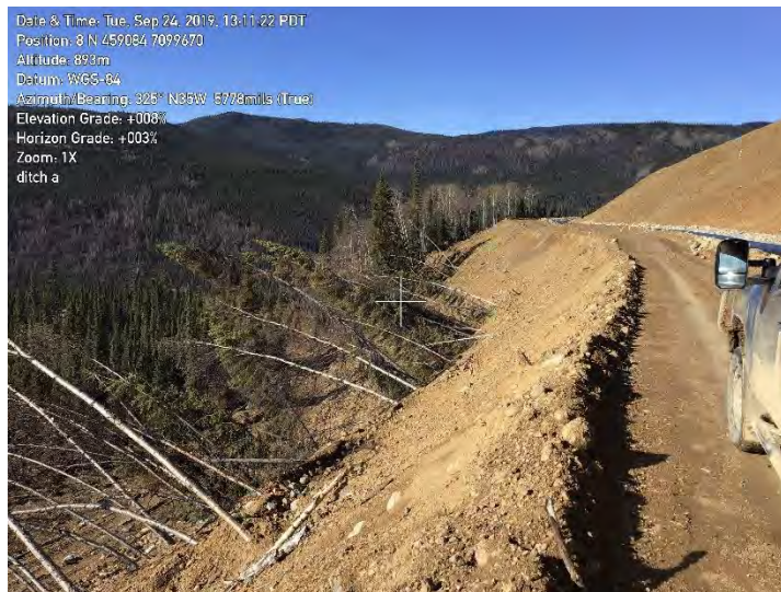
Figure 49: Trees in fill subgrade
