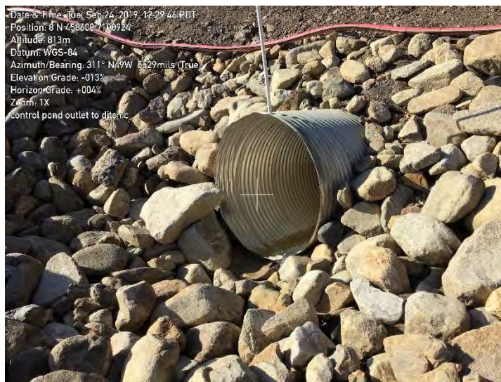
Figure 52: Outlet from control pond spillway and weir sump
