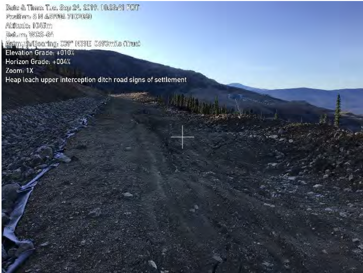
Figure 23: Road settlement along temporary access road
