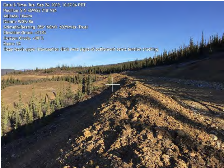
Figure 24: Downhill slope from road settlement
