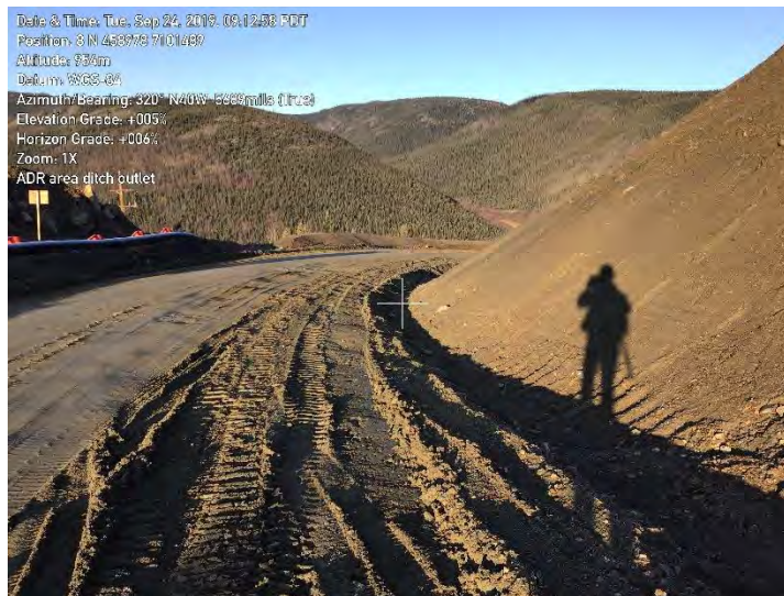
Figure 39: Flow into roadside ditch
