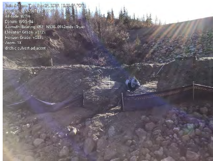
Figure 6: LDPS – Some flow from adjacent culvert
