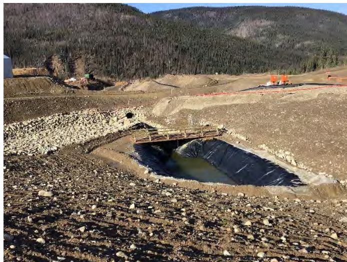
Figure 2: LDSP – Outlet Sump and Weir
