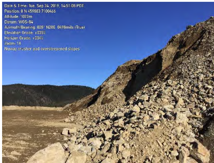
Figure 55: Over steepened slopes
