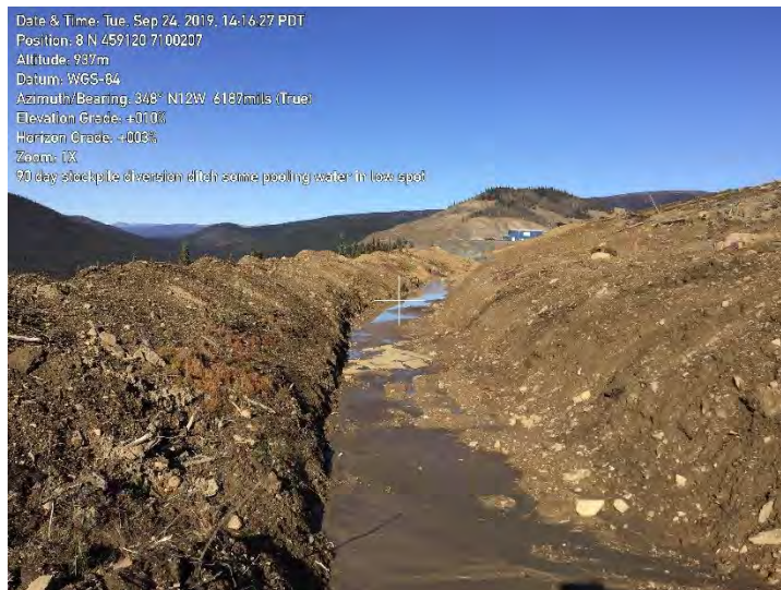
Figure 10: Pooling water in perimeter ditch
