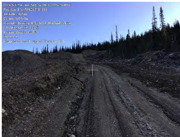
Figure 16: Scour on access road
