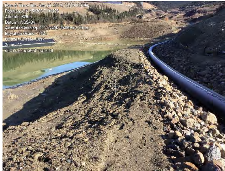
Figure 5: LDSP – Erosion on the Southwest slope
