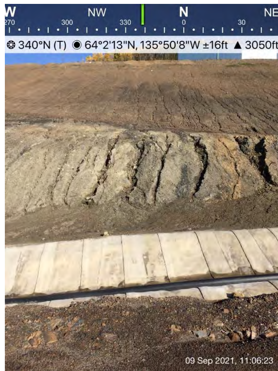
Figure 47: Rill erosion above HLF spillway
