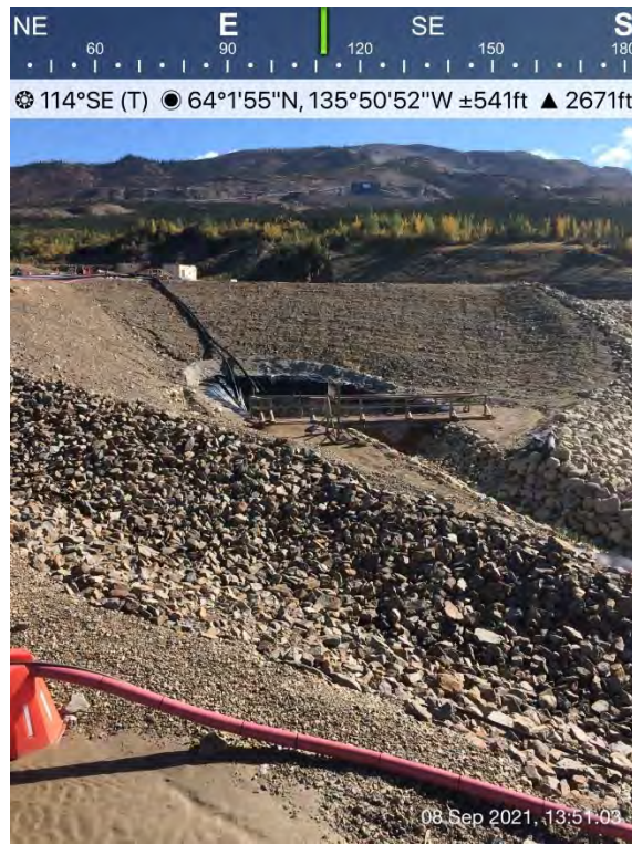
Figure 2: LDSP – Outlet Sump and Weir
