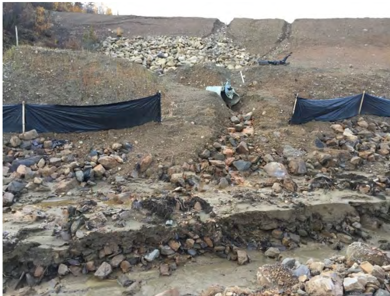
Figure 11: LDPS – Some flow from adjacent culvert 2020
