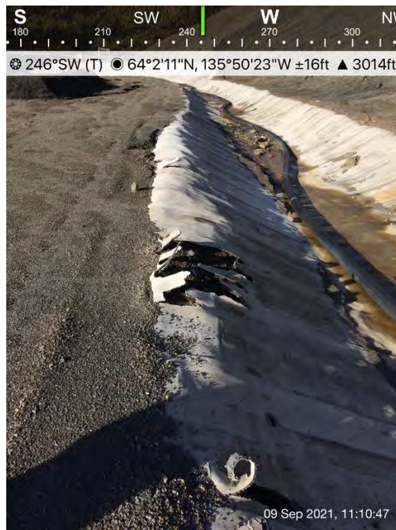
Figure 50: Heap leach spillway damage
