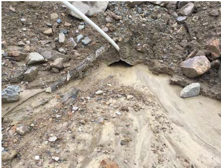
Figure 54: Secondary Stockpile drainage ditch culvert blocked 2020
