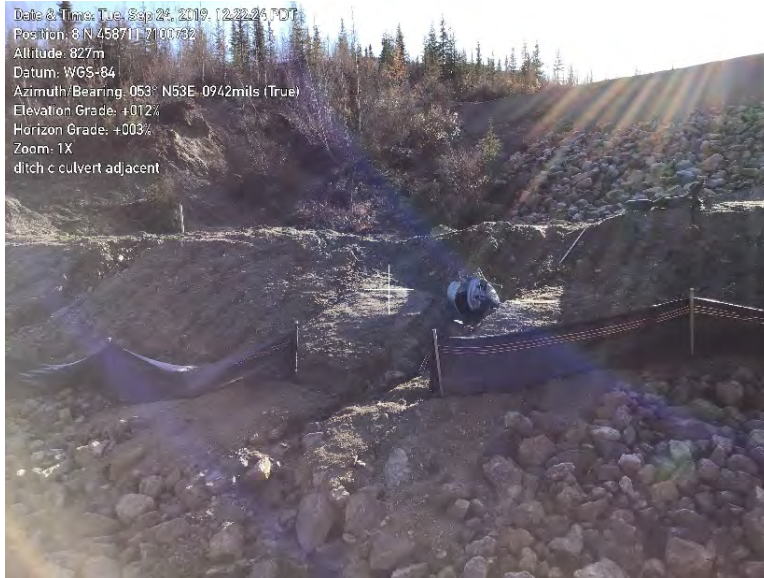
Figure 10: LDPS – Some flow from adjacent culvert 2019
