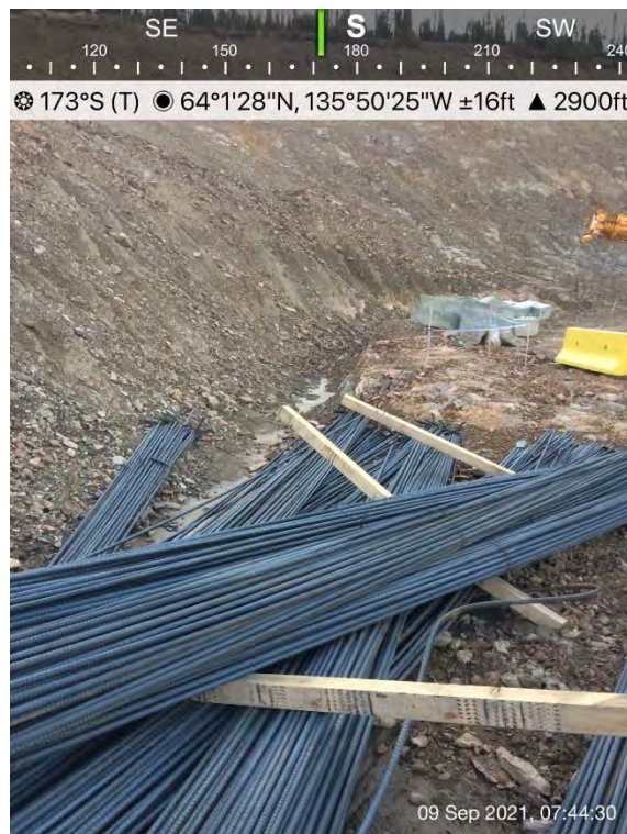
Figure 62: Drain ditch rebar blockage
