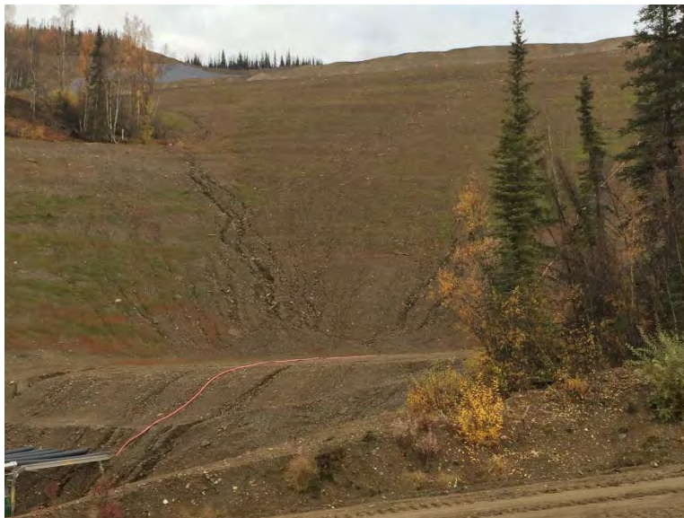
Figure 22: Scouring and rilling along toe slope of HLF (2020)
