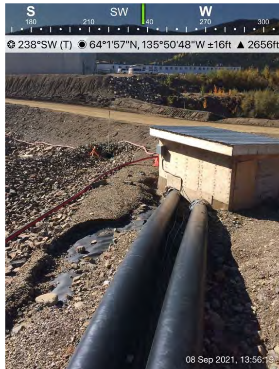
Figure 1: LDSP – Erosion adjacent to Shed and Diversion Ditch
