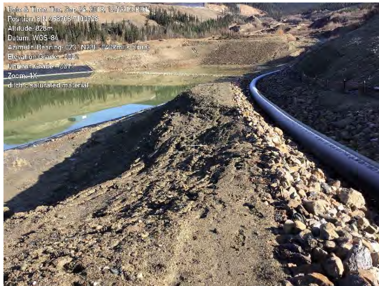
Figure 7: LDSP – Erosion on the Southwest slope 2019
