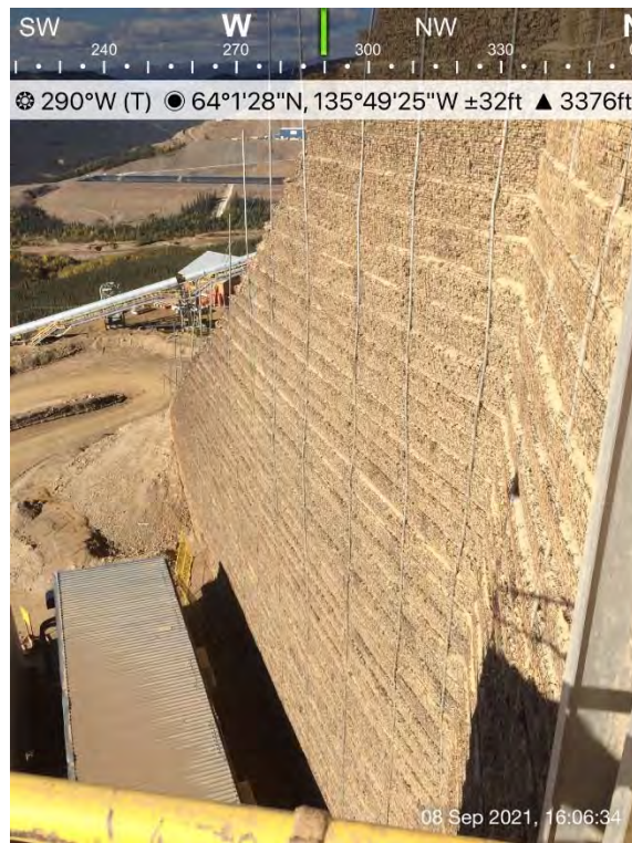
Figure 36: Primary Crusher North-West Wall
