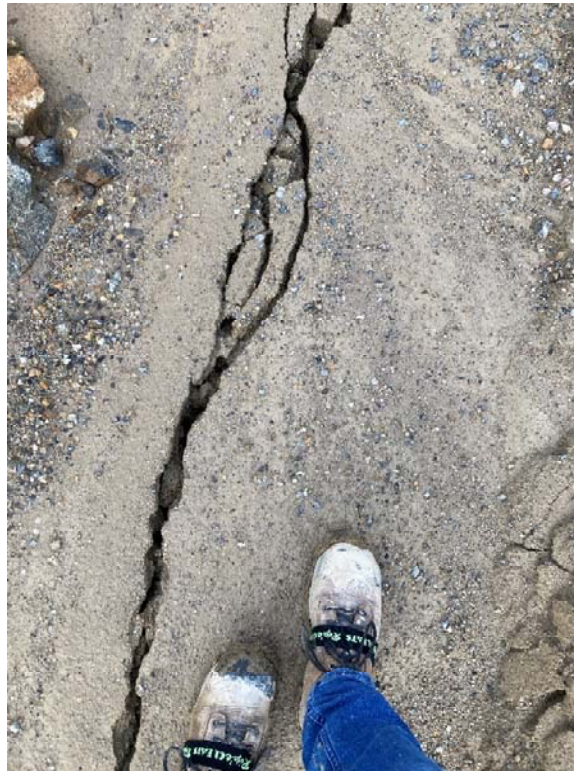
Figure 40: Platinum Gulch Dump Cracking
