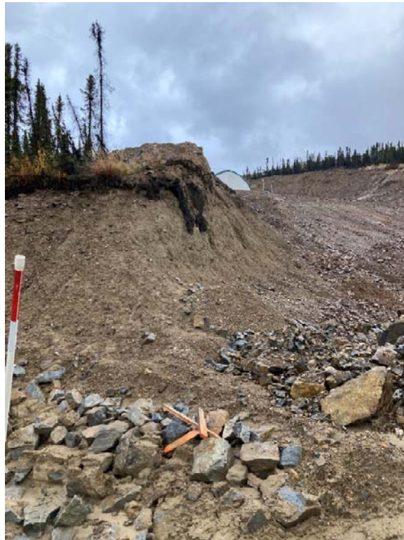
Figure 73: Over Steepened Slope – Truck Shop
