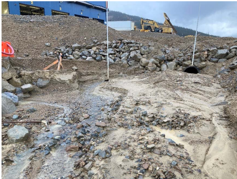
Figure 66: Ditch A culvert blocked
