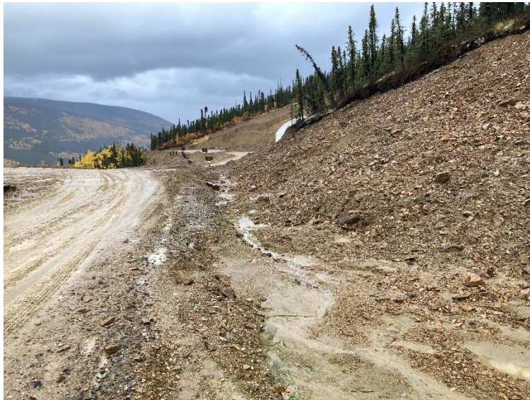
Figure 77: Orica ditch sediment build-up
