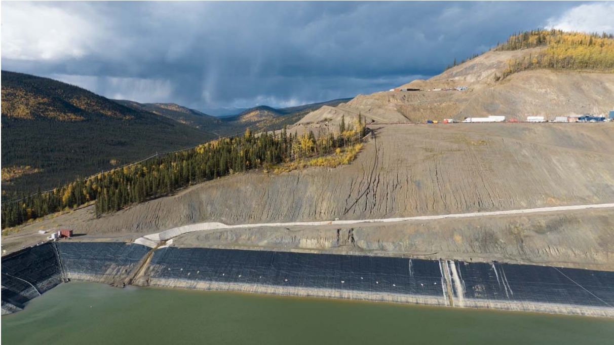
Figure 55: Rill erosion above HLF spillway
