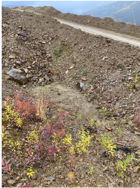
Figure 78: Orica ditch sump & drain culvert
