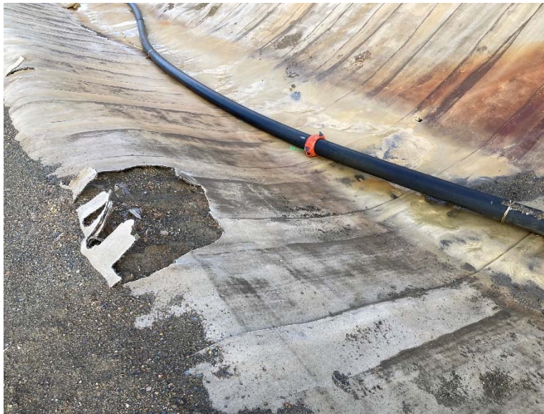
Figure 61: Heap leach spillway damage (2022)
