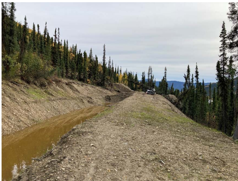
Figure 31: HLF Overburden sump system 2022
