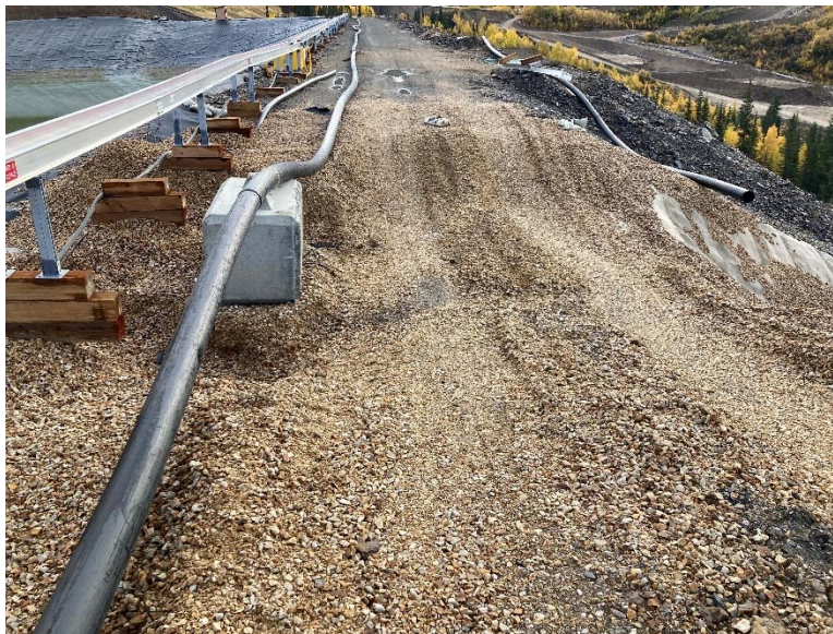
Figure 62: Events Pond Emergency spillway crush blockage
