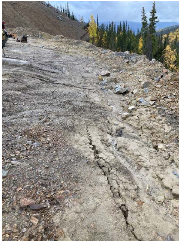
Figure 75: Cracking – Warehouse Pad
