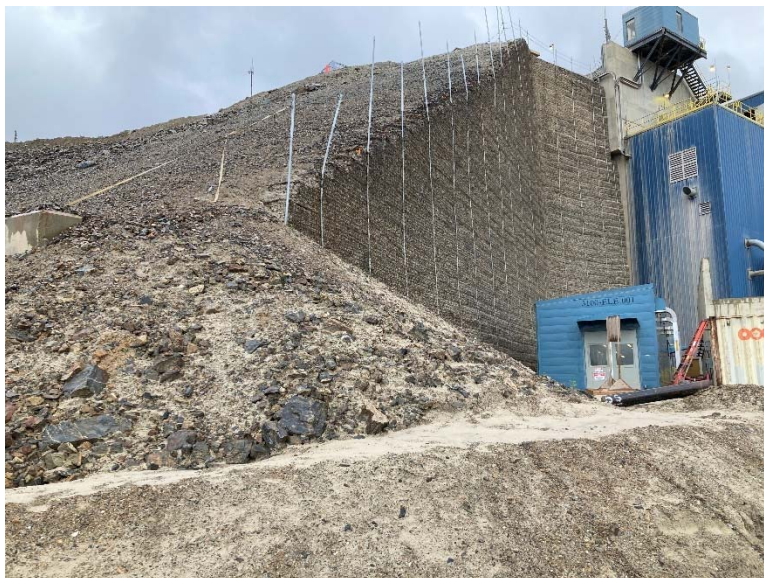
Figure 44: Primary Crusher North-West Wall
