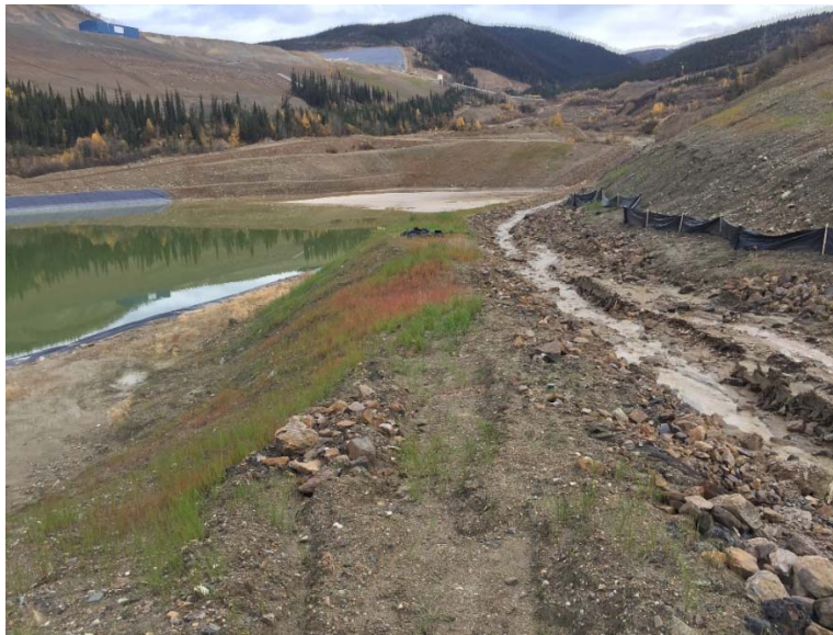
Figure 2: LDSP – Erosion on the Southwest slope 2020
