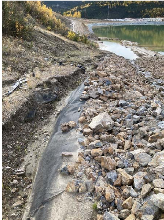
Figure 67: Ditch B Erosion (view towards LDSP)
