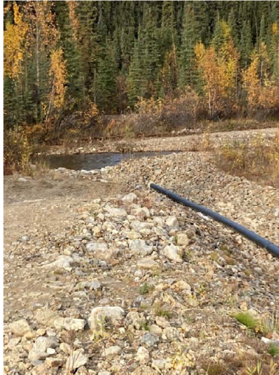
Figure 68: Ditch C Outlet (LDSP Pipeline Discharge)
