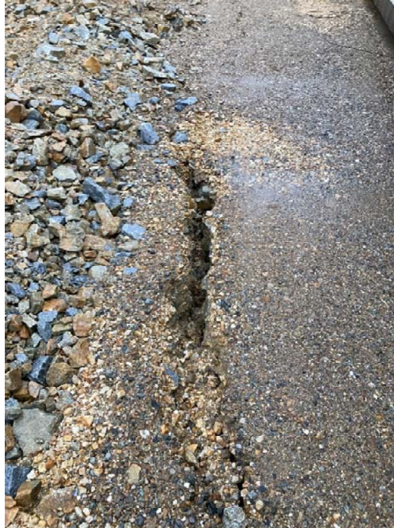
Figure 74: Cracking – Warehouse Pad
