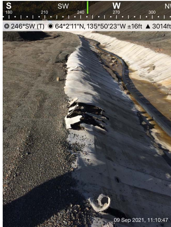
Figure 59: Heap leach spillway damage (2021)
