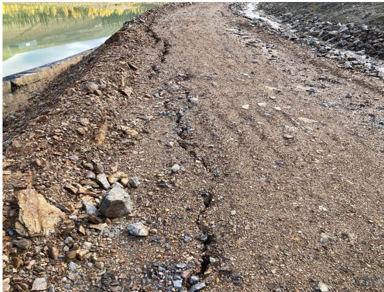
Figure 4: LDSP – Cracking on the Southwest slope 2022
