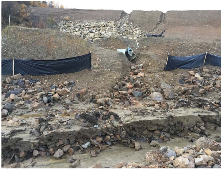
Figure 6: LDSP – Some flow from adjacent culvert 2020
