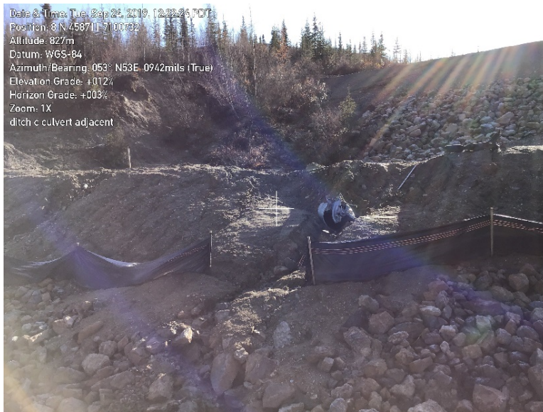
Figure 5: LDSP – Some flow from adjacent culvert 2019
