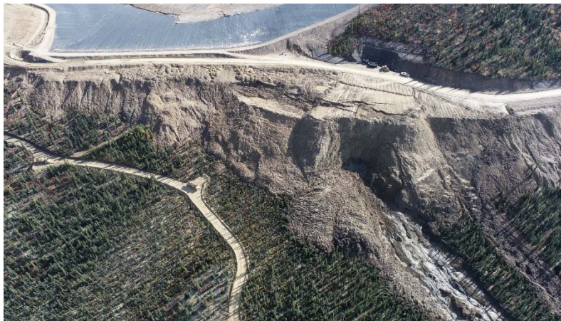
Figure 27: HLF Overburden Stockpile collapse – plan view 2021
