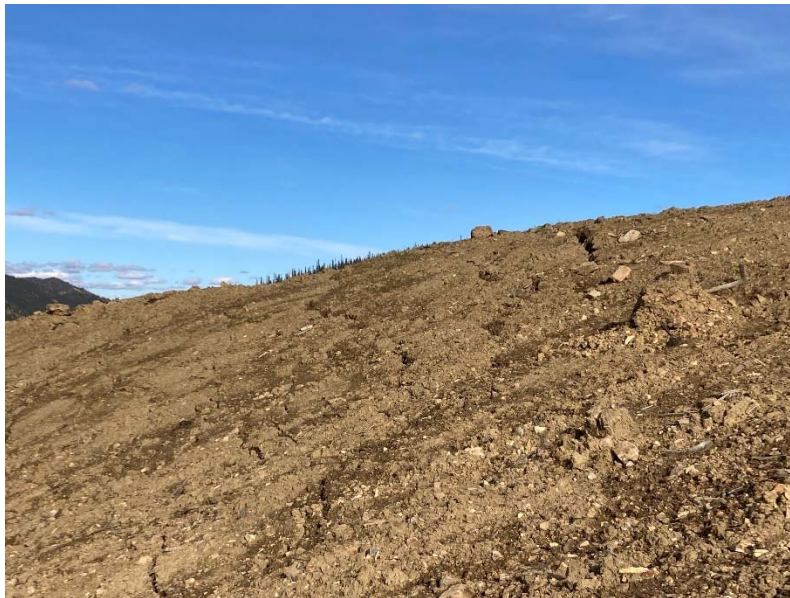
Figure 29: HLF Overburden Stockpile collapse – slope cracking 2022
