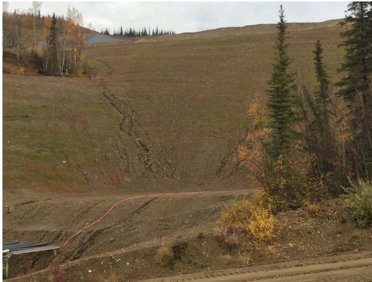
Figure 19: Rilling along toe slope of HLF (2020)
