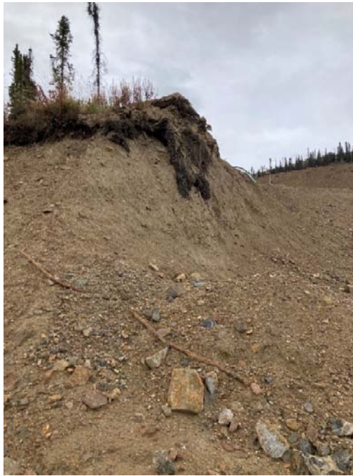
Figure 66: Over Steepened Slope – Truck Shop
