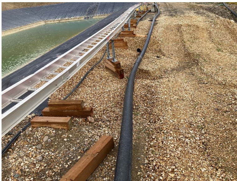
Figure 57: Events Pond Emergency spillway crush blockage
