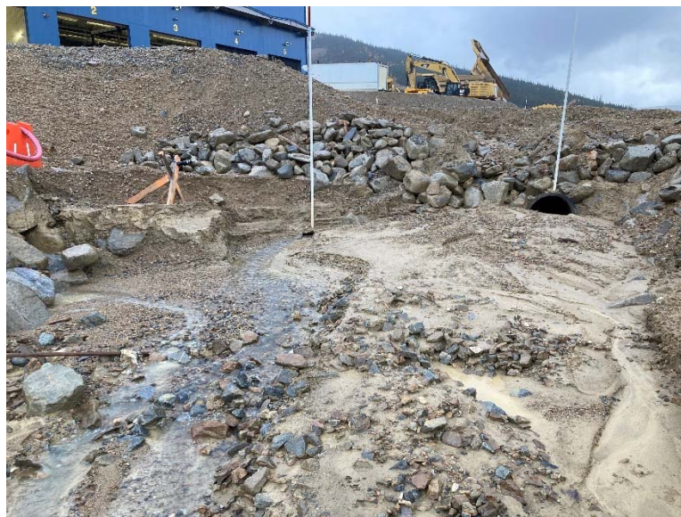
Figure 62: Ditch A culvert blocked (2022)
