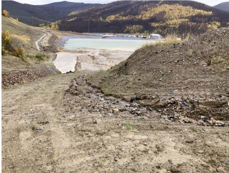
Figure 63: Ditch B Erosion (view towards LDSP)
