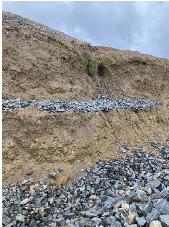
Figure 10: Secondary Stockpile Cut Slopes 2023 – Surficial Slough
