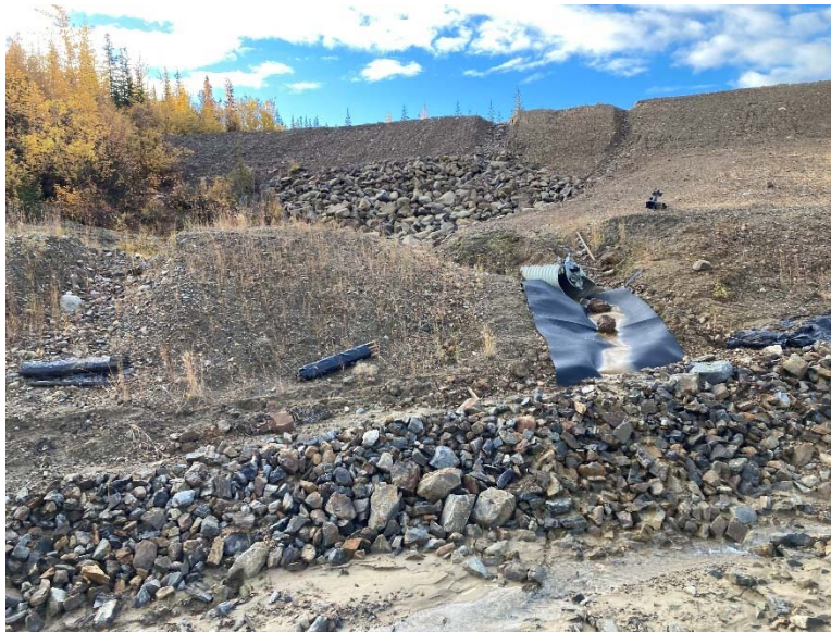
Figure 4: LDSP – Some flow from adjacent culvert 2022
