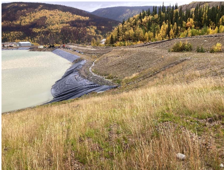
Figure 7: Material wash-out above the LDSP
