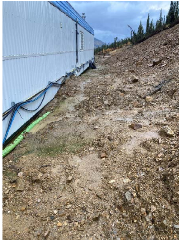
Figure 72: Orica site trailer sediment build-up (2022)
