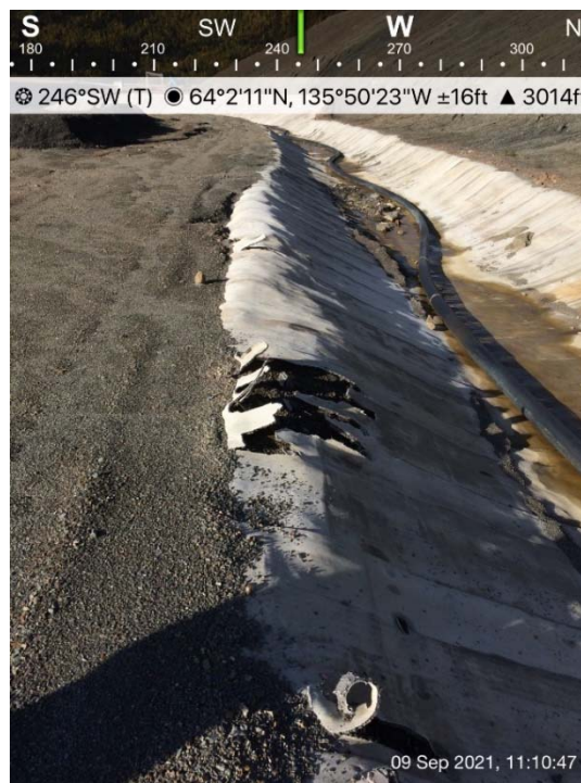
Figure 55: Heap leach spillway damage (2021)
