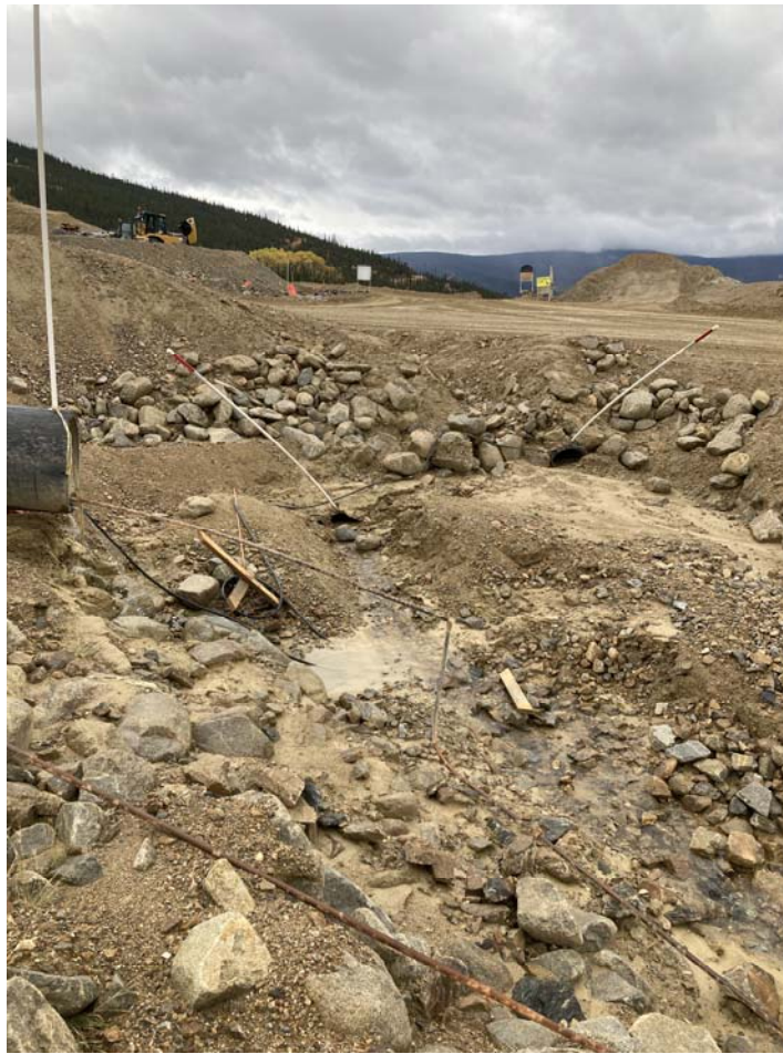
Figure 61: Ditch A culvert blocked (2023)
