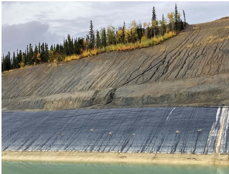
Figure 50: Rill erosion above HLF spillway (2023)
