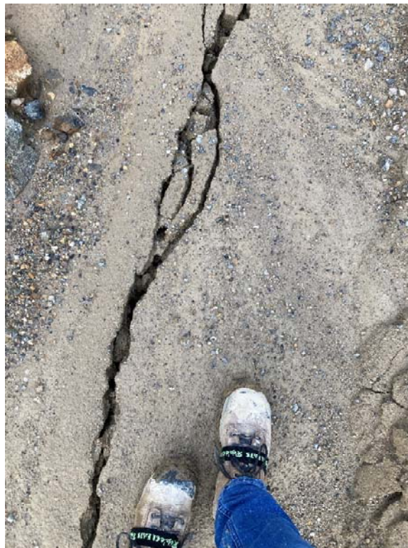
Figure 34: Platinum Gulch Dump Cracking (2022)
