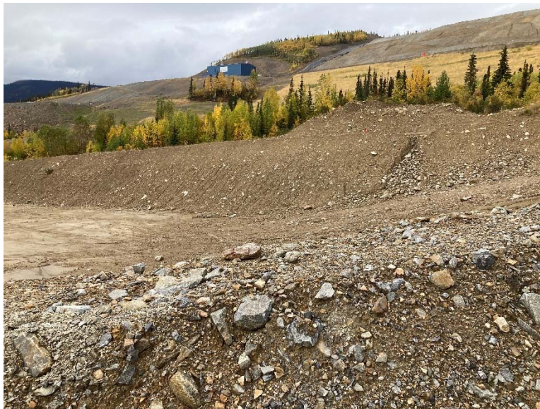
Figure 59: Emergency Pond Slope Erosion
