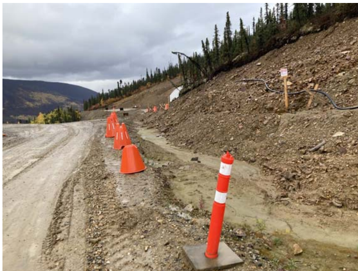
Figure 70: Orica ditch sediment build-up
