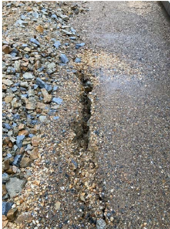
Figure 67: Cracking – Warehouse Pad (2022)
