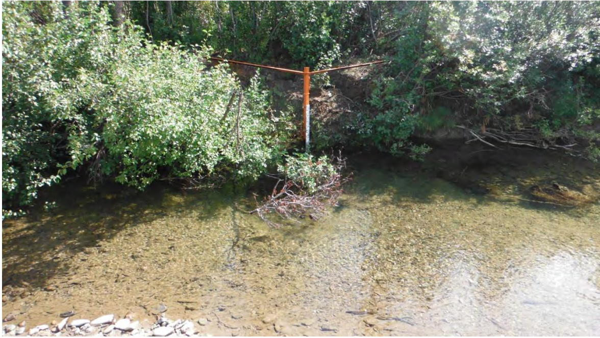
Figure 9 – W-5 after repairs. Note that the braces have been moved up onto the bank and that the original 2007 bank has sloughed into the creek.
