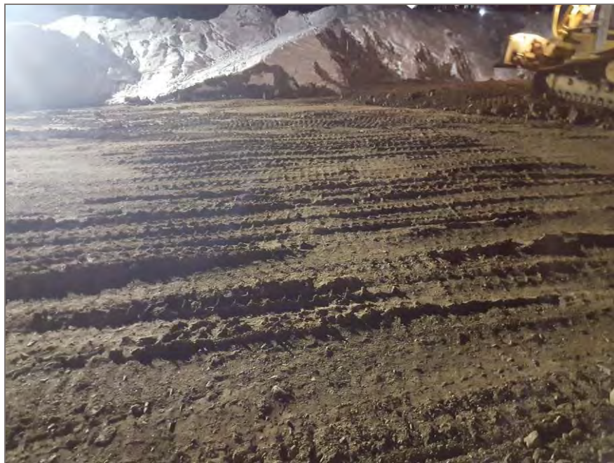
Photo 1: Unstable material noted by dayshift
