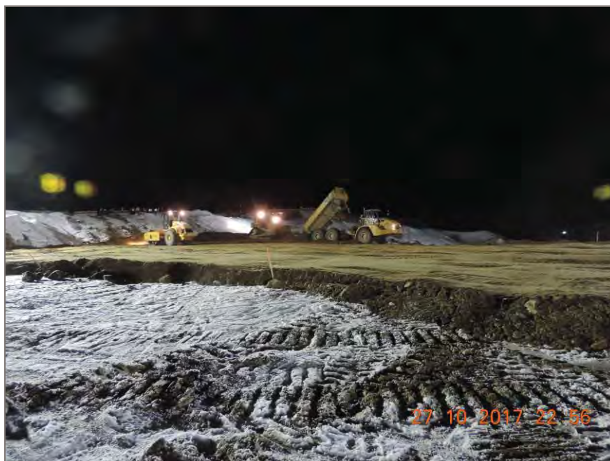
Photo 2: Placement of pit run base material for south dam on first lift.
