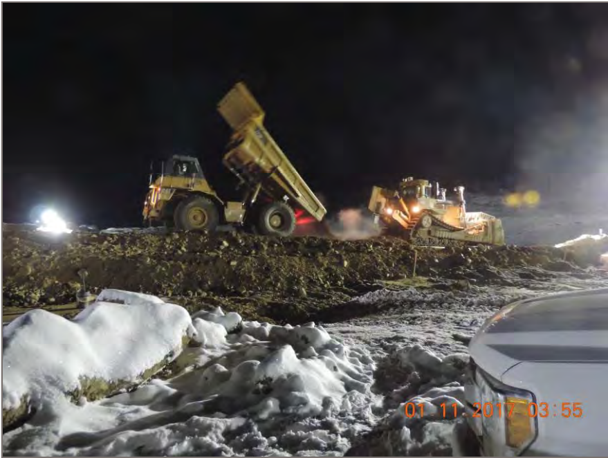
Photo 3: Placement of backfill material using a CAT 773 haul truck and D10T Dozer at grade 813.1m.
