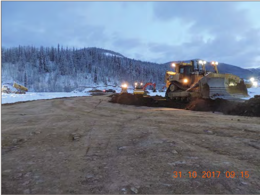
Photo 3: 2-Single Smooth Drum packers compacting behind Cat D10T Dozer spreading subgrade fill
