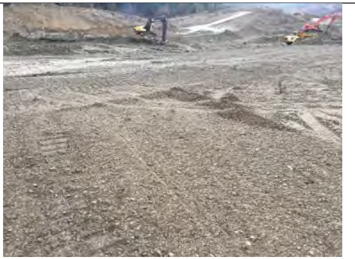
Photo 4 Native material present at midpoint of West Dam. Well graded, no cobble/boulders
