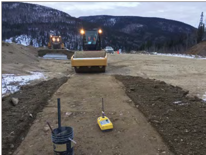
Photo 5: Control strip testing of material proposed for initial backfill of the south control dam sub-excavation.
