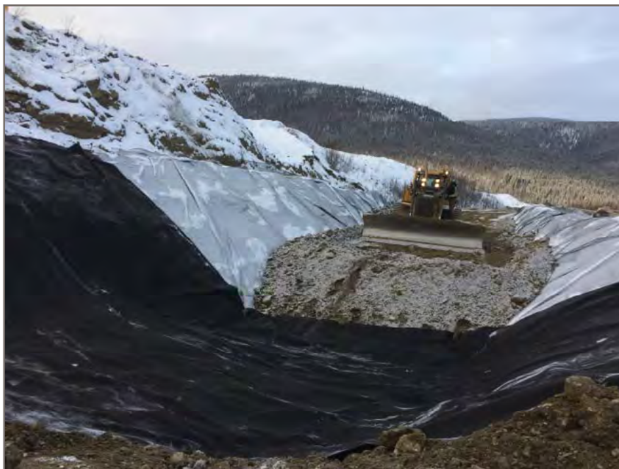
Photo 5: Bridge lift being extended into area previously used as sump that was located adjacent east side toe of south dam.
