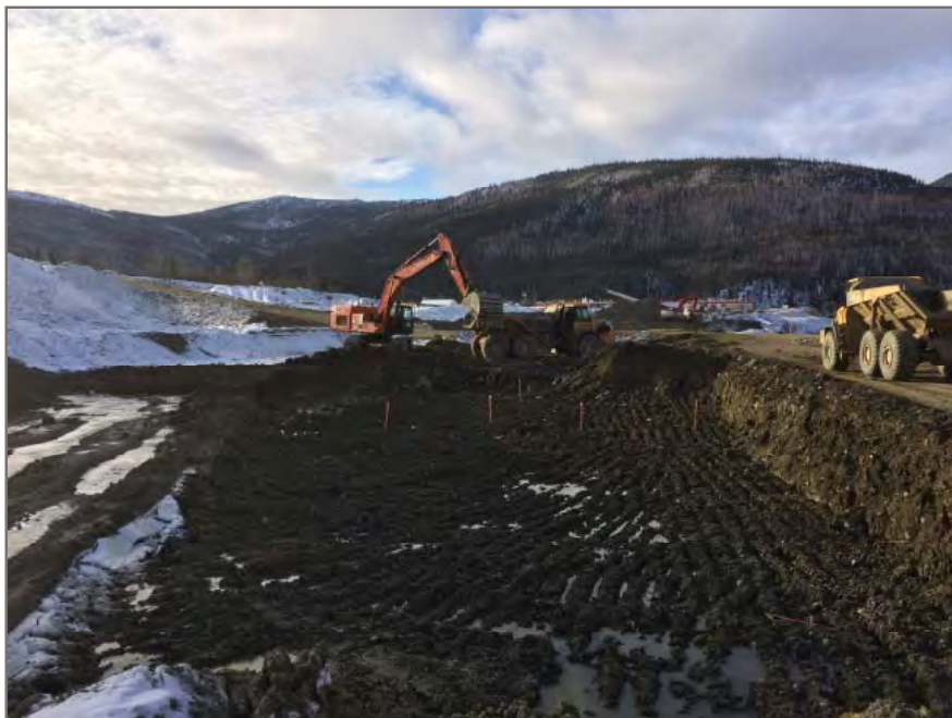
Photo 5: View looking west at sub-excavation in progress along south side of control pond.
