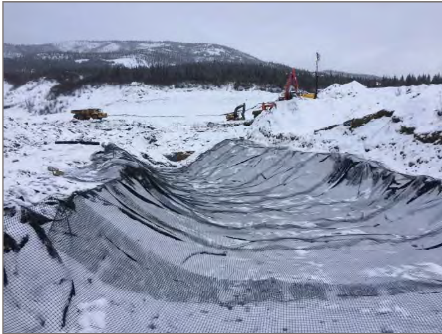
Photo 5: View from west end looking east at geotextile and geogrid placed throughout sub-excavation.
