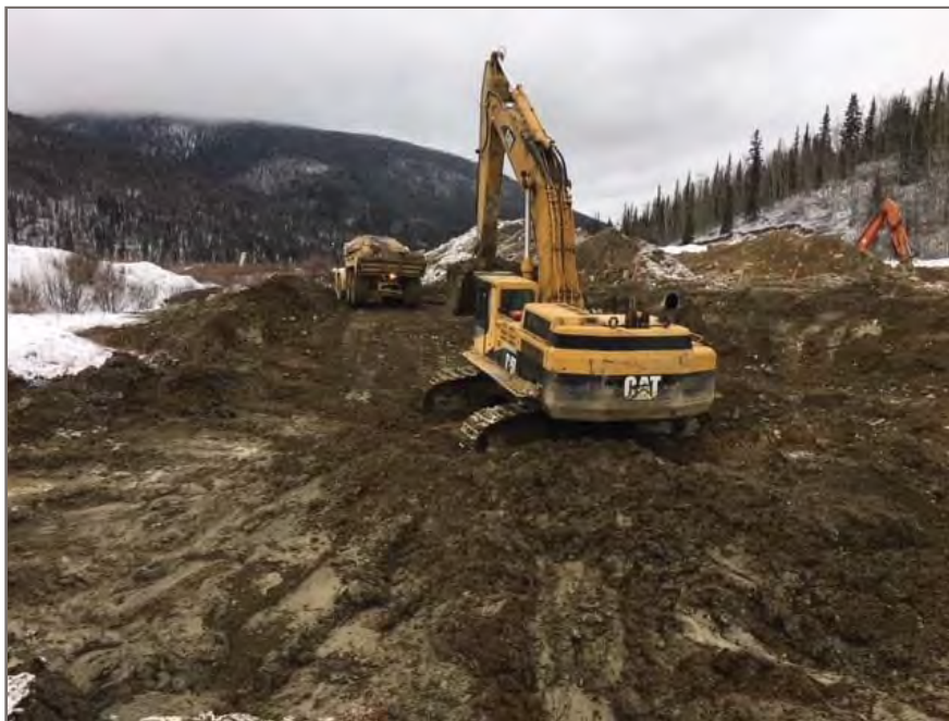
Photo 4 View looking west at in-progress sub-excavation of soft, saturated silt/clay material within southwest area of containment pond
