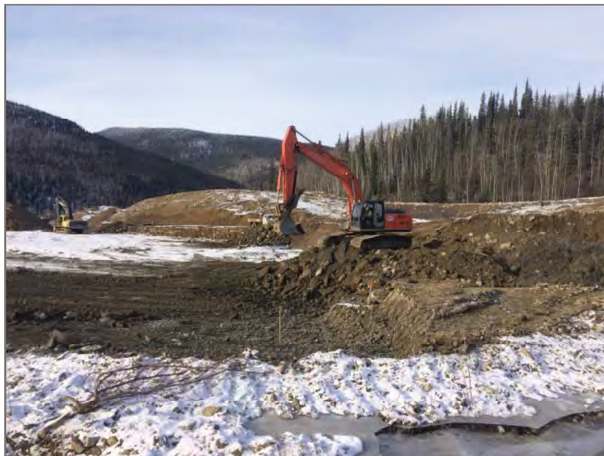
Photo 2: Sub-excavation in progress with and near north end of spillway area of control pond.
