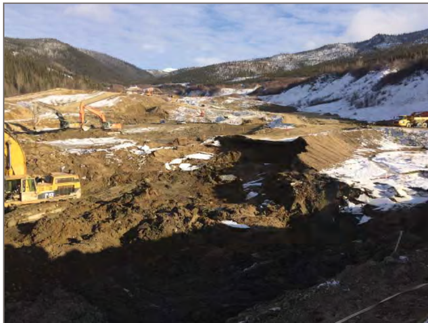
Photo 1: View of slough from east side of excavation within south dam area.
