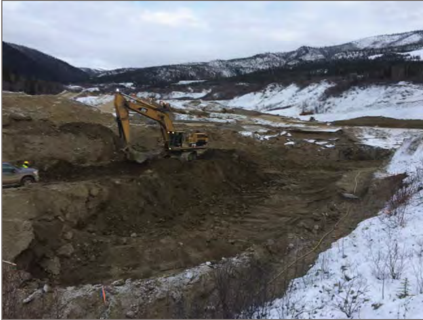
Photo 5: View looking northeast at sub-excavation in progress along south side of control pond. Estimated depth at 4.5 m below design depth.
