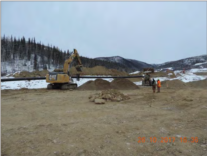
Photo 4: HDPE 450mm Pipe moved to LLO Trench with one loader and two excavators
