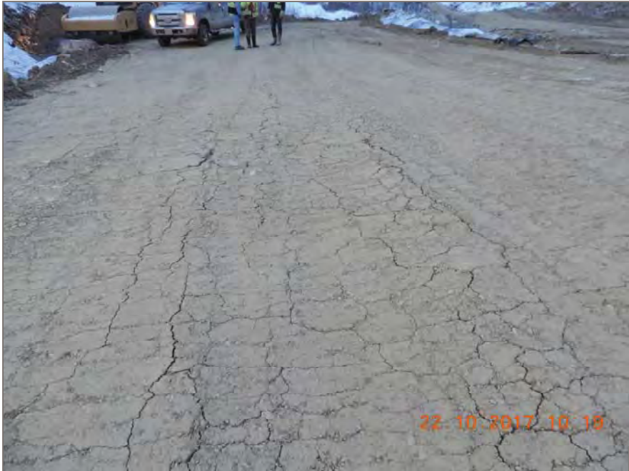
Photo 1: Sub grade failure. Proof Roll performed showed heavy rut and roll
