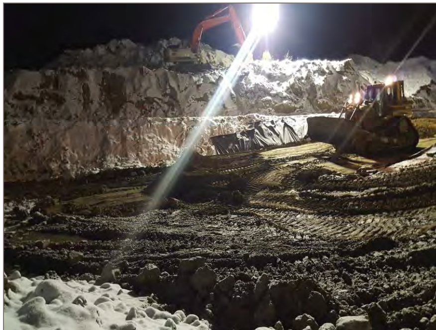
Photo 1: Placement of bridge lift east side of excavation where underlying saturated material is located.
