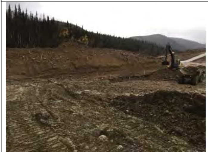
Photo 3 View of Northeast corner of pond. Contractor plans to push material down from crest of hill to build up the North slope between the crest and toe stake lines shown running along the cut edge of hill.
