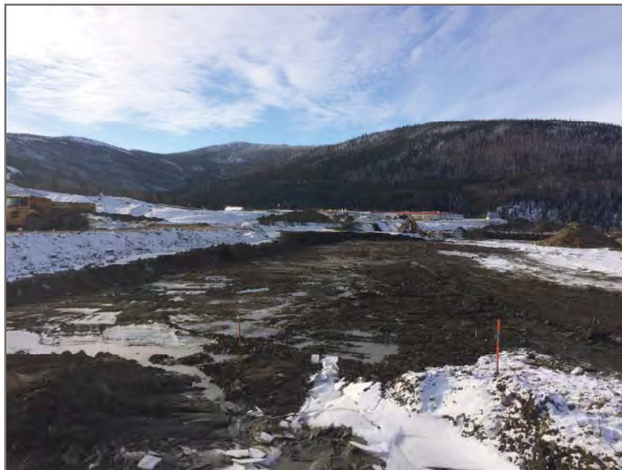
Photo 1: View looking west from east end at partial excavation of control pond
