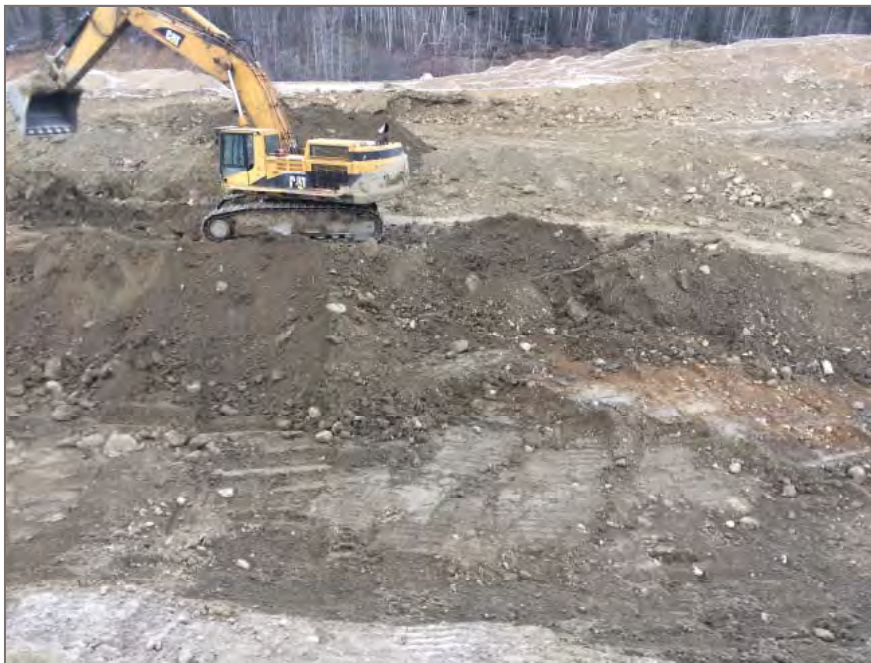
Photo 4: View looking north at excavation of south end of control dam in progress.
