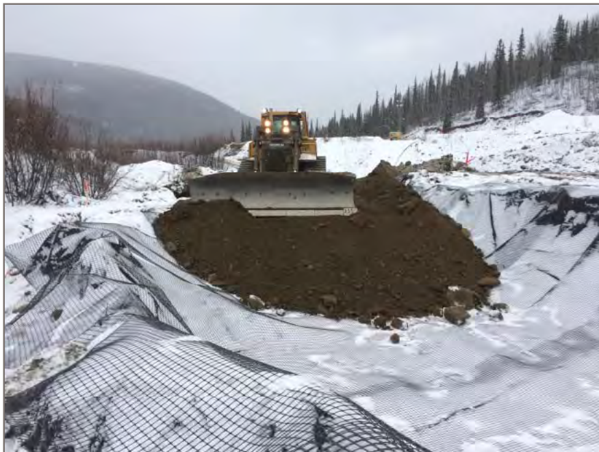
Photo 6: View from south embankment looking northwest at pit run being padded throughout the west end of the sub-excavation.
