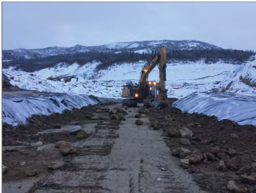
Photo 8: Coarse rock being pulled away from geotextile and geogrid lined excavation walls.
