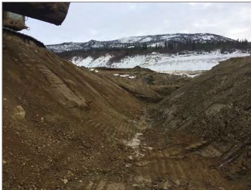
Photo 2: View looking east from mid-point of sub-excavation within south end of control pond dam area.
