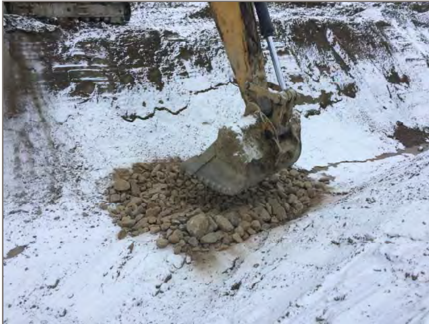
Photo 1: Placement and pushing coarse rock into the soft base within the South Control Dam sub-excavation.
