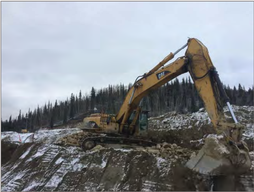
Photo 4: CAT 265 excavator used to place and push coarse rock into soft subgrade of excavation area.
