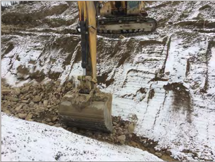
Photo 3: Placement and pushing rock into the narrow section of the excavation in-progress.
