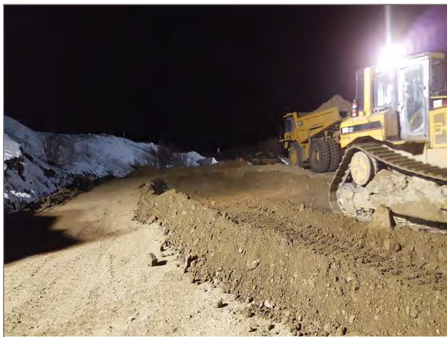
Photo 2: Unstable material located within Berm
