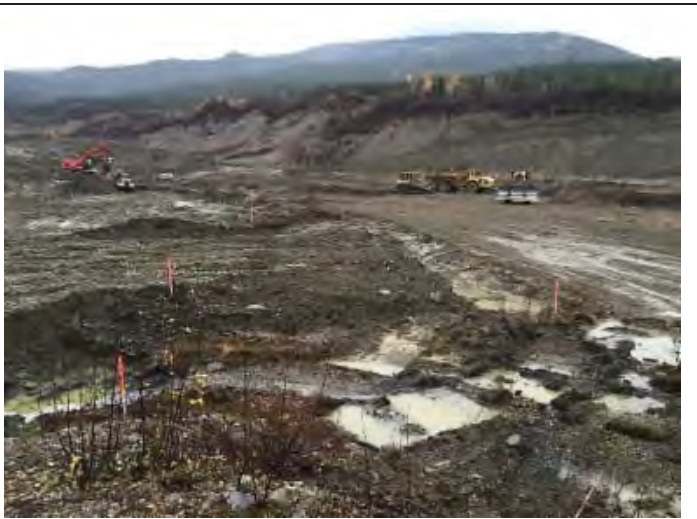
Photo 2 East view of West Dam (in middle ground). Notice difference in material in dam footprint from left to right.
