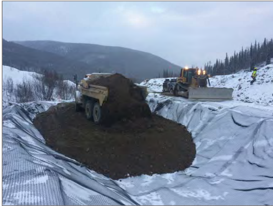
Photo 7: View looking northwest at pit run gravel placement within west end of sub-excavation.
