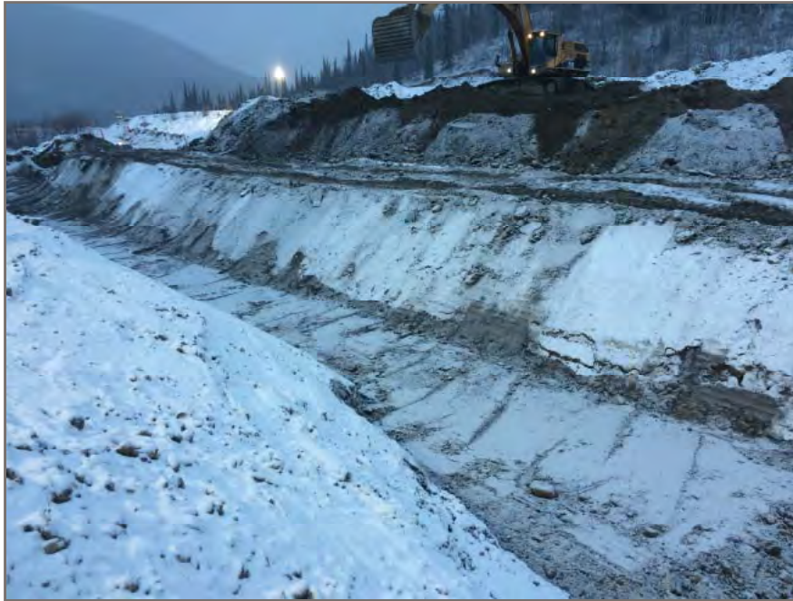
Photo 1: View looking northwest at 300 mm thick layer of pit run gravel placed within sub-excavation prior to geotextile and geogrid placement.
