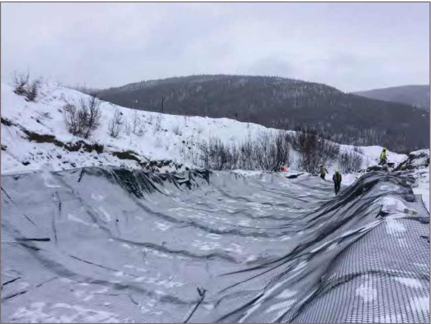
Photo 4: View from north embankment looking south west at geogrid placed over geotextile.
