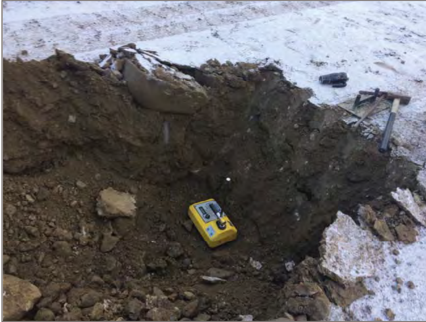
Photo 3: Field density testing in progress within testpit excavated into the bridge lift
