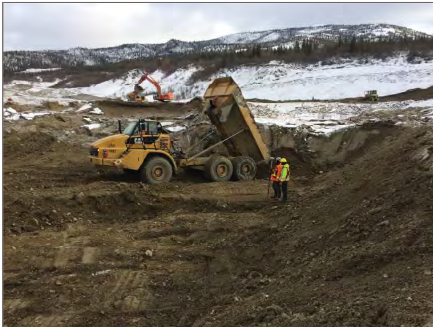
Photo 2: View looking east at placement of buttress in progress against toe of east wall of excavation and base completed to about 4.5 m below design depth.
