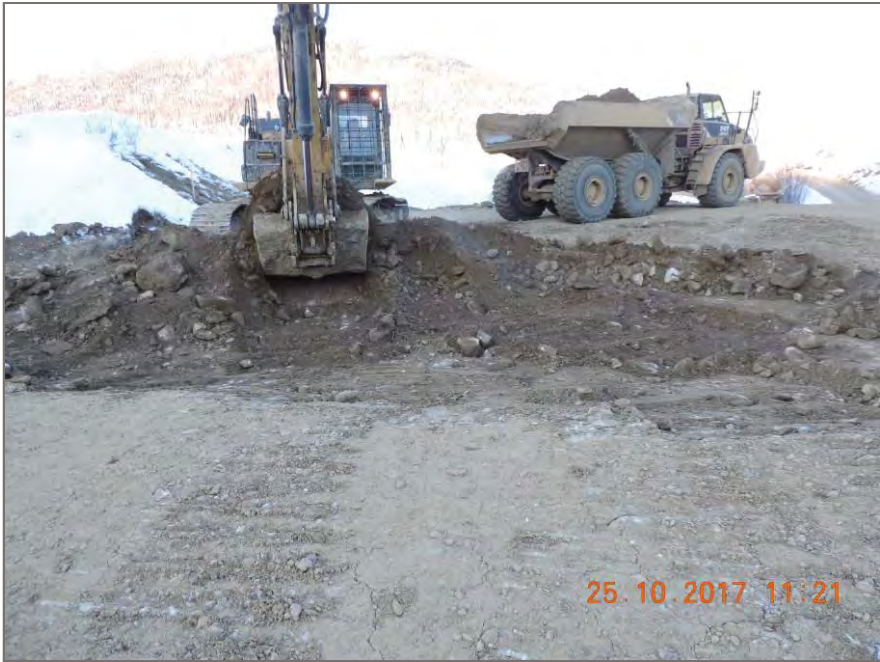
Photo 3: One of two soft spots excavated out due to excessive rut and roll
