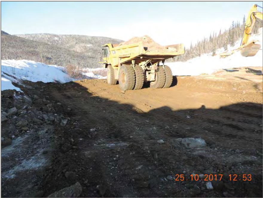
Photo 4: Cat 773D Rock Truck packs prior lift after excavation before continuing backfill
