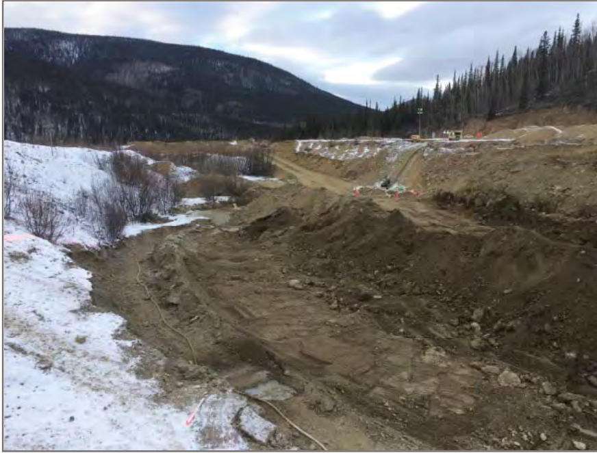
Photo 3: View looking west at partial excavation of soft, saturated soils within south end of control dam area.
