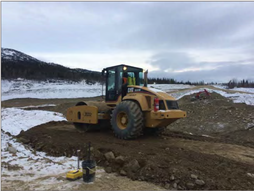
Photo 4: Material proposed for fill within the south control sub-excavation being prepared for control strip testing.
