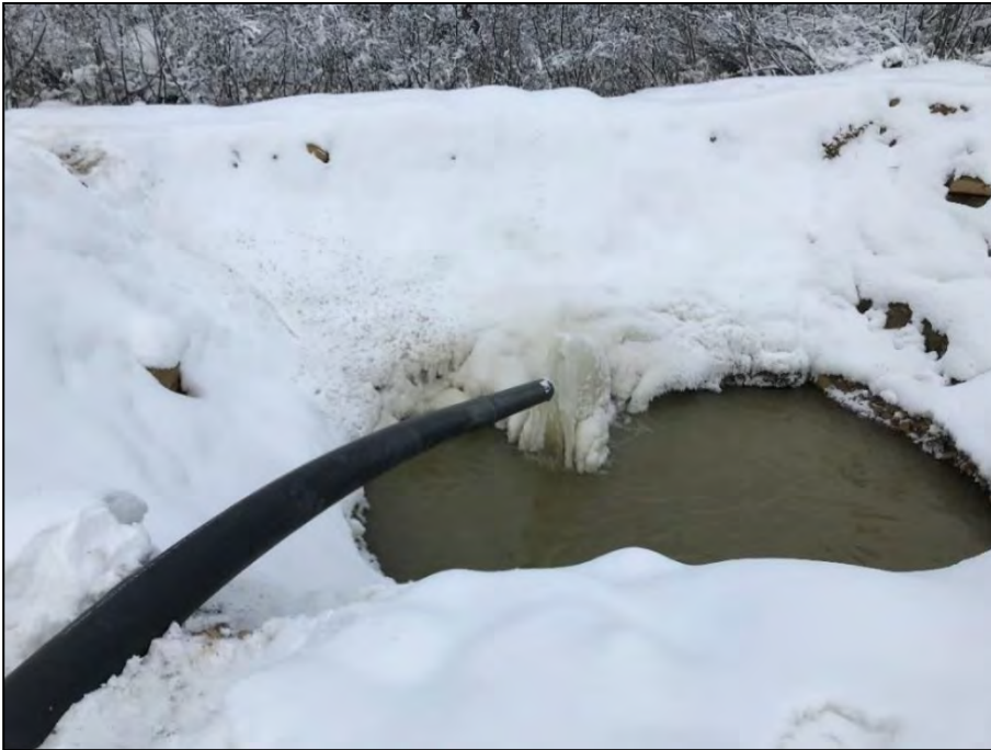
Figure 3.11-4: Temporary Exfiltration Sump
