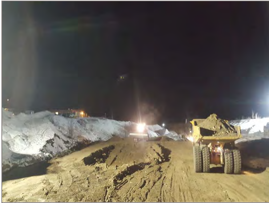
Photo 3: Unstable material removed from berm
