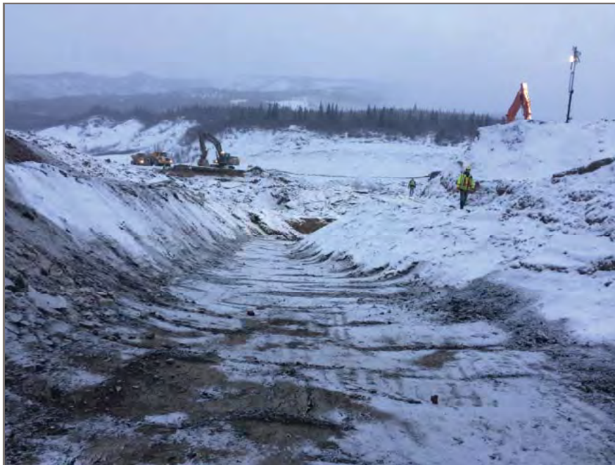
Photo 2: View looking east at 300 mm thick layer of pit run gravel placed within sub-excavation prior to geotextile and geogrid placement.
