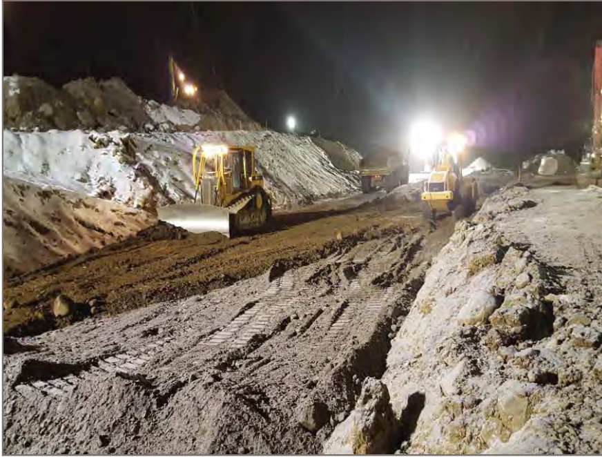
Photo 3: Placement and compaction of pit run within pipe trench and adjacent area.
