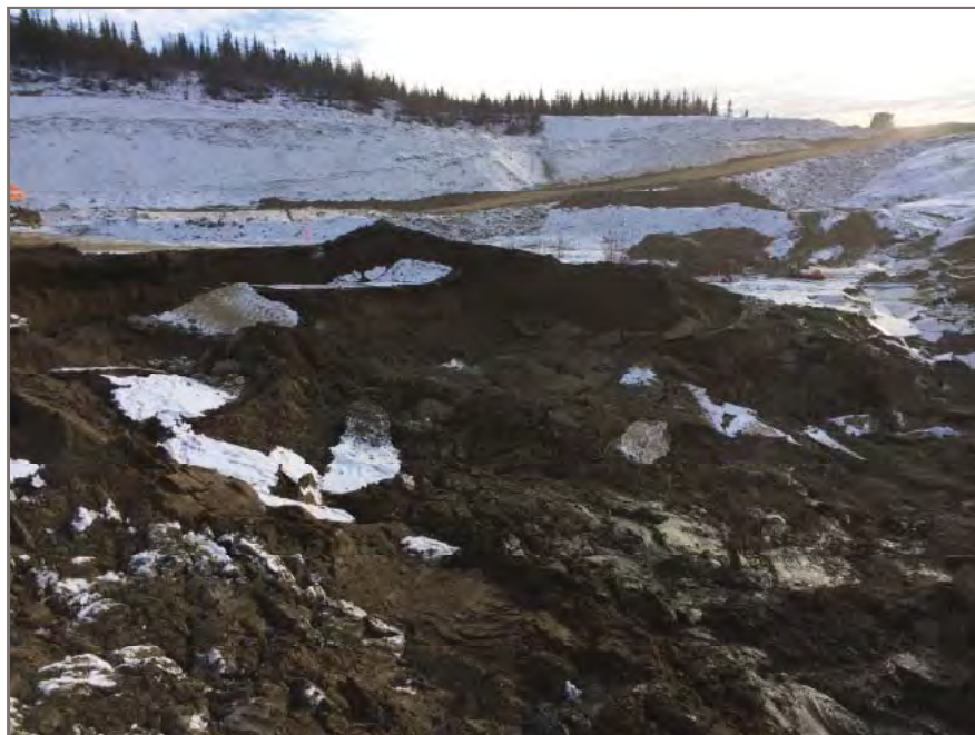
Photo 2: View looking south at sloughing soils from east wall of south dam excavation area.
