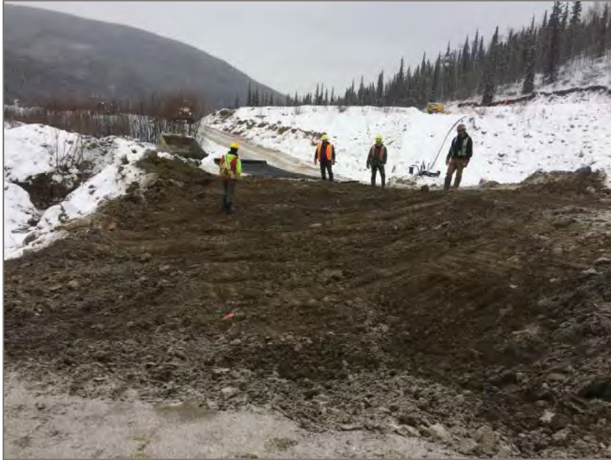
Photo 7: Entrance into fill area within west toe of dam where unstable material removed in preparation for geotextile placement
