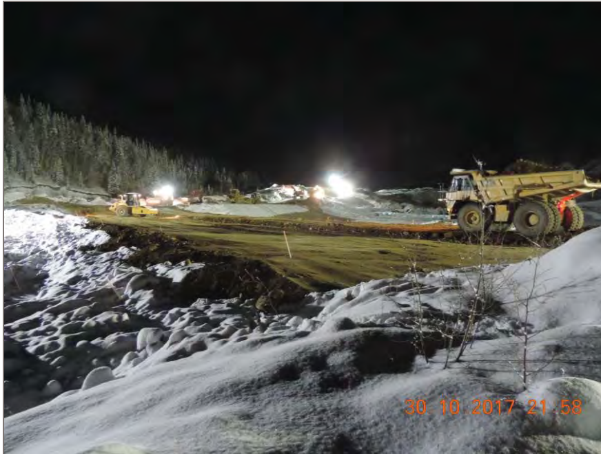
Photo 1: Compaction and placement of pit run using a CAT 773 and D10T Dozer at grade 811.3m.
