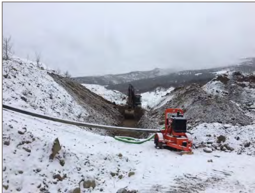
Photo 1: Sub-excavation of underdrain area to subgrade at west end of Control Pond.
