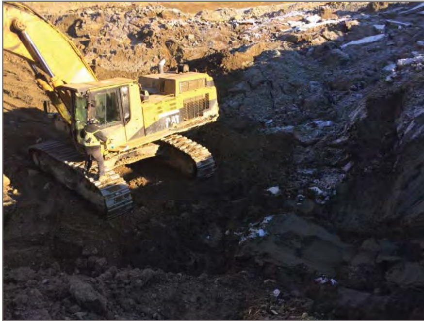
Photo 1: Continued slough from east side of excavation within south dam area.
