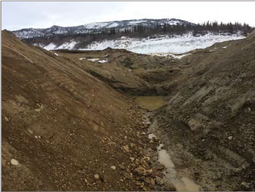
Photo 3: View looking east at sub-excavation within area of the south control dam.
