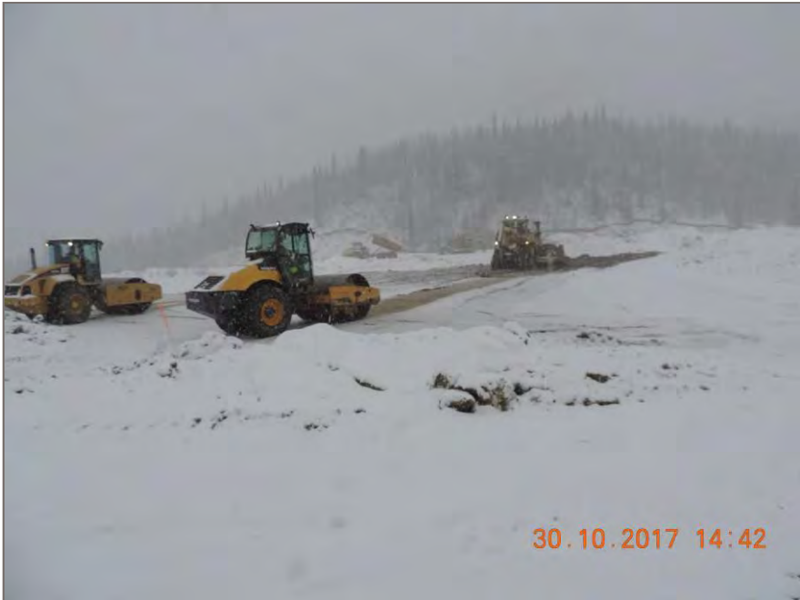
Photo 3: 2-Single Smooth Drum packers working on pad with Cat D10T Dozer spreading subgrade fill
