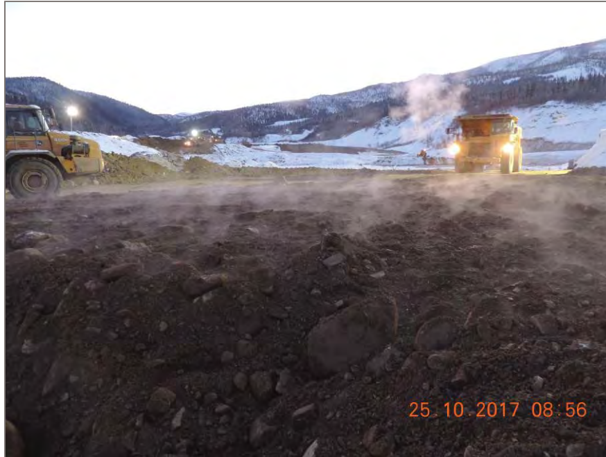
Photo 1: Positive temperature fill material placed and compacted with Cat 773D Rock Truck
