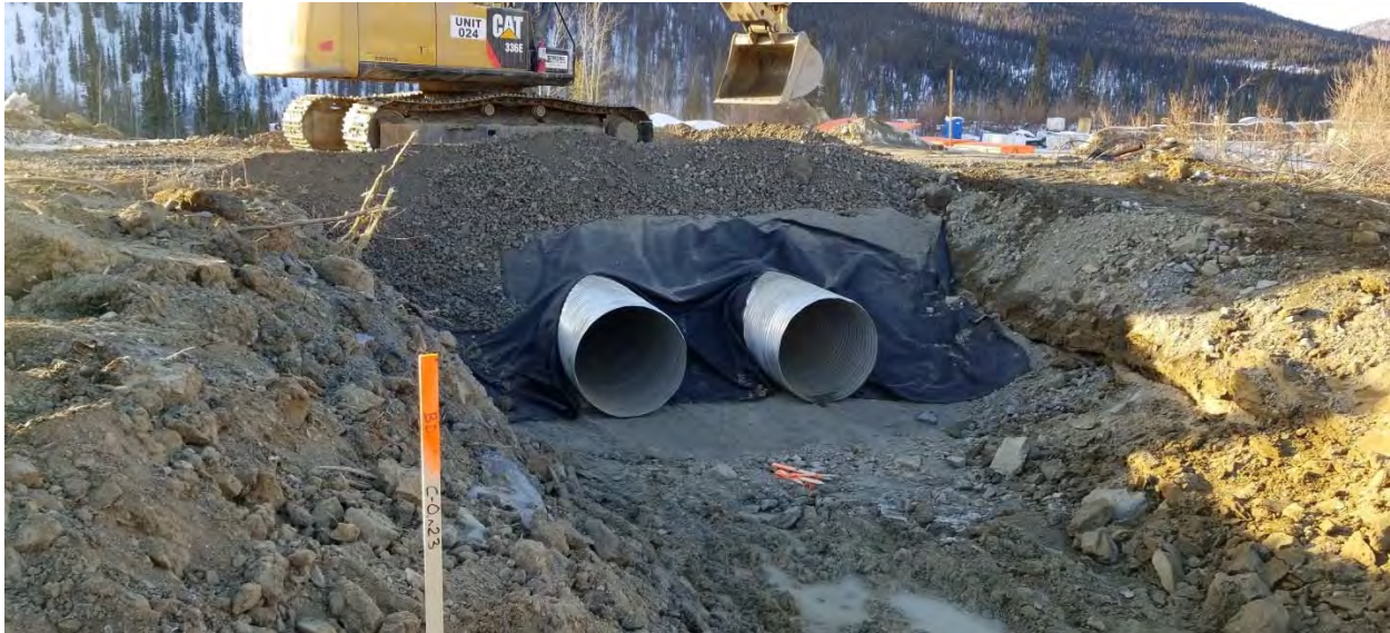
Figure 19. Ditch C Dual 1200mm Culverts near STN 0+200
