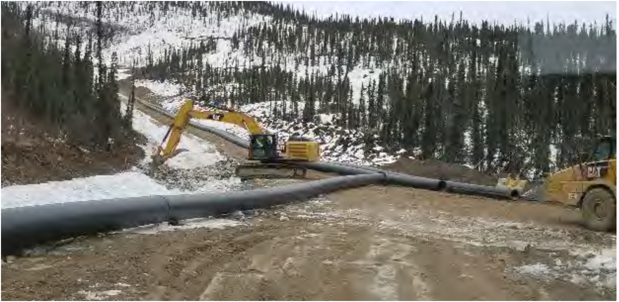
Photo 12 - 19.04.06 - Ditch A Collection Sump
