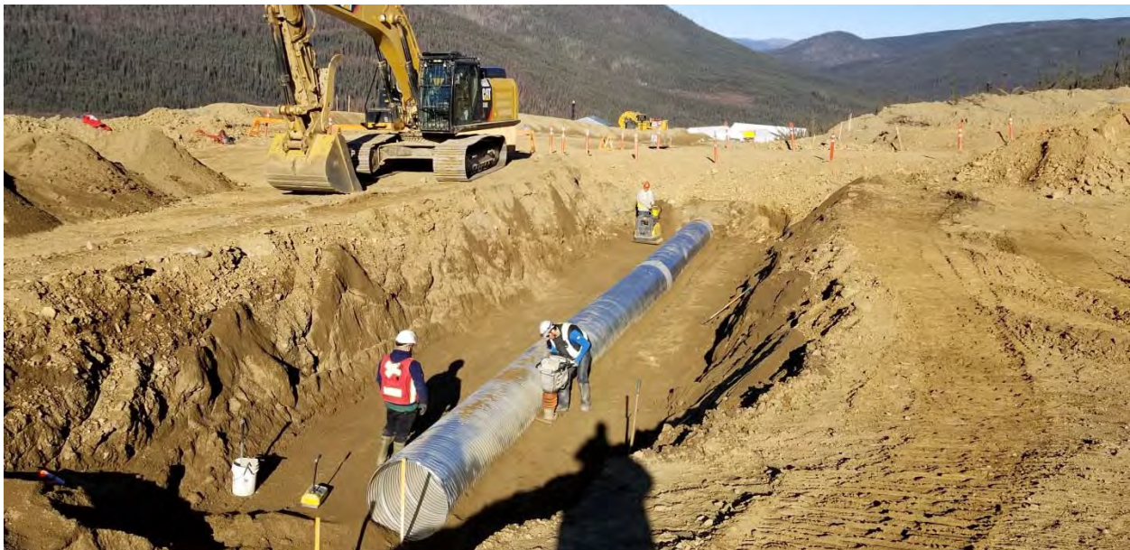
Figure 7. Placement and Compaction of 1000mm Diameter Culvert C8 Under Crusher Access Road
