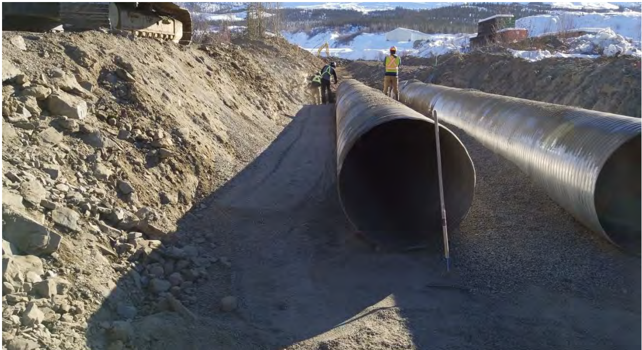
Figure 18. Ditch C Dual 1200mm Culvert Compaction and Placement near STN 0+460 Looking Upstream
