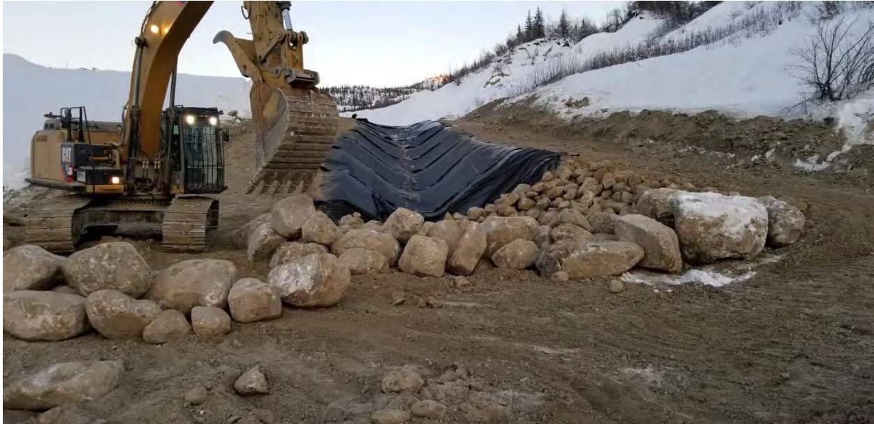
13. Ditch B Riprap Placement at Energy Dissipater in the LDSP Fore Bay
