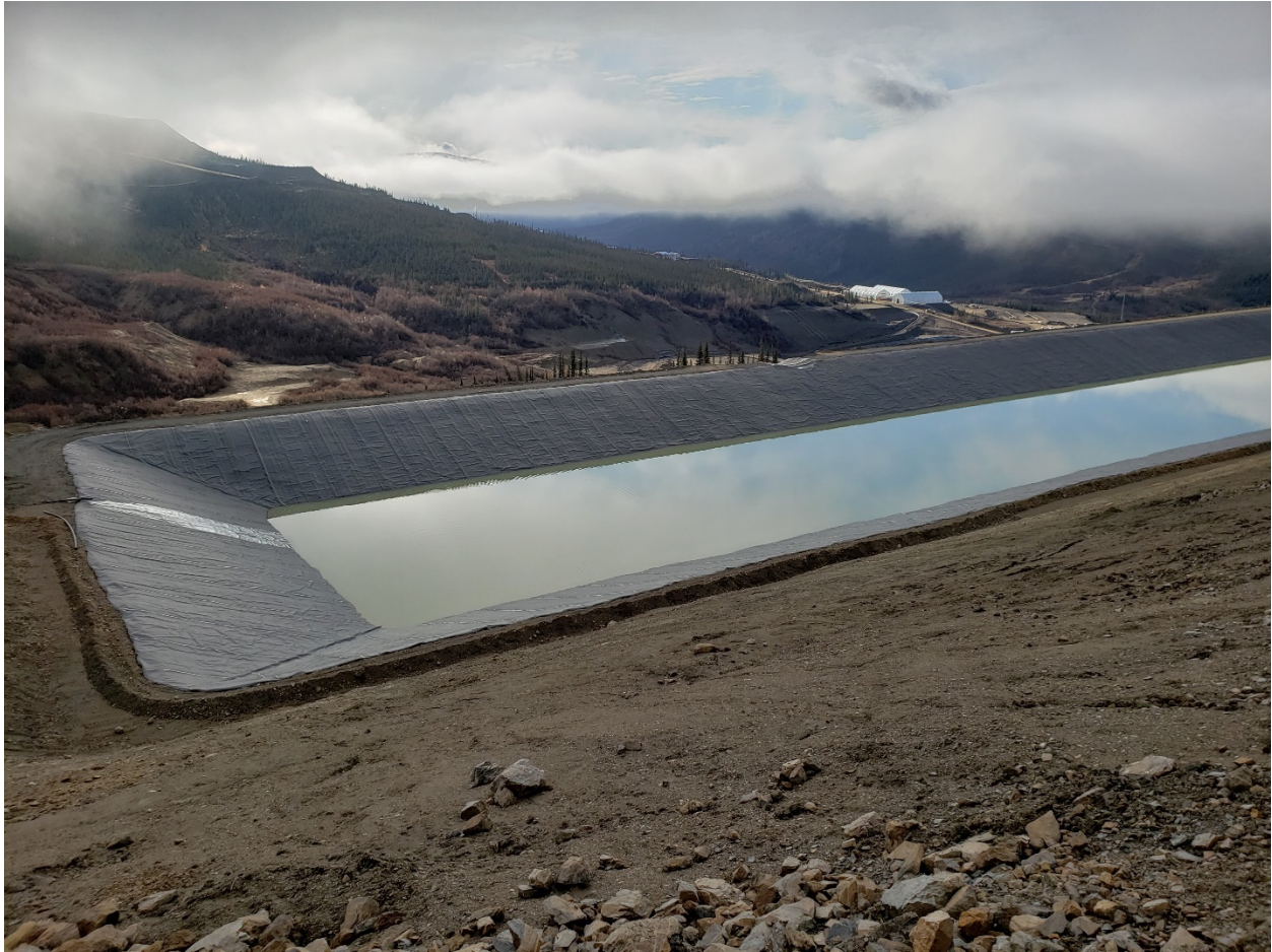
Photo 2. Event Pond looking south.
