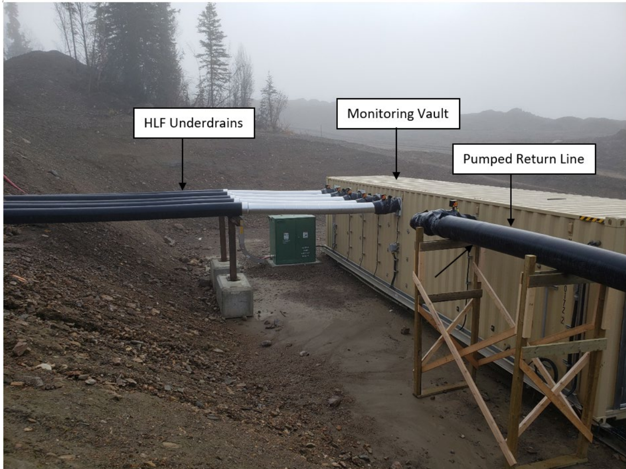
Photo 10. HLF underdrain outlet into monitoring vault looking east.
