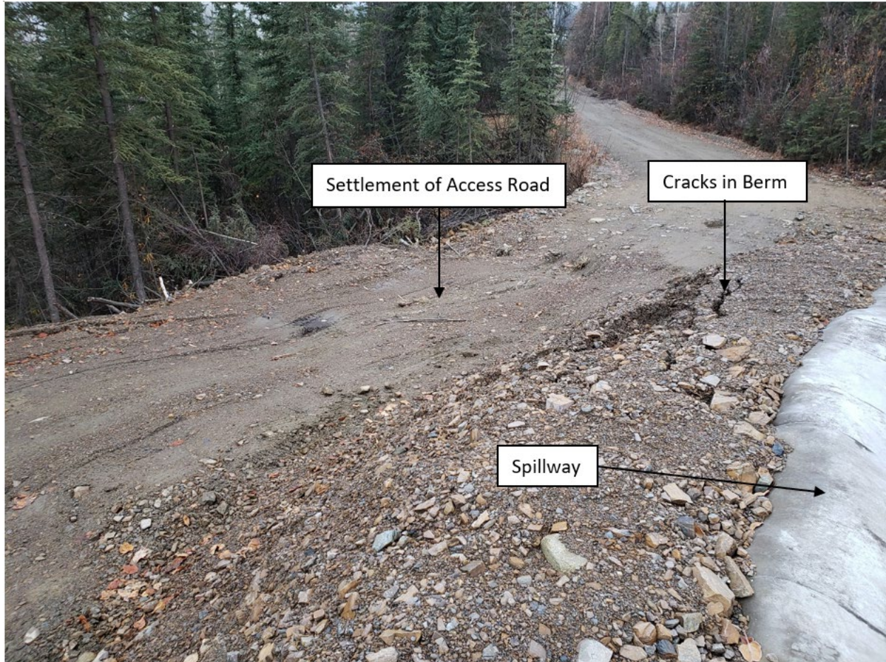
Photo 8. Berm and access road adjacent to bottom portion of Event Pond spillway.
