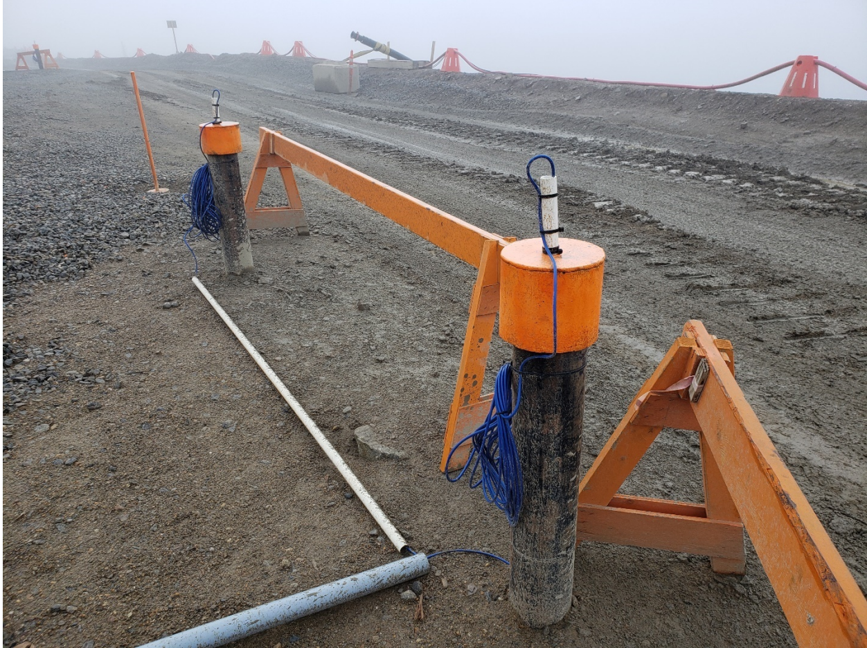
Photo 23. HLF embankment crest piezometers.
