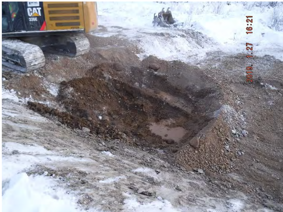
Photo 3-16: Small remaining area that needs to be scraped clean and sampled, separated by berm - January 27
