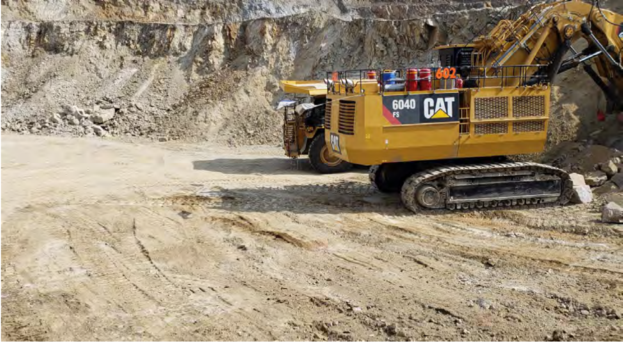
Photo 4: Spill Cleanup - July 31, 2019
