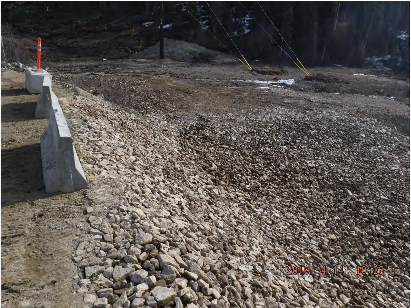
Photo 3-3: Site Stabilization with Rip Rap and View of Concrete Lock Blocks - May 14, 2019
