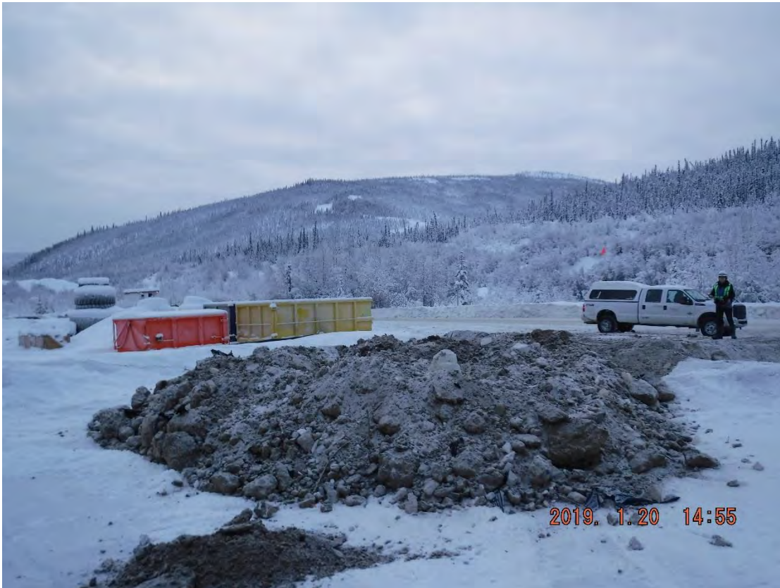
Photo 3-14: Contaminated material moved to temporary containment berm, January 20 th
