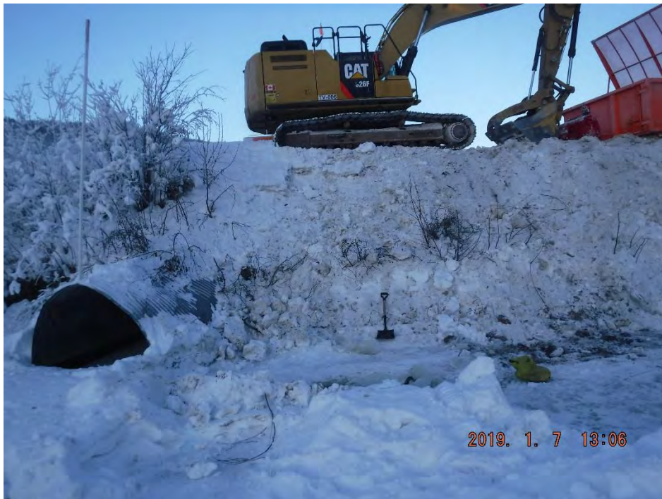
Photo 3-3: Spill Response Equipment - January 7, 2019
