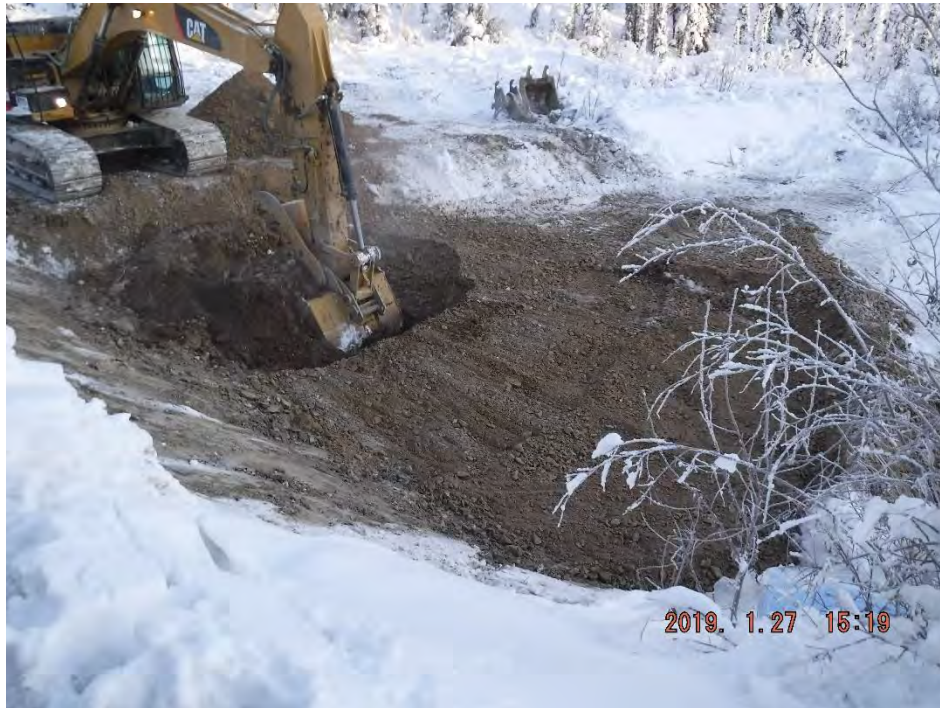
Photo 3-15: Contaminated material being scraped back and separated by “clean” berm - January 27 th
