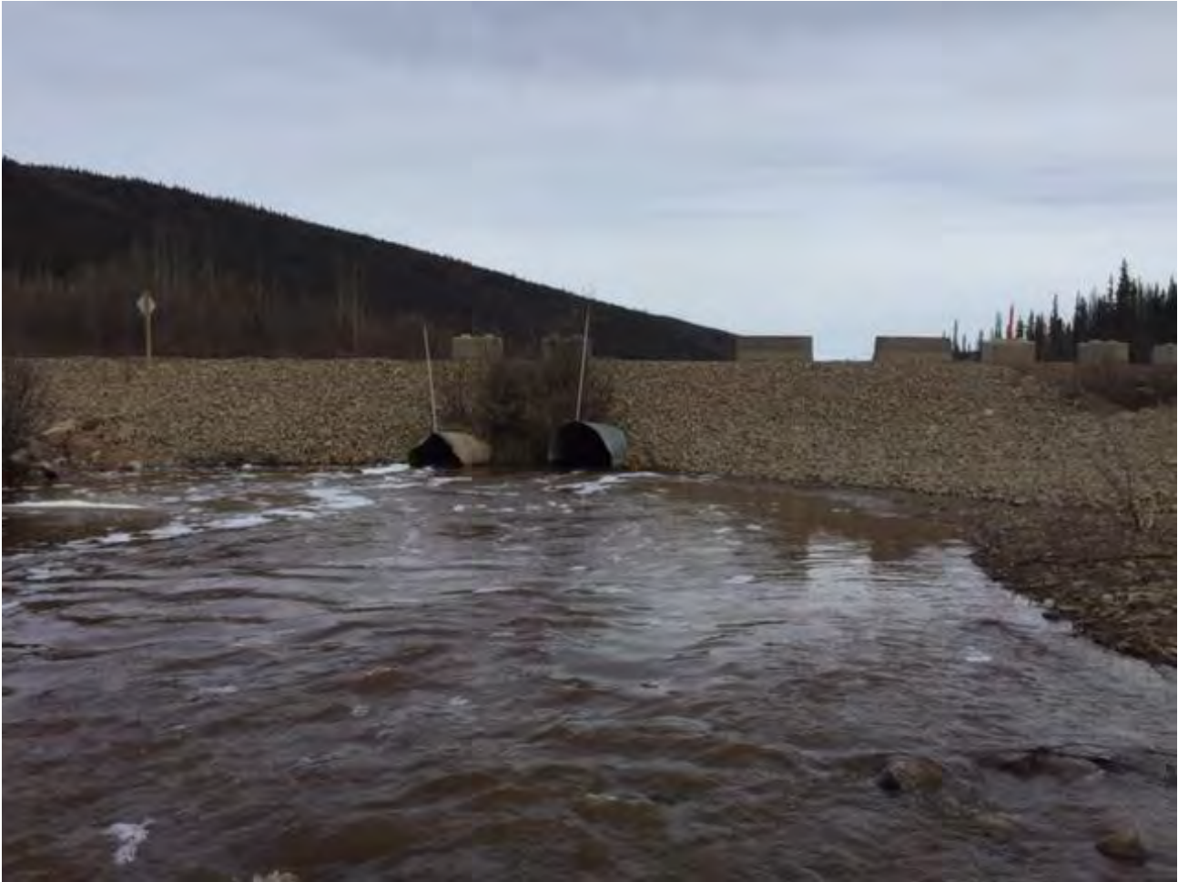
Photo 3-2: Site Stabilization with Rip Rap and View of Concrete Lock Blocks - May 10, 2019
