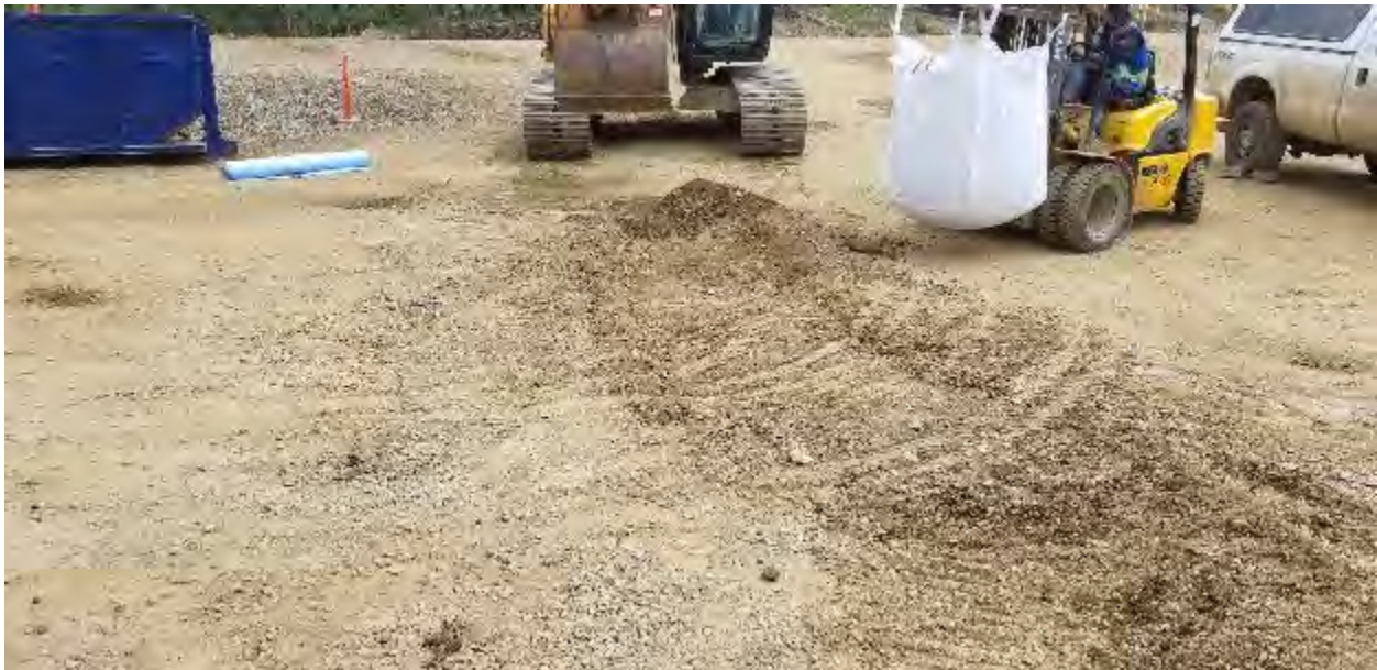
3. Excavator was used to clean up the spill and place contaminated material in super sacs
