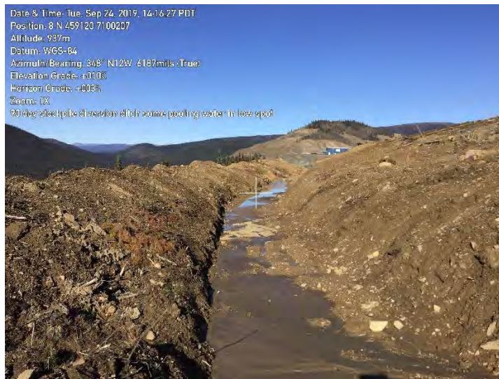
Figure 10: Pooling water in perimeter ditch
