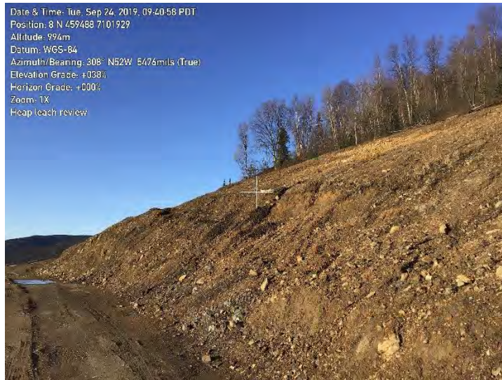
Figure 13: Noted sloughing material
