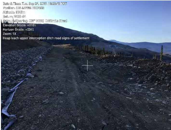
Figure 23: Road settlement along temporary access road
