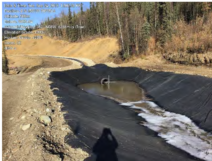
Figure 47: Flow into collection sump
