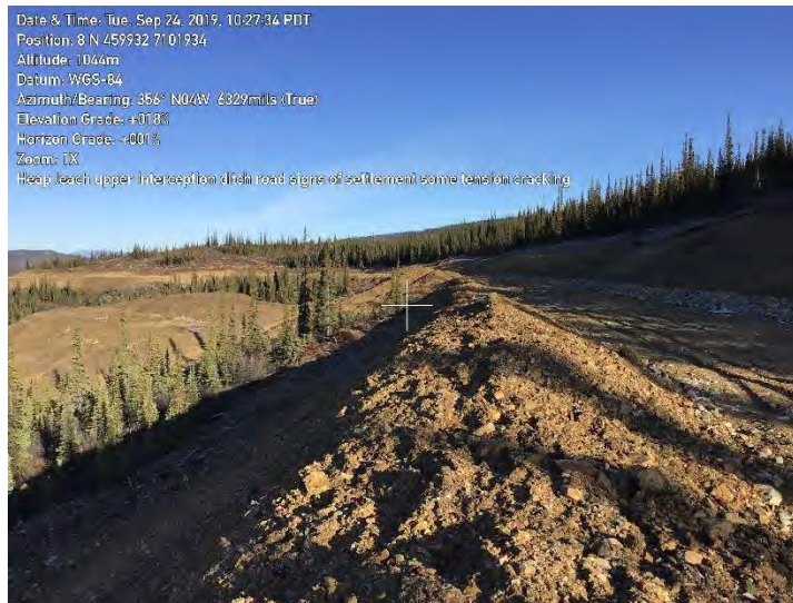
Figure 24: Downhill slope from road settlement
