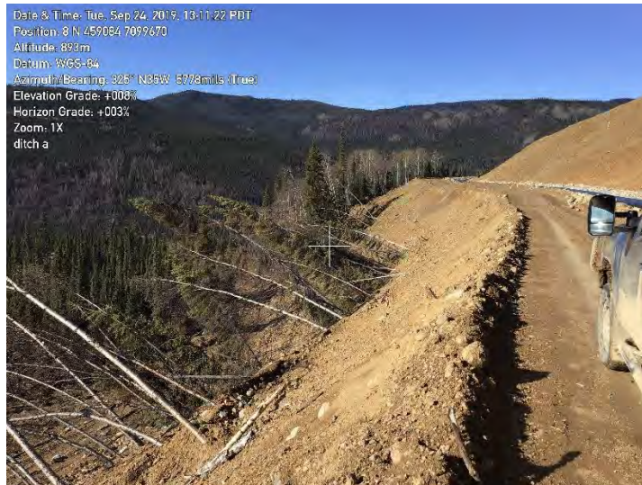
Figure 49: Trees in fill subgrade
