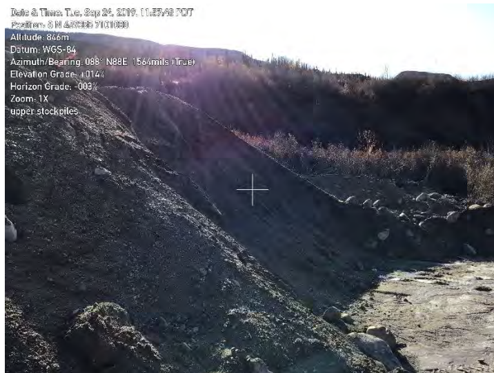
Figure 58: Some stockpiles with steep side slopes
