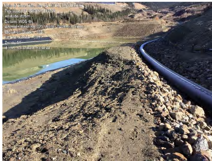
Figure 5: LDSP – Erosion on the Southwest slope
