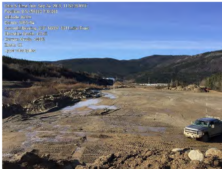
Figure 60: Ponding downhill of stockpiles
