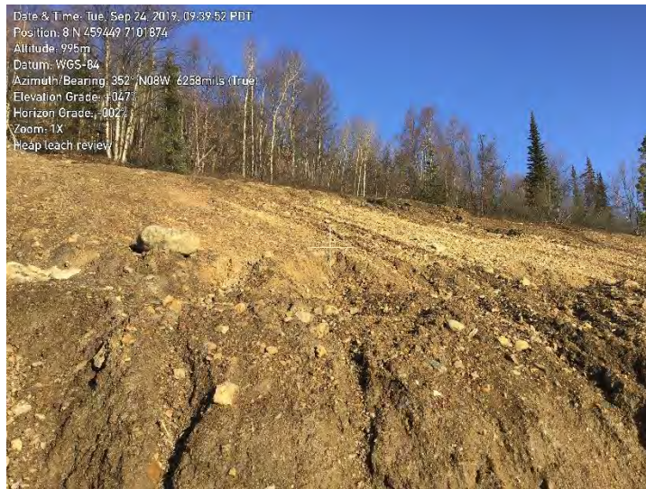
Figure 14: Some erosion on slopes
