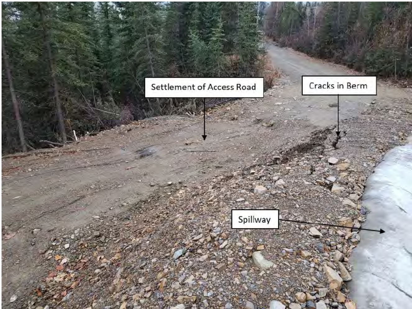
Photo 4.3-6: Berm and Access Road Adjacent to Bottom Portion of Event Pond Spillway
