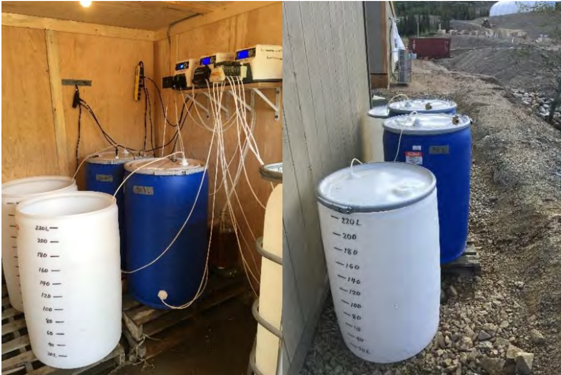
Photo 6.1-2: Bioreactor Inlet and Outlet Drums
