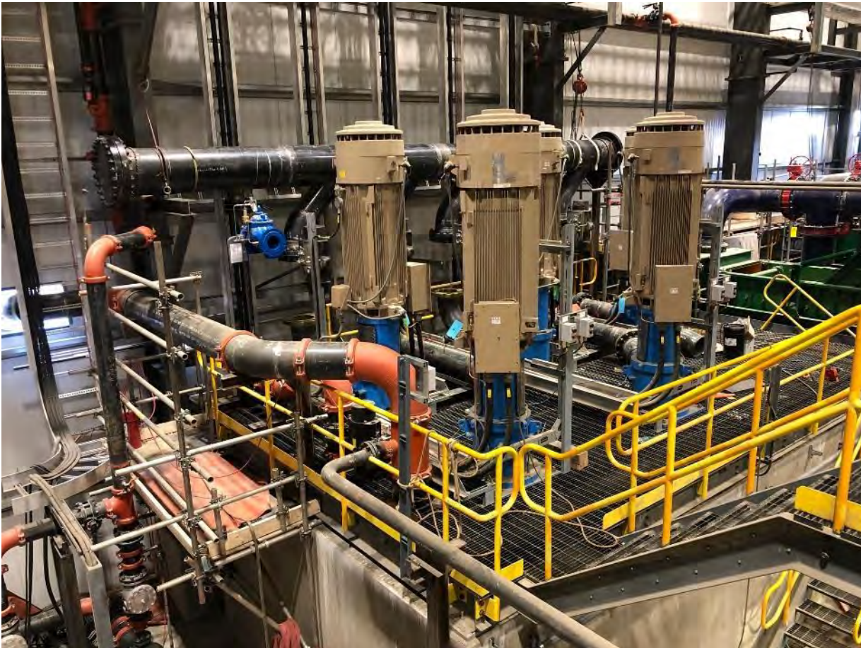
Photo 4.3-8: Barren Solution Pumps - May 7, 2019
