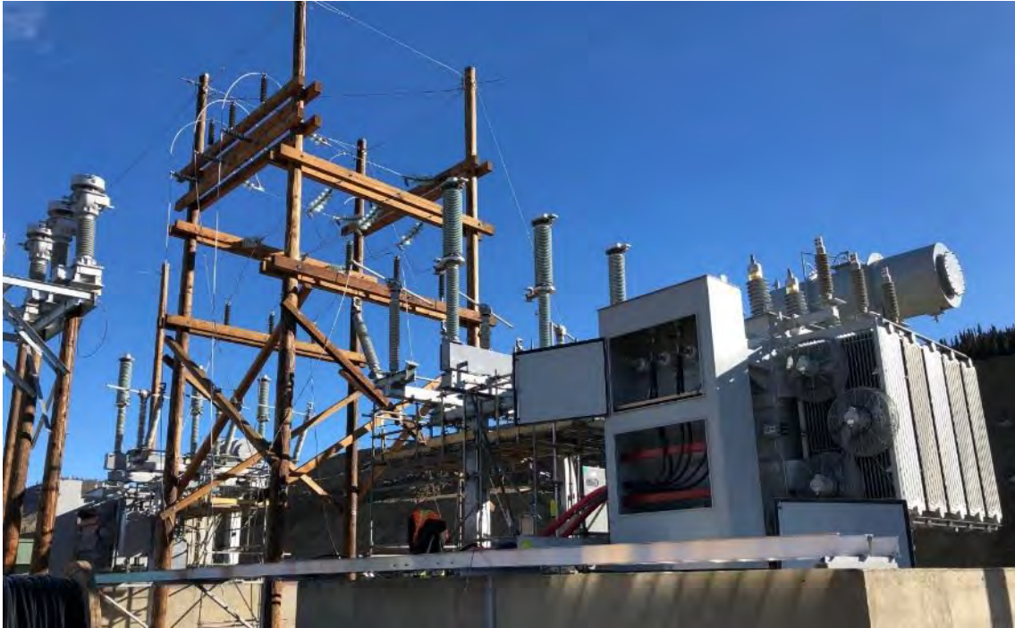
Photo 2.1-25: Site Substation - April 9, 2019
