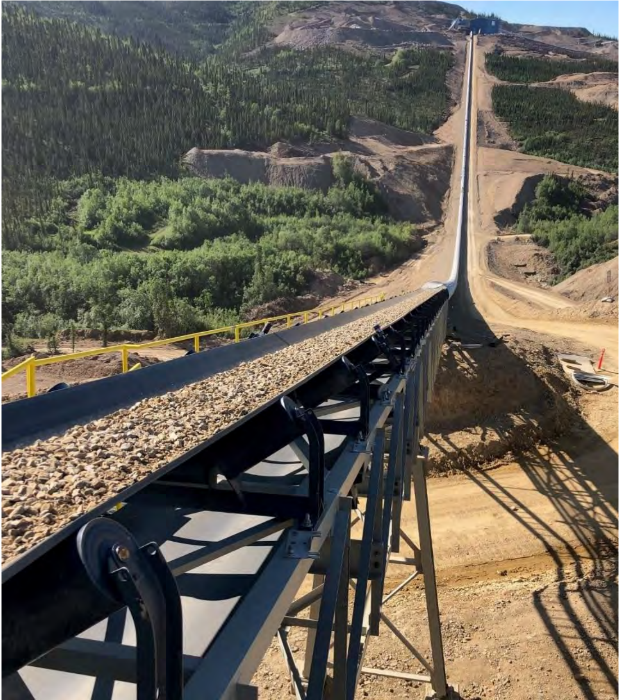
Photo 2.1-14: Overland Conveyor Operational and Conveying ODF - June 20, 2019
