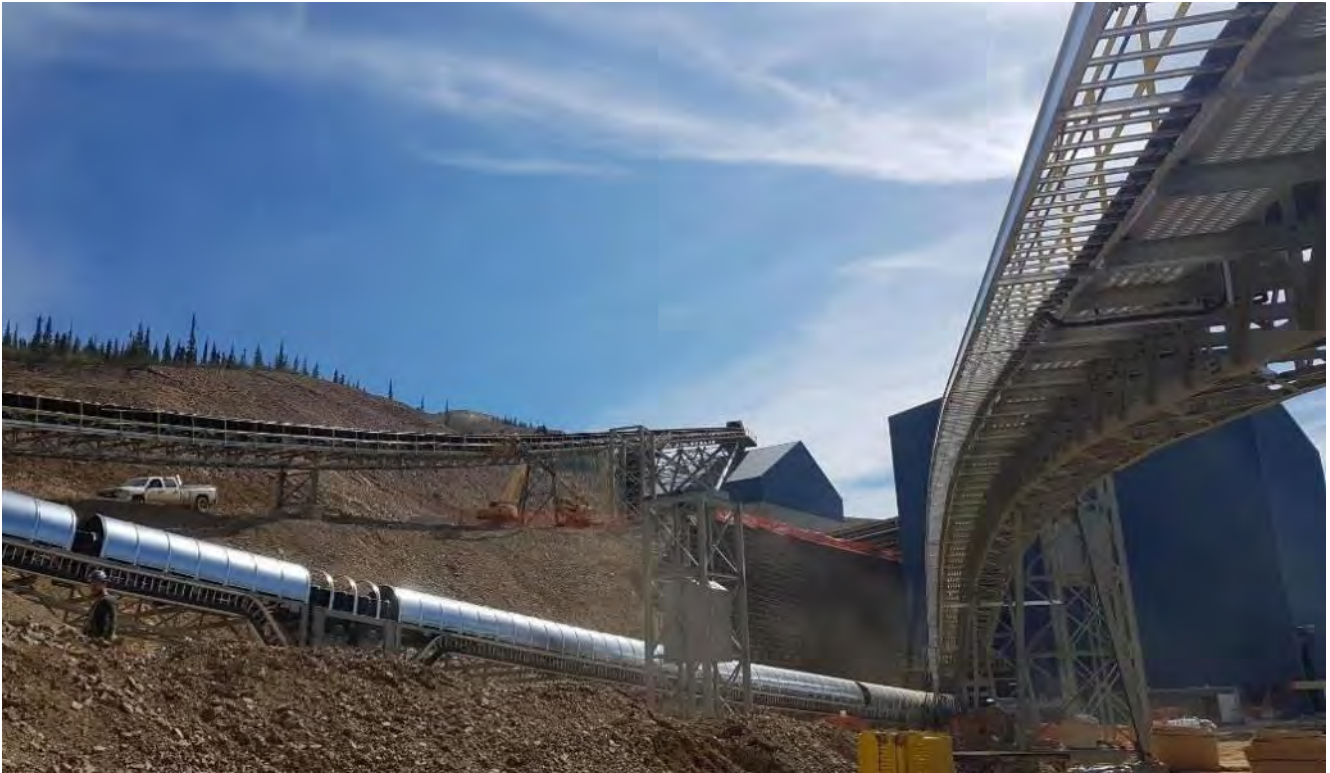
Photo 2.1-10: Secondary and Tertiary Crusher Conveyor Circuit - May 27, 2019
