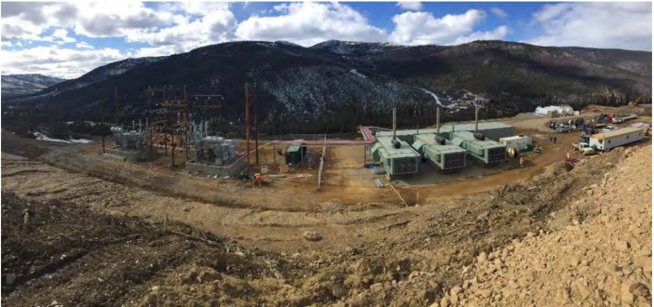
Photo 4.3-9: Project Substation and Back-Up Generators - April 11, 2019
