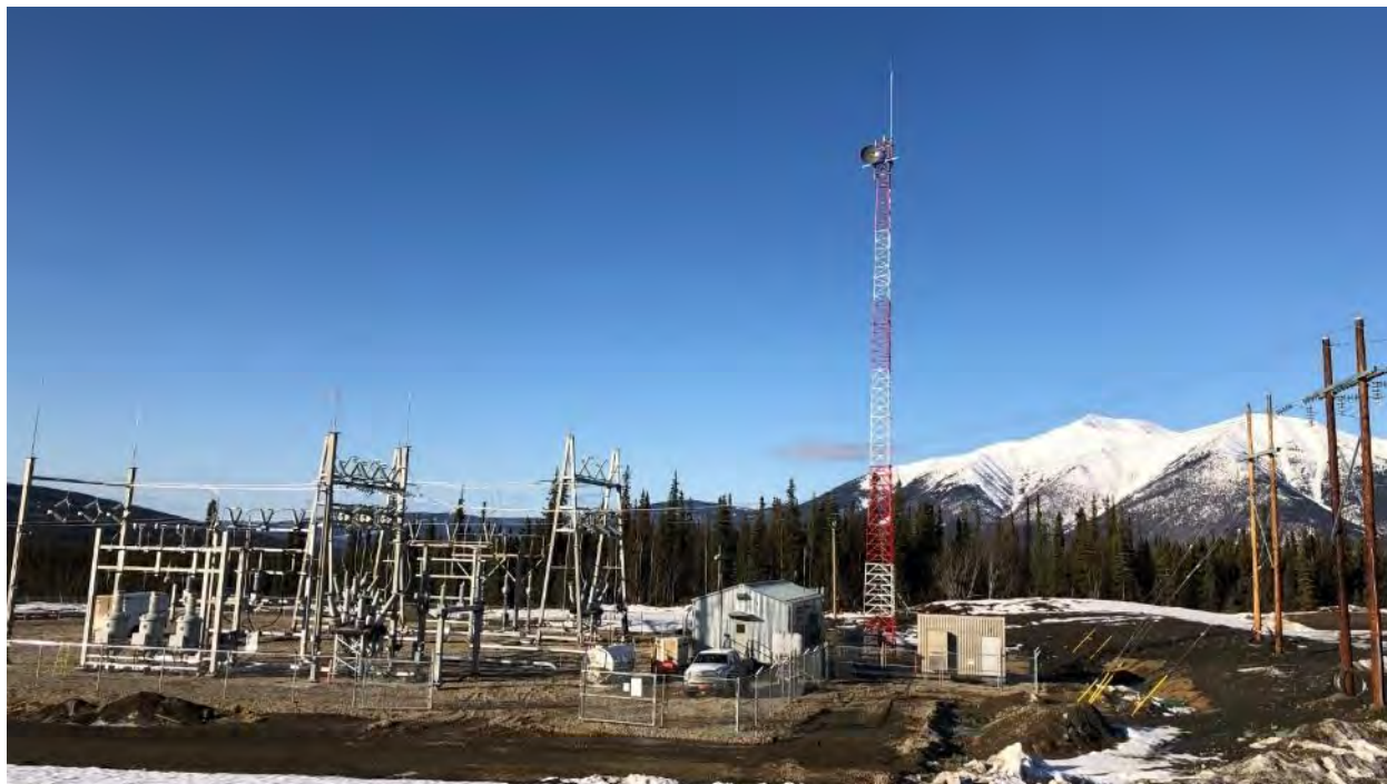
Photo 2.1-24: South McQuesten Substation - March 29, 2019
