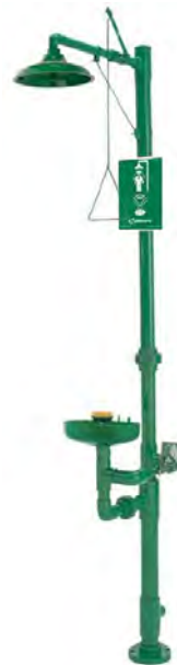
Figure 2.1-2: Typical Shower/Eyewash Station
