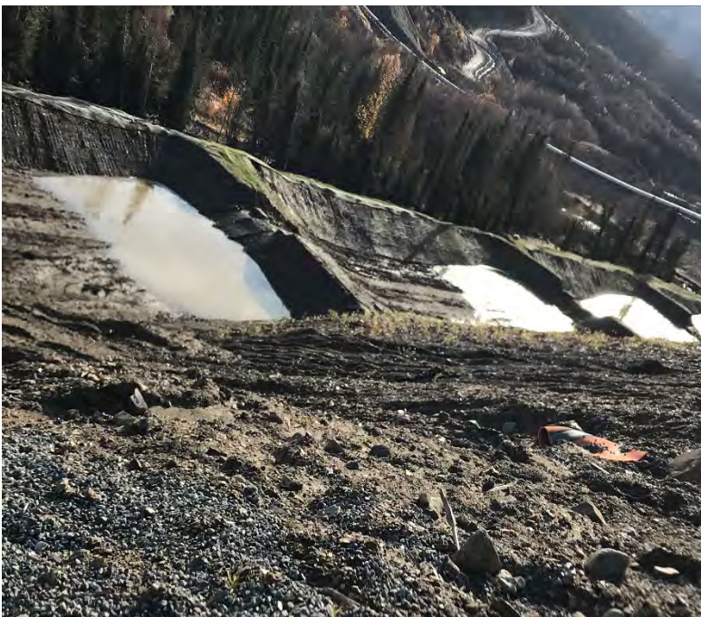
Photo 16 Sediment Control Ponds south of Eagle Pup Waste Rock Storage Area and Dublin Gulch
