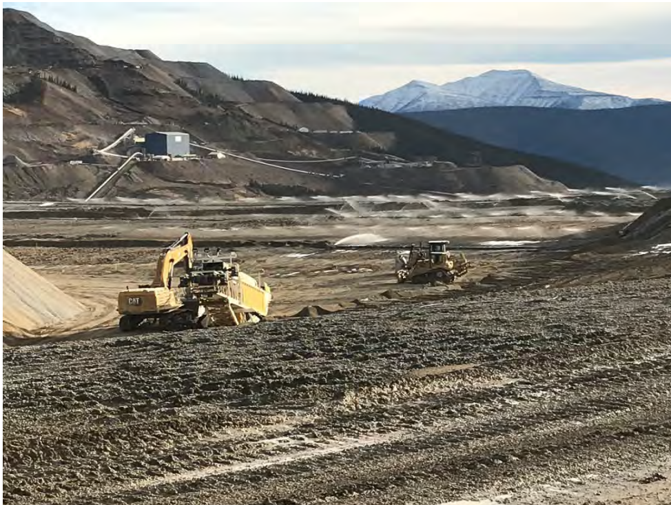
Photo 24 Heap Leach Facility (HLF) Phase 1 – Note Sprinklers in HLF, and Primary Crusher in Background
