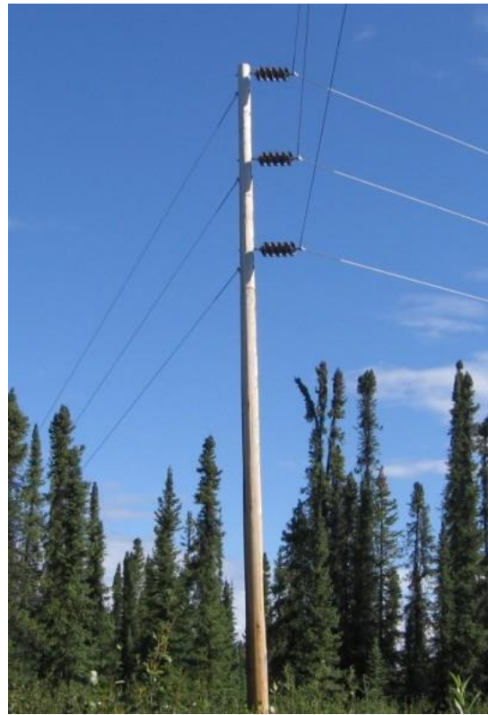
Photo 6.9-2: Typical Running Angle Pole
