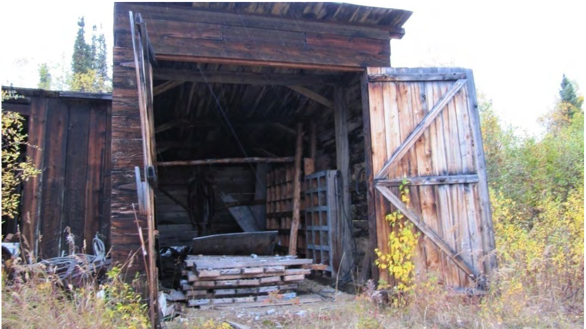
Plate 13: Site 1, view east showing interior view of the larger of two plank shacks [4]
