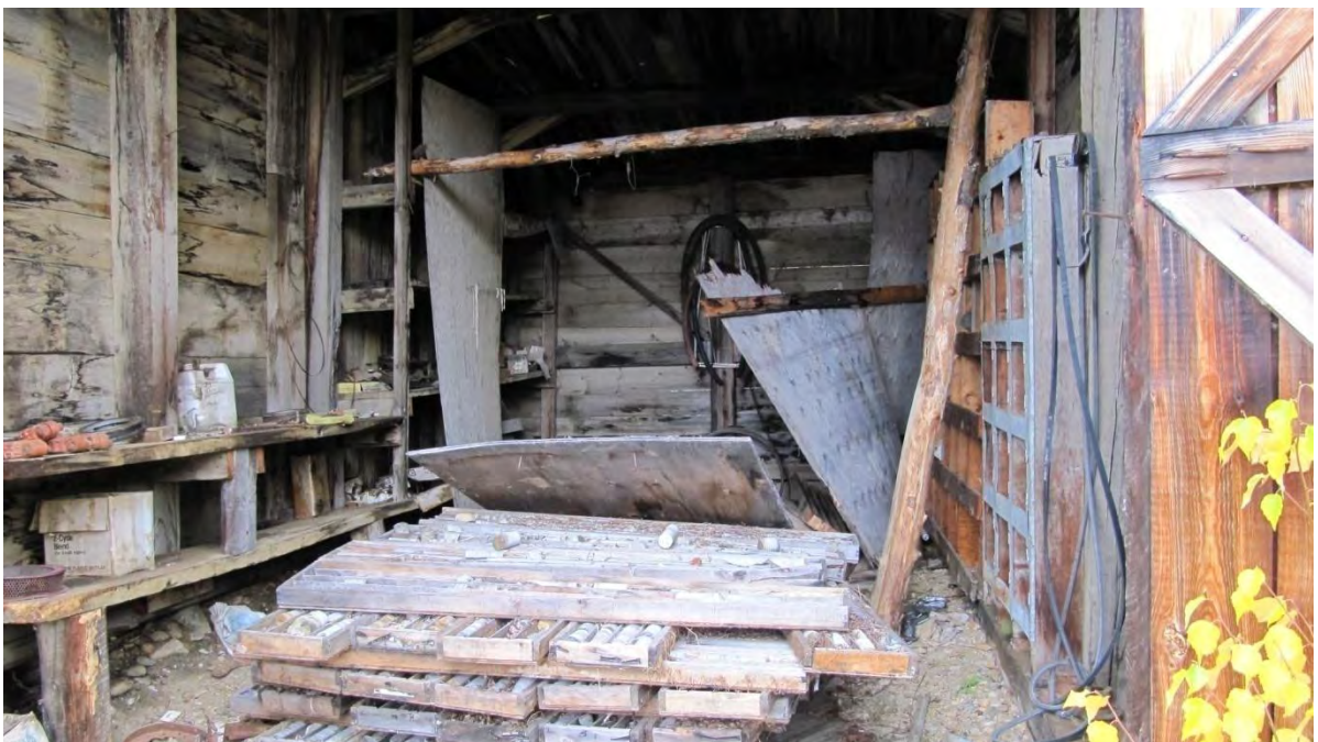
Plate 14: Site 1, view east showing detail of the interior of the larger of two plank shacks [4]
