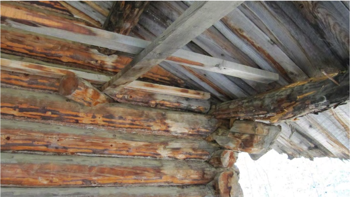
Plate 29: Site 2 structure, view northwest of roof and exterior wall detail at front of building
