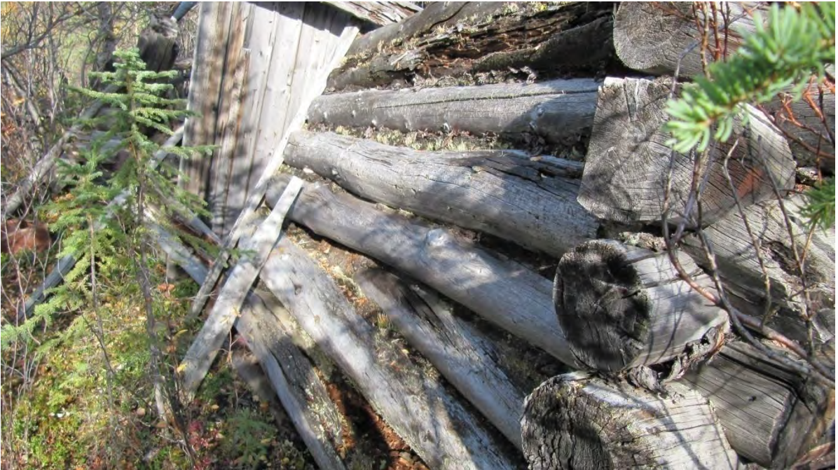
Plate 37: Site 3 structure, view northeast showing construction detail of west wall and southwest corner
