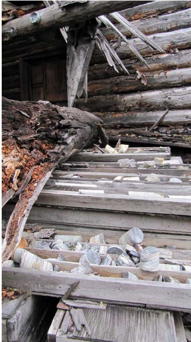
Plate 10: Site 1, view southeast of the interior of log structure [7], showing collapsed roof and recent (1970s) use of the cabin for core storage
