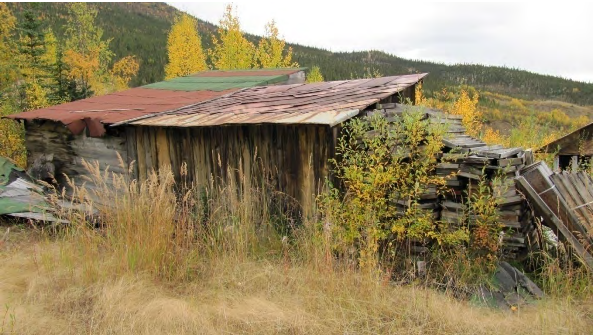
Plate 12: Site 1, view southwest showing the back side and partial metal roof of the plank structures [4]
