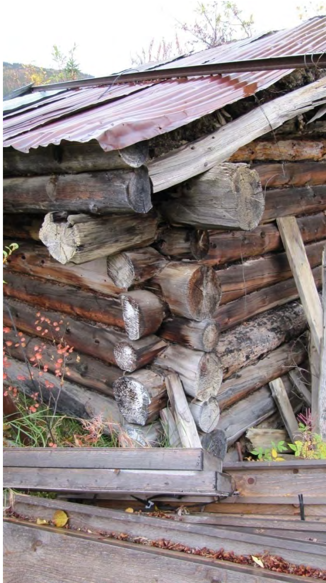
Plate 3: Site 1, close view of log structure [2] construction, view southwest of back corner
