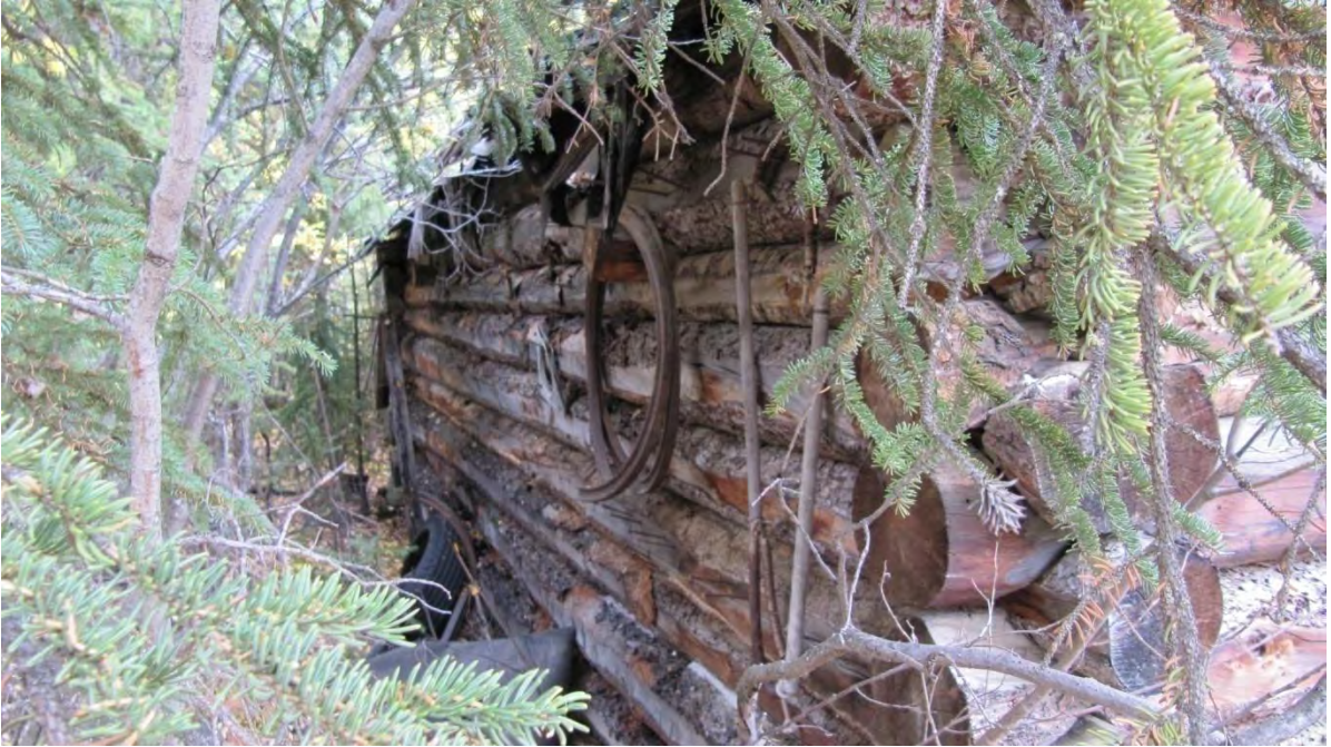
Plate 9: Site 1, view south of the east exterior wall of log structure [7] showing construction detail
