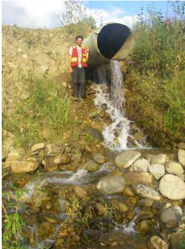
Photo 3-3: Culvert barrier on lower Eagle Pup, photo taken facing upstream on August 15, 2008
