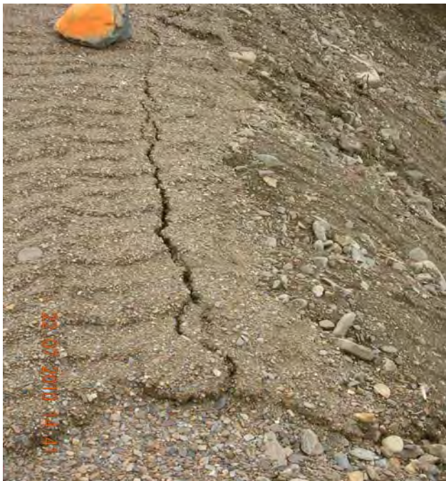
Photograph 2 Secret Creek - Fill failing
