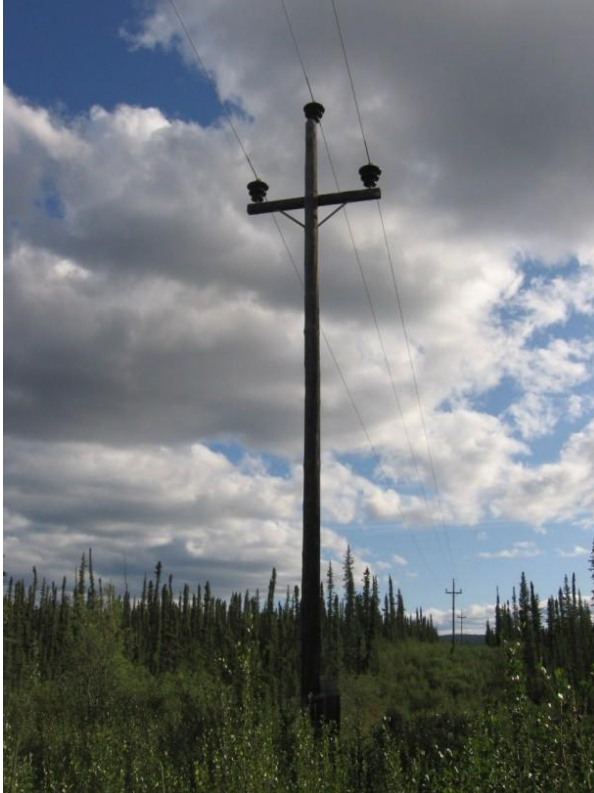
Photo 4.4-1: Typical Tangent Pole
