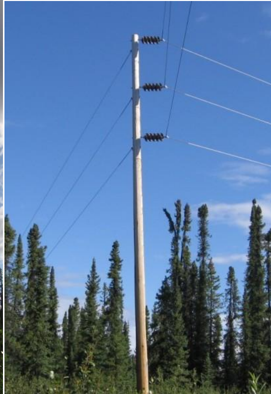
Photo 4.4-2: Typical Running Angle Pole
