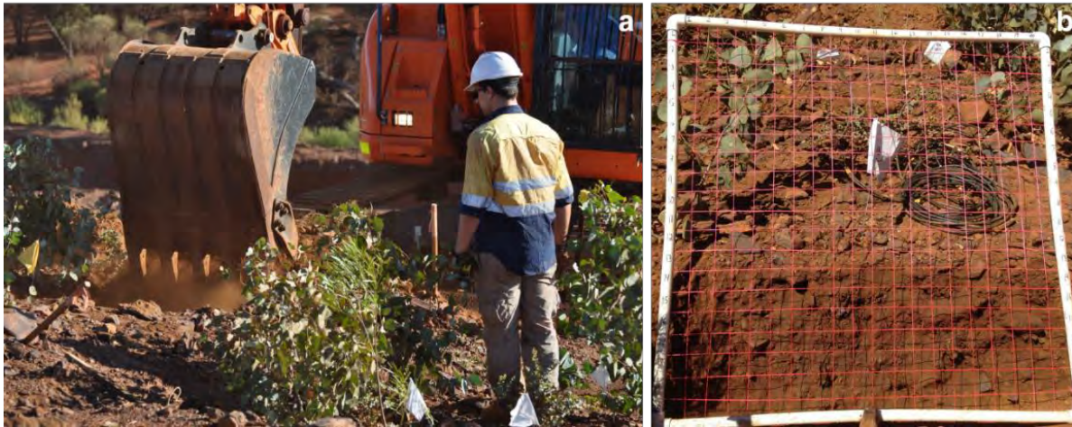
Figure 2.1-1: Creation of pit into a cover system with established vegetation to quantify root depths, distribution, and material textures
