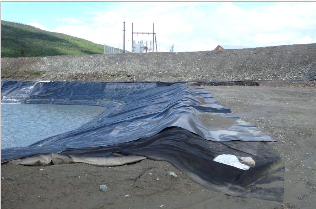
Photo 16: Incomplete liner anchoring trench at east end of mill water storage pond (Facing north – July 28, 2011)
