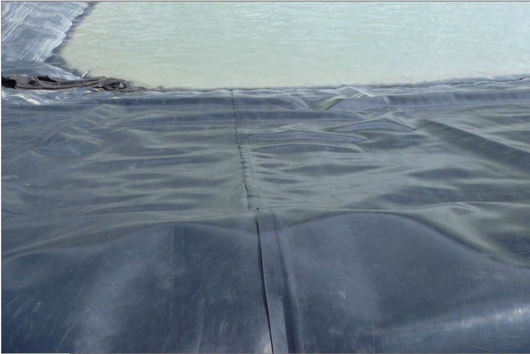
Photo 15: Typical seam in liner of mill water storage pond (Facing east – July 28, 2011)
