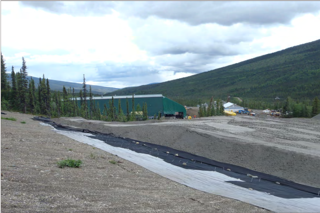
Photo 17: Gravel drainage blanket, geosynthetic clay liner, geonet, geotextile, and tailings placed within the DSTF (Facing south – July 28, 2011)
