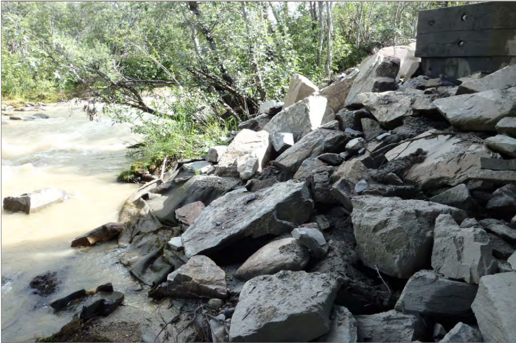
Photo 13: Exposed geotextile on south bank of Lightning Creek requiring additional riprap placement (Facing east – July 28, 2011)
