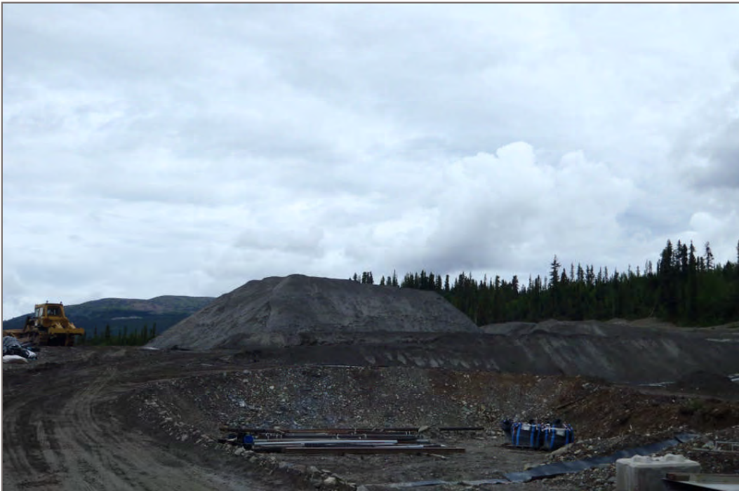
Photo 18: Existing pile crest exceeds design elevation; the pile should be reshaped to design dimensions (Facing north – July 28, 2011)
