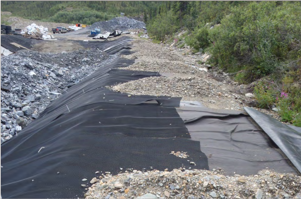
Photo 5: Loose material piled on top of west berm to hold liner in place (Facing south – July 28, 2011)
