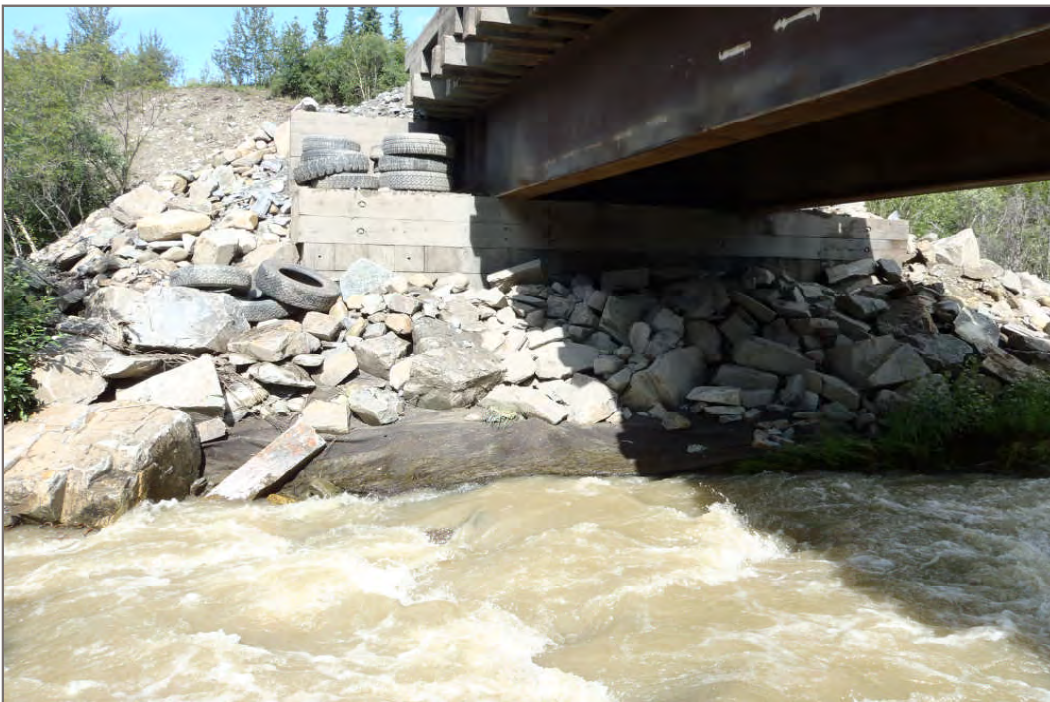
Photo 12: Exposed geotextile on north bank of Lightning Creek requiring additional riprap placement (Facing north – July 28, 2011)
