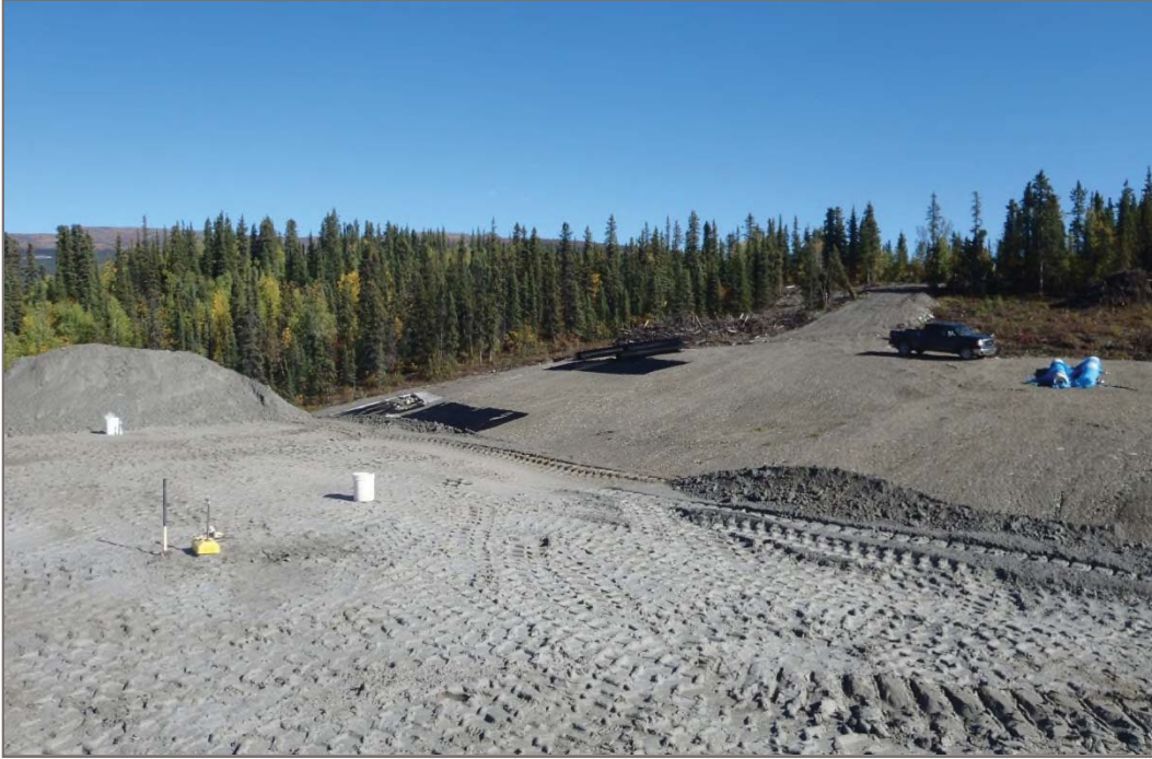
Photo 27: Dry Stacked Tailings Facility Compaction testing at the dry stacked tailings facility Facing north – September 10, 2013
