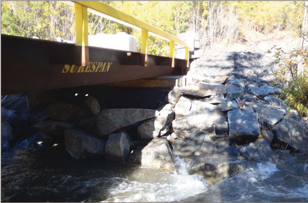
Photo 15: Lightning Creek Bridge Abutments (Onek Road) Rip-rap armoring providing erosion protection for bridge abutments Facing north – September 10, 2013
