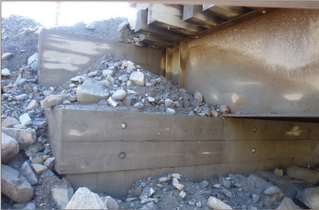
Photo 17: Lightning Creek Bridge Abutments (Bellekeno Road) Earth filled timber cribbing bridge abutments Facing east – September 10, 2013
