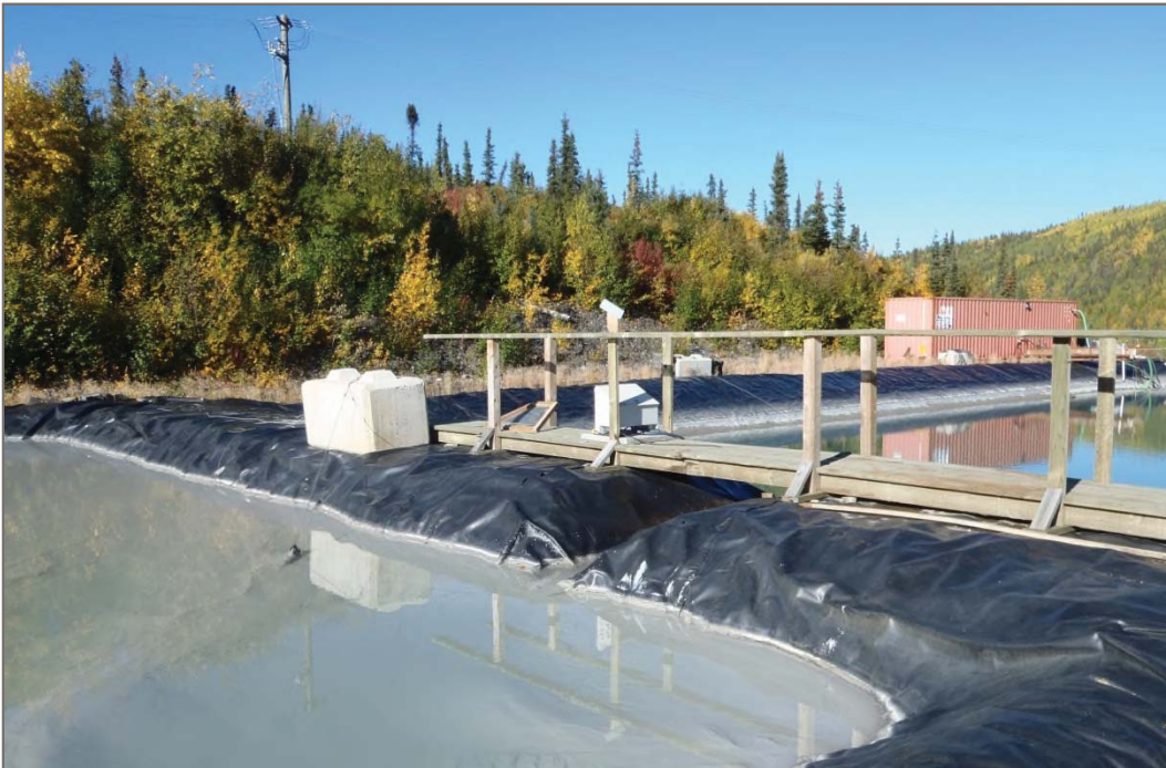
Photo 6: Bellekeno 625 Water Treatment Ponds Approximately 0.5 m freeboard in pond one Facing west – September 10, 2013
