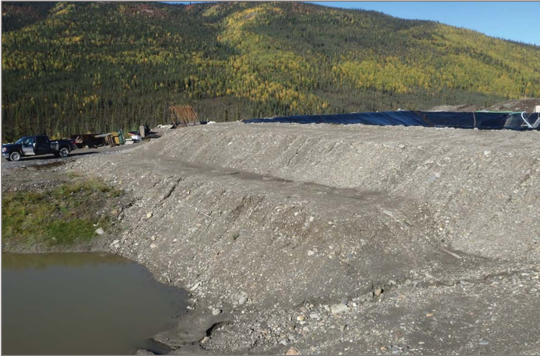
Photo 21: Mill Water Storage Pond Minor erosion observed on exterior of perimeter berm on south and west sides Facing west – September 10, 2013
