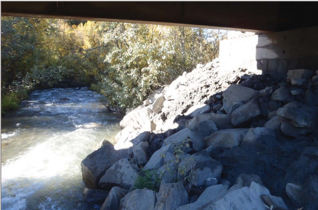
Photo 18: Lightning Creek Bridge Abutments (Bellekeno Road) Rip-rap armoring providing erosion protection for bridge abutments Facing south – September 10, 2013
