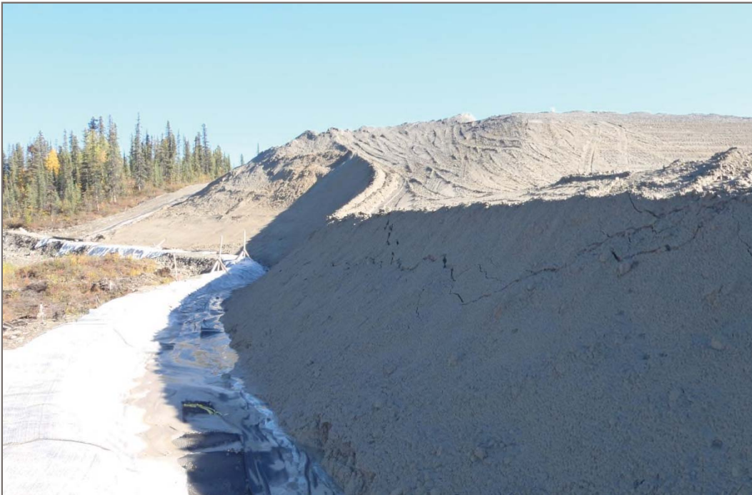
Photo 26: Dry Stacked Tailings Facility Minor tension cracking on north side of facility Facing east – September 10, 2013
