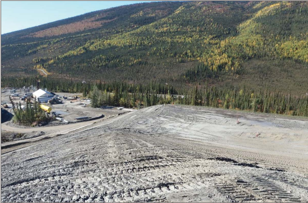
Photo 23: Dry Stacked Tailings Facility Contouring of facility to design grades Facing west – September 10, 2013
