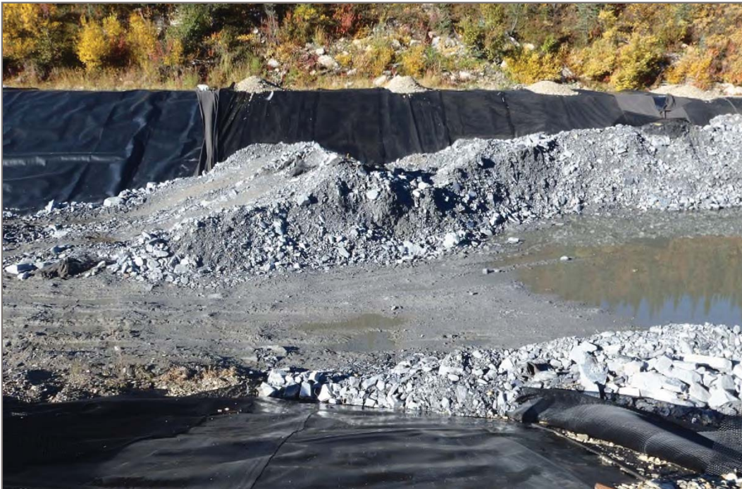
Photo 4: PAG Waste Storage Facility Angular waste material in direct contact with liner Facing west – September 10, 2013
