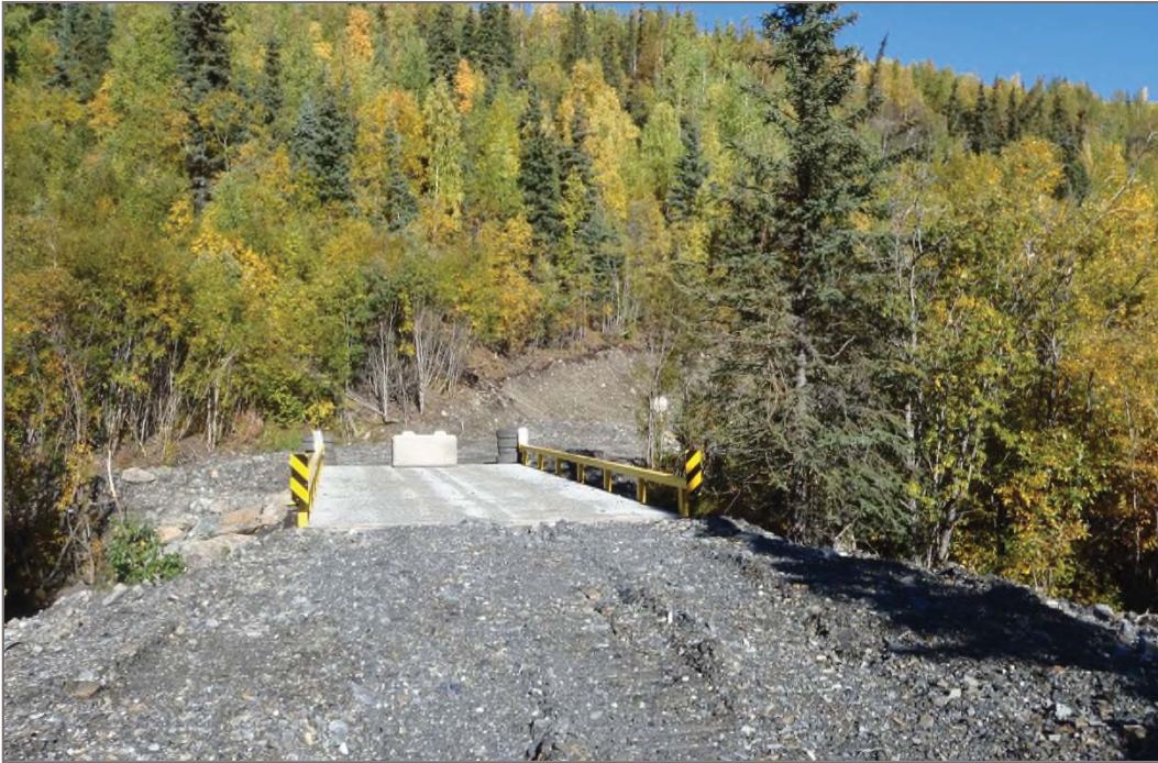
Photo 13: Lightning Creek Bridge Abutments (Onek Road) Lightning Creek Bridge on the Onek Road Facing north – September 10, 2013
