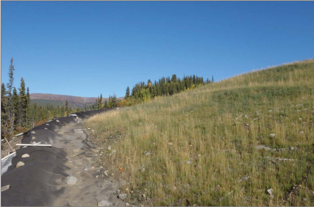
Photo 25: Dry Stacked Tailings Facility Perimeter berm and surface water collection system Facing north – September 10, 2013
