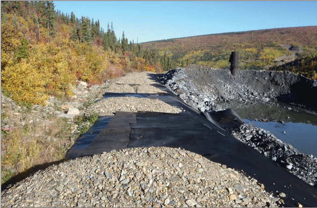
Photo 3: PAG Waste Storage Facility Liner not properly anchored around north and west perimeter Facing north – September 10, 2013
