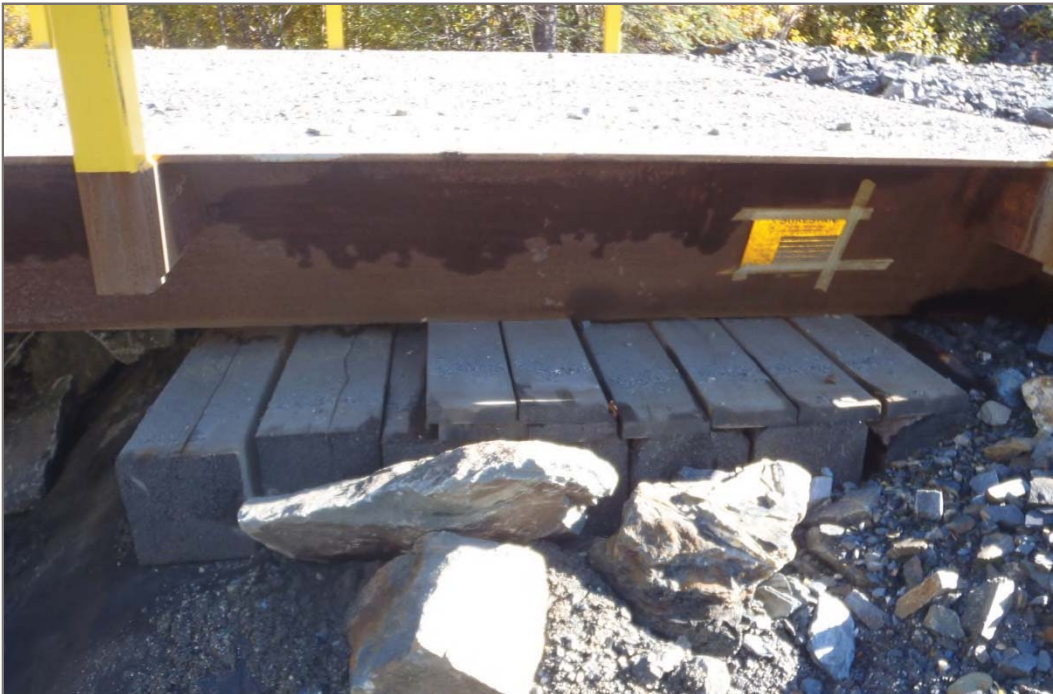
Photo 14: Lightning Creek Bridge Abutments (Onek Road) Compacted earth fill and wooden timber bridge abutments Facing east – September 10, 2013
