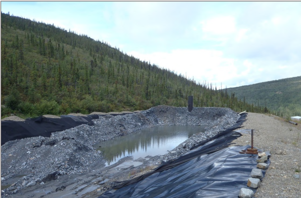
Photo 2: PAG Waste Storage Facility Surface water in facility Facing north – August 12, 2014
