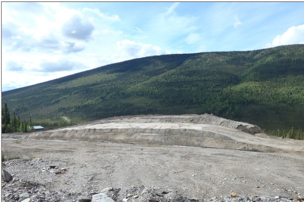
Photo 24: Dry Stacked Tailings Facility Top of facility where tailings placement will continue Facing west – August 13, 2014
