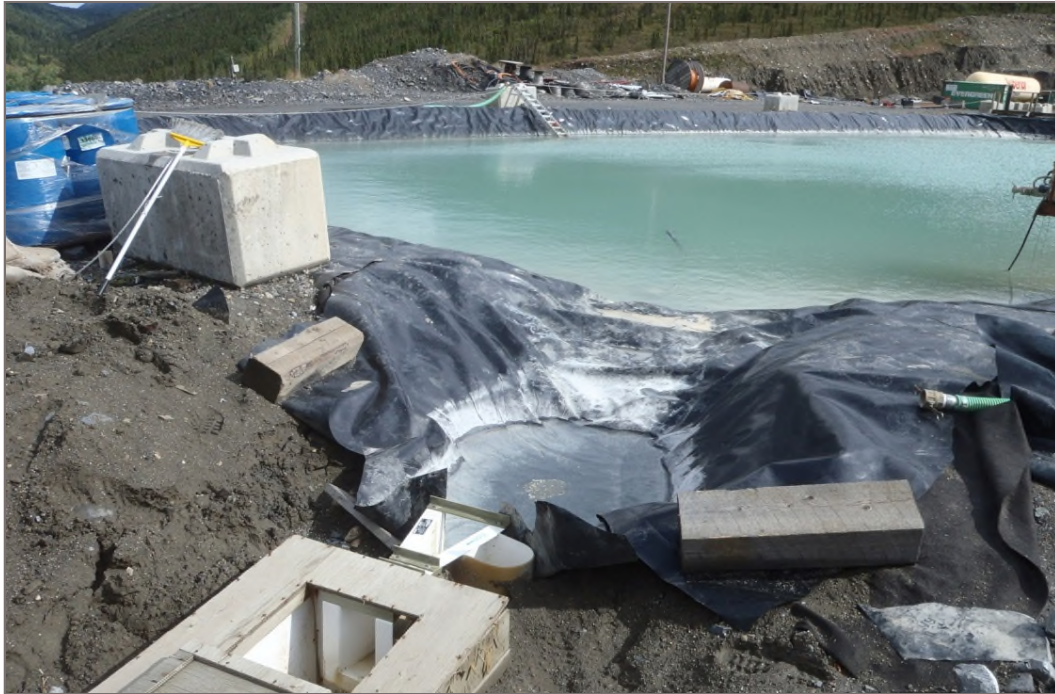
Photo 9: Bellekeno 625 Water Treatment Ponds Freeboard in secondary pond at outlet location Facing east – August 12, 2014
