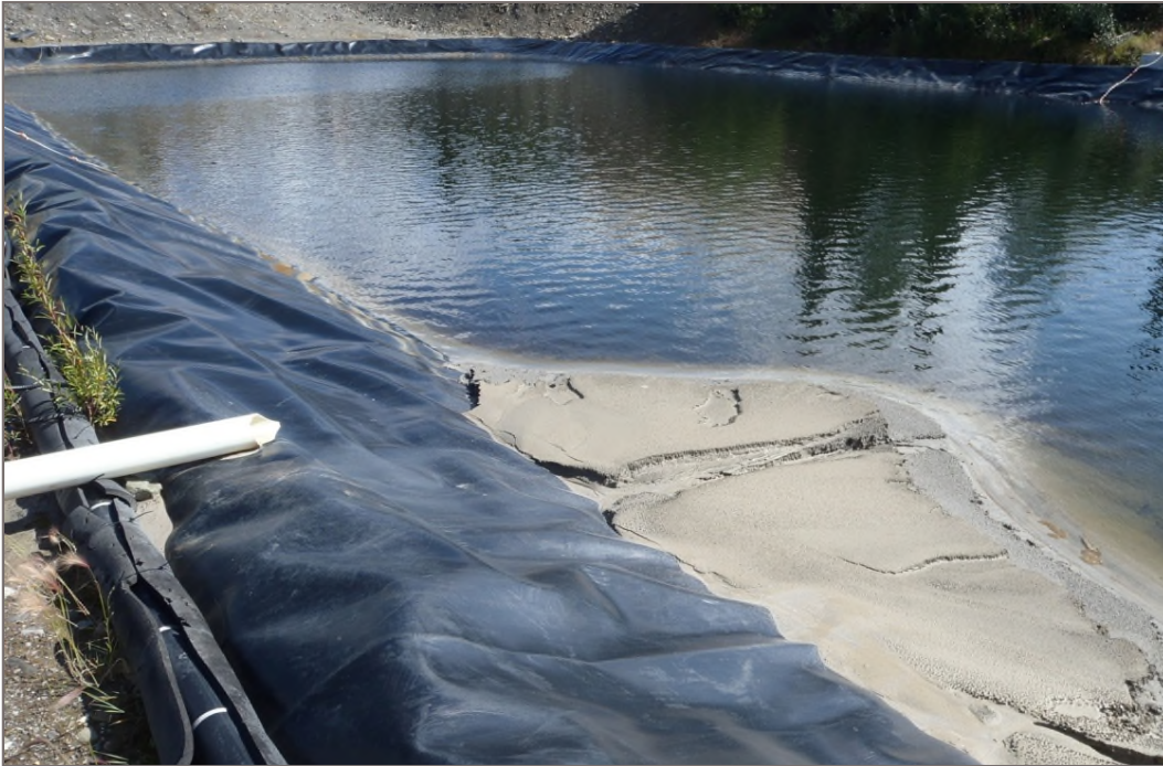
Photo 21: Mill Water Storage Pond Sediment deposited at inlet from DSTF surface water collection system Facing east – August 13, 2014
