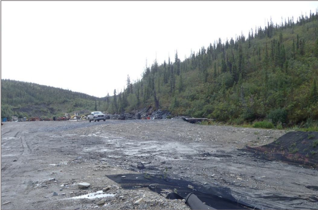
Photo 3: PAG Waste Storage Facility Laydown area graded toward facility entrance Facing south – August 12, 2014
