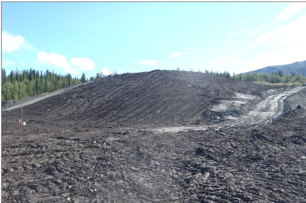
Photo 23: Dry Stacked Tailings Facility Progressive reclamation of upper bench (cover and seed mixture applied) Facing east – August 13, 2014
