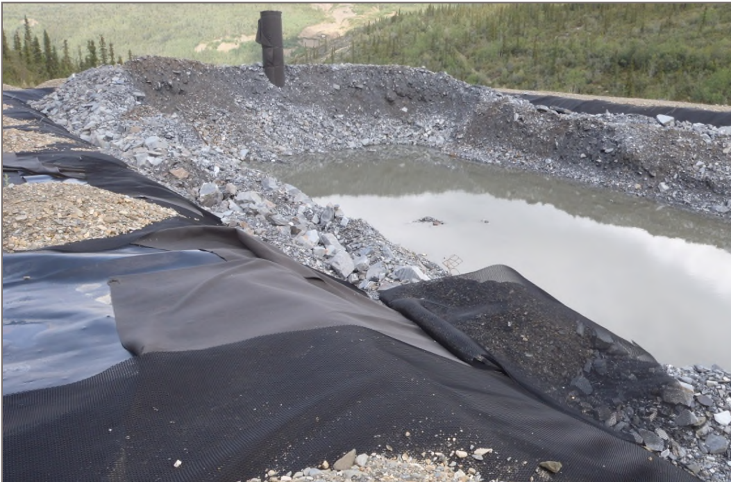
Photo 4: PAG Waste Storage Facility Liner components displaced due to wind Facing east – August 12, 2014
