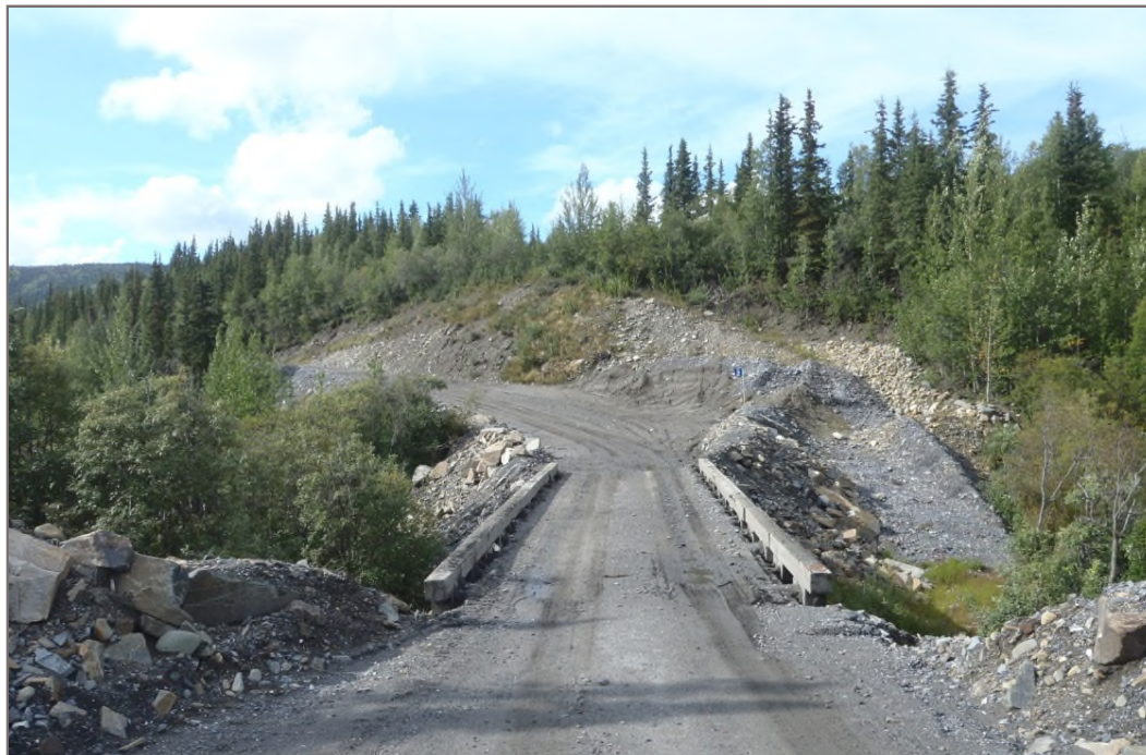
Photo 16: Lightning Creek Bridge Abutments (Bellekeno Haul Road) Bridge overview Facing west – August 12, 2014
