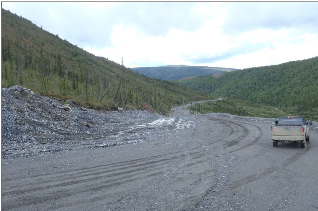
Photo 12: Bellekeno Waste Rock Pile Surface water and erosion on roadway Facing west – August 12, 2014
