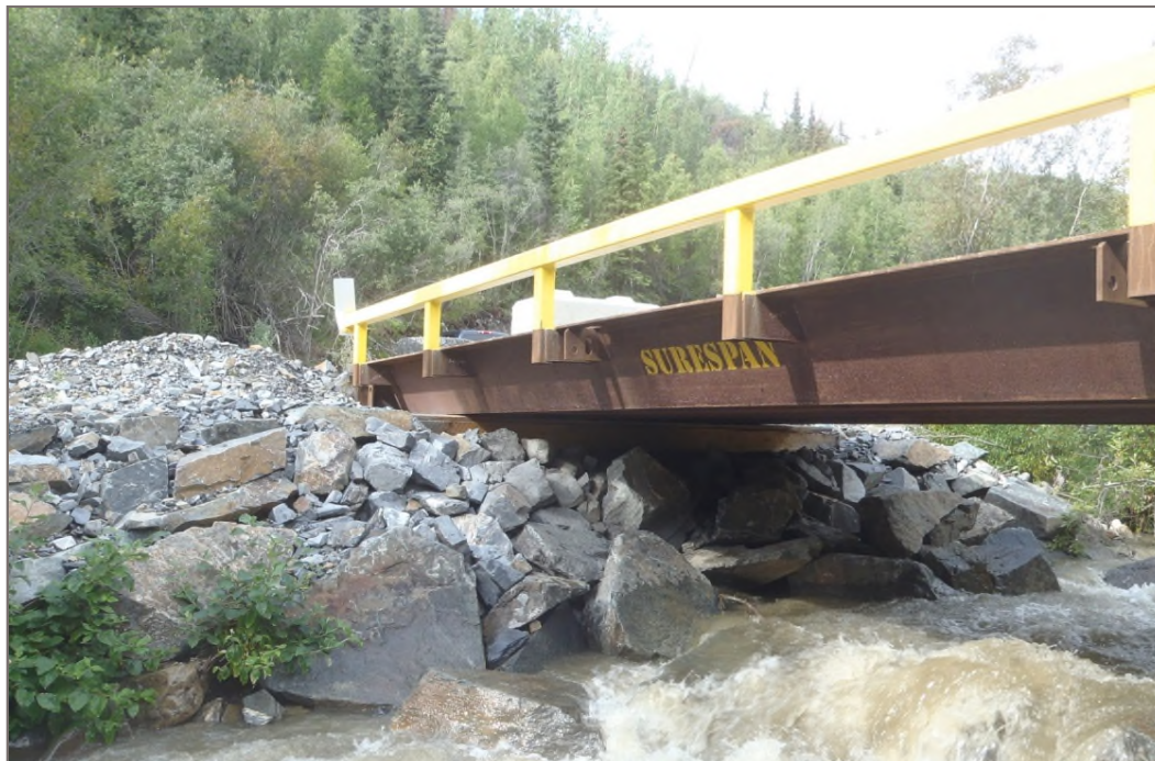
Photo 15: Lightning Creek Bridge Abutments (Onek Road) Rip-rap armouring bridge abutments Facing north – August 12, 2014
