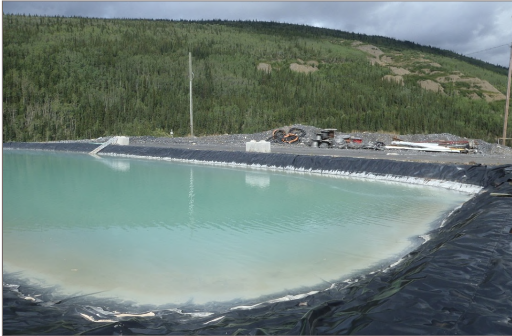
Photo 7: Bellekeno 625 Water Treatment Ponds Intact perimeter berms and liners Facing east – August 12, 2014
