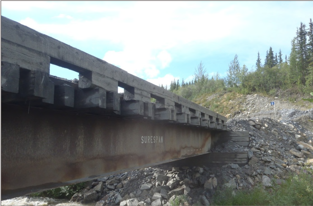
Photo 17: Lightning Creek Bridge Abutments (Bellekeno Haul Road) Stable earth filled timber abutments Facing west – August 12, 2014
