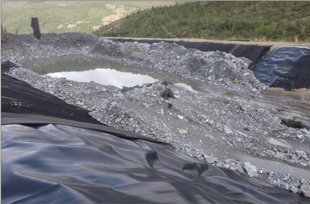
Photo 5: PAG Waste Storage Facility Angular waste rock in direct contact with liner Facing east – August 12, 2014
