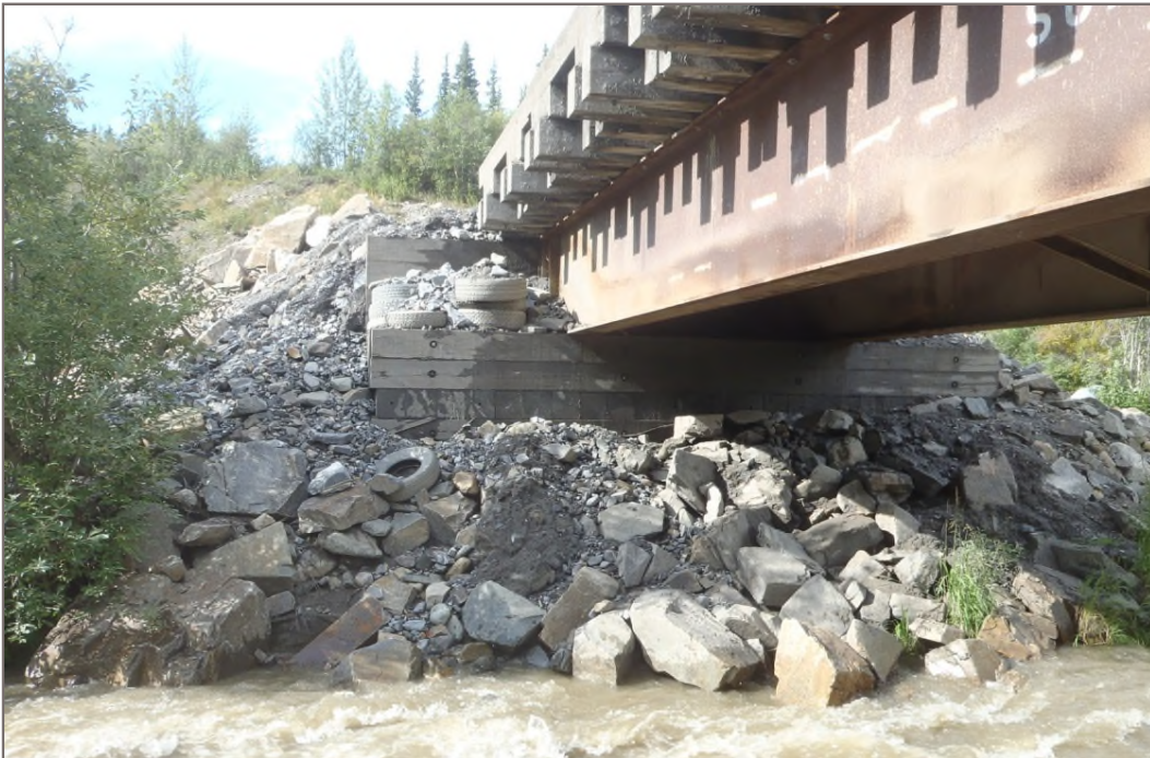
Photo 18: Lightning Creek Bridge Abutments (Bellekeno Haul Road) Rip-rap armouring bridge abutments Facing west – August 12, 2014
