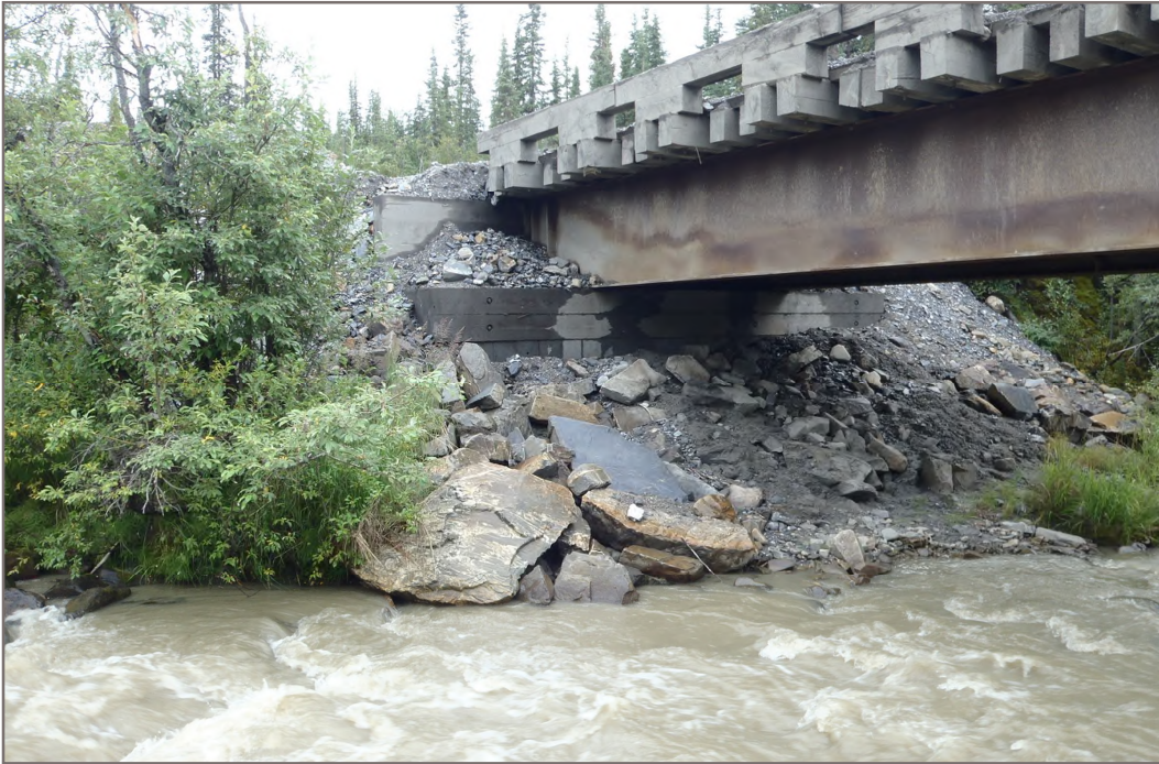
Photo 13: Lightning Creek Bridge Abutments (Bellekeno Haul Road) Stable abutment and sufficient rip-rap armouring Facing South - August 10, 2015
