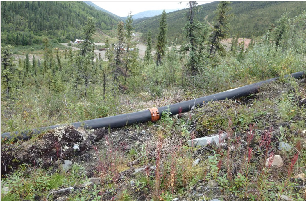
Photo 8: Bellekeno 625 Water Treatment Ponds Bend in discharge pipe at coupler Facing East - August 10, 2015
