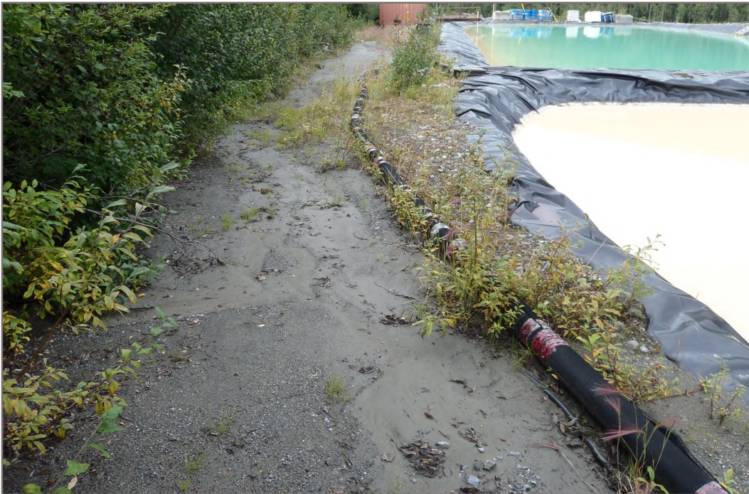
Photo 6: Bellekeno 625 Water Treatment Ponds Sediment deposited outside southwest corner of facility Facing North - August 10, 2015
