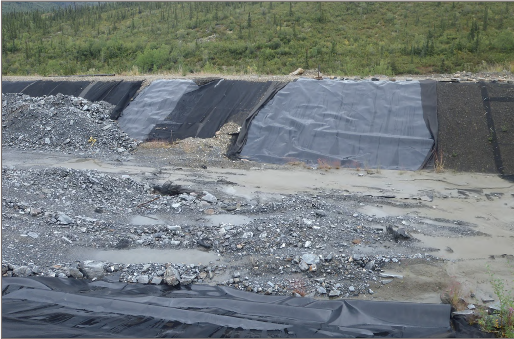
Photo 3: PAG Waste Storage Facility Liner components displaced due to wind Facing East - August 10, 2015
