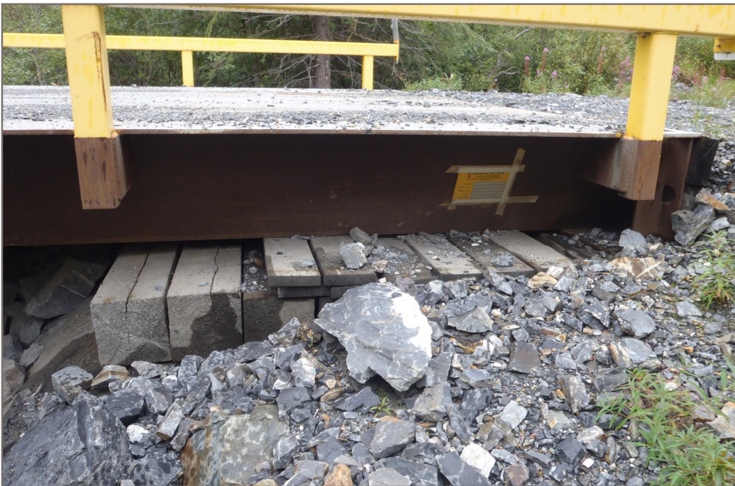
Photo 10: Lightning Creek Bridge Abutments (Onek Road) South bridge abutment Facing East - August 10, 2015
