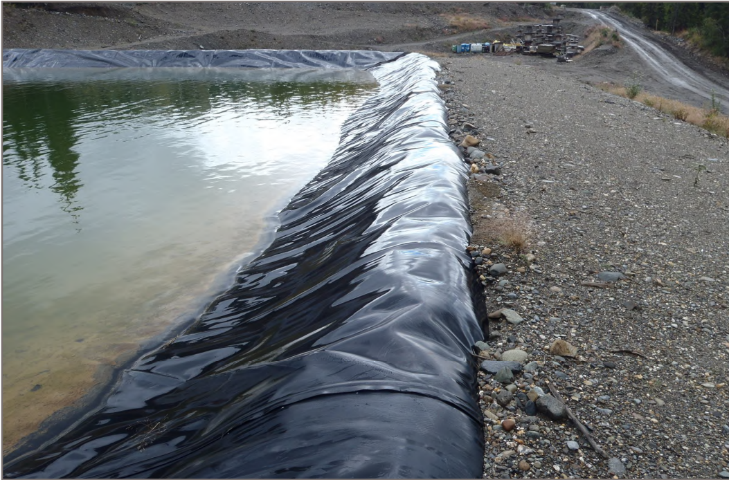
Photo 15: Mill Water Storage Pond Stable perimeter berm and intact liner Facing South - August 11, 2015
