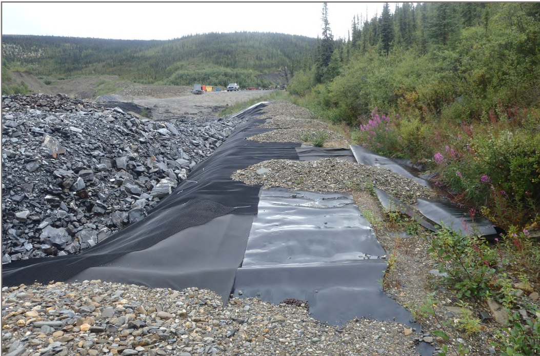
Photo 2: PAG Waste Storage Facility Incomplete anchor trench on north and west side of facility Facing South - August 10, 2015
