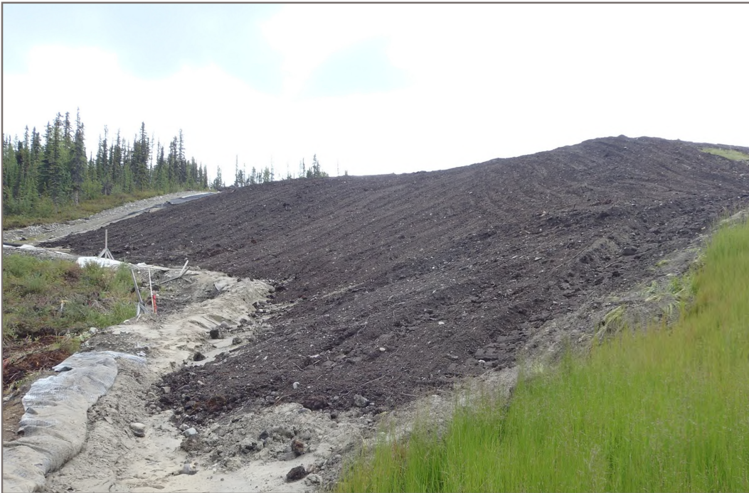
Photo 18: Dry Stacked Tailings Facility Surface of DSTF covered with growth medium Facing South - August 11, 2015
