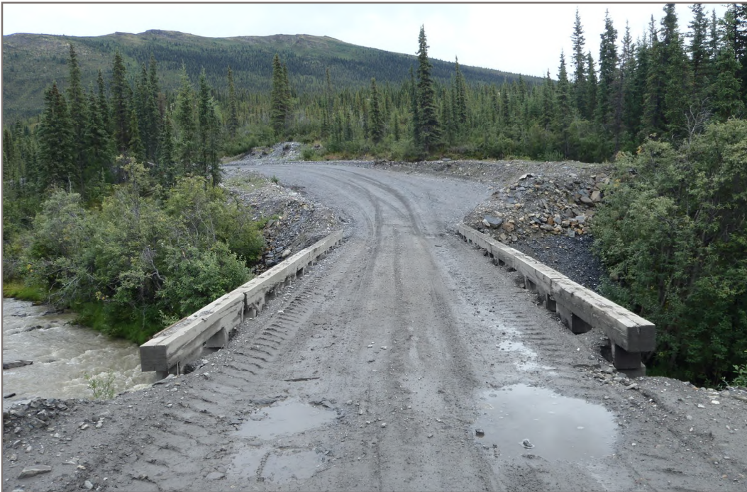
Photo 12: Lightning Creek Bridge Abutments (Bellekeno Haul Road) Bridge overview Facing South - August 10, 2015
