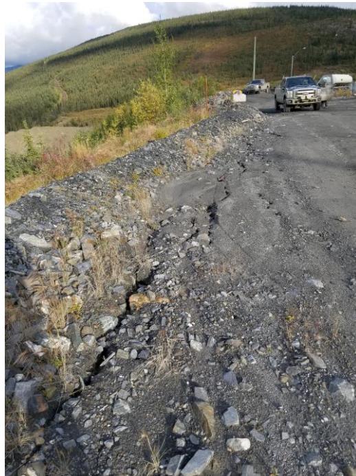
Photo 4: Bellekeno 625 Water Treatment Ponds Access Road Tension Cracks August 24, 2017
