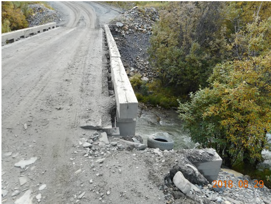
Photo 5: Bellekeno Haul Road bridge crossing Lightning Creek – erosion protection is required at the ends of the approaches to the bridge to protect the abutments and the bridge deck
