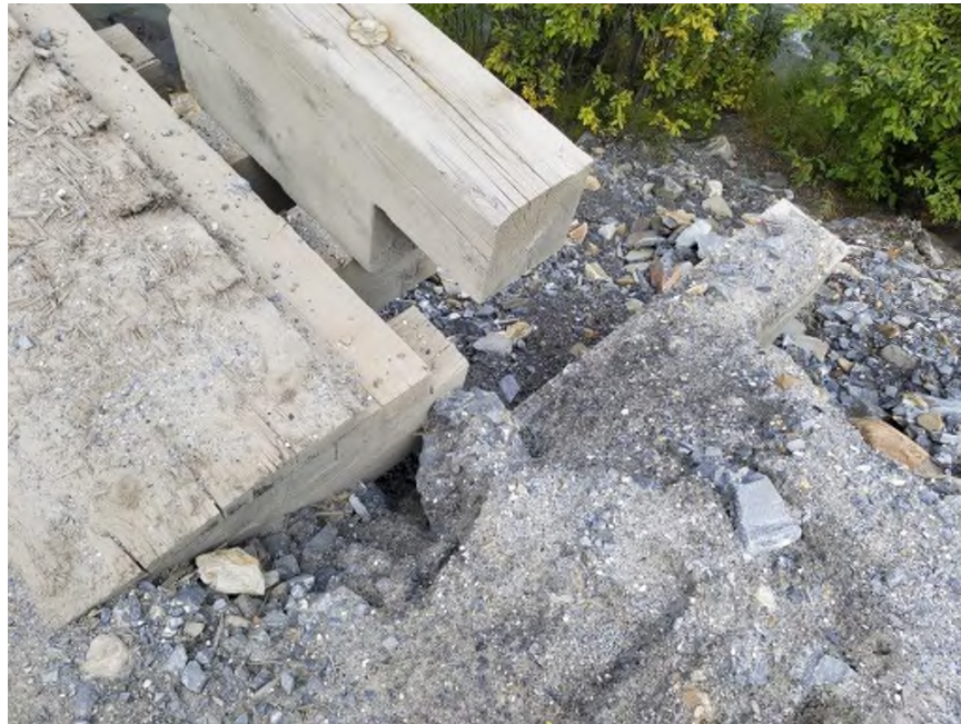
Photo 5 - Bellekeno Haul Road, Approach Erosion (August 20/19)
