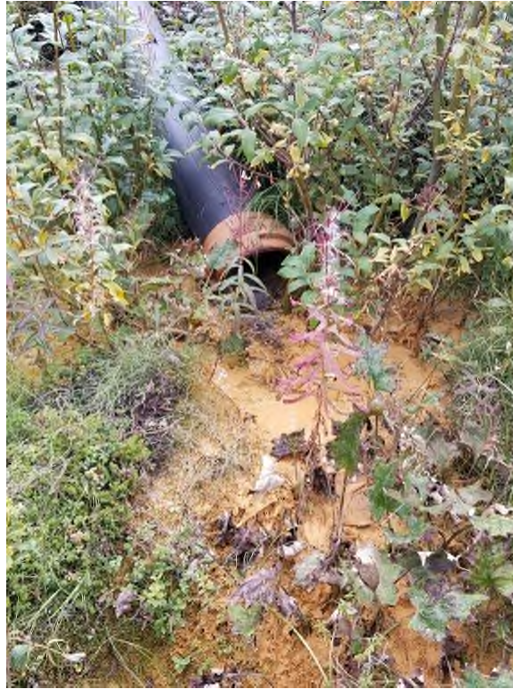
Photo 4 - Bellekeno 625 Water Treatment Ponds, Discharge Location (August 20/19)
