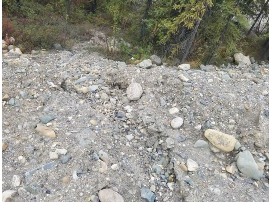
Photo 8 - Mill Storage Ponds, Access Road Erosion (August 2019)
