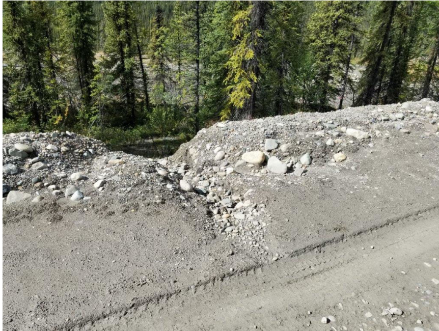
Photo 8 - Mill Storage Ponds, Access Road Erosion (August 18/20)
