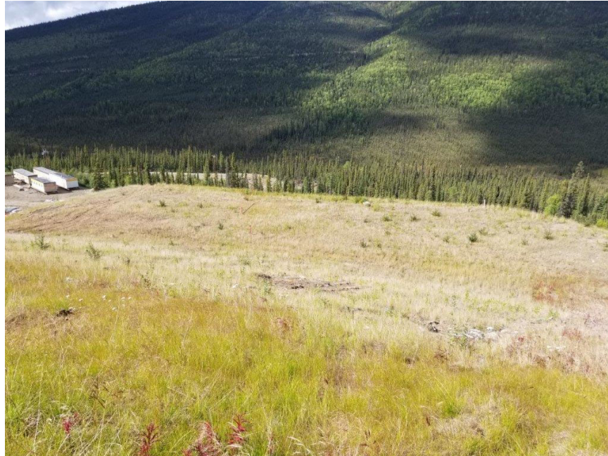
Photo 9 – DSTF Surface Showing some Repaired Tension Cracks (August 18/20)
