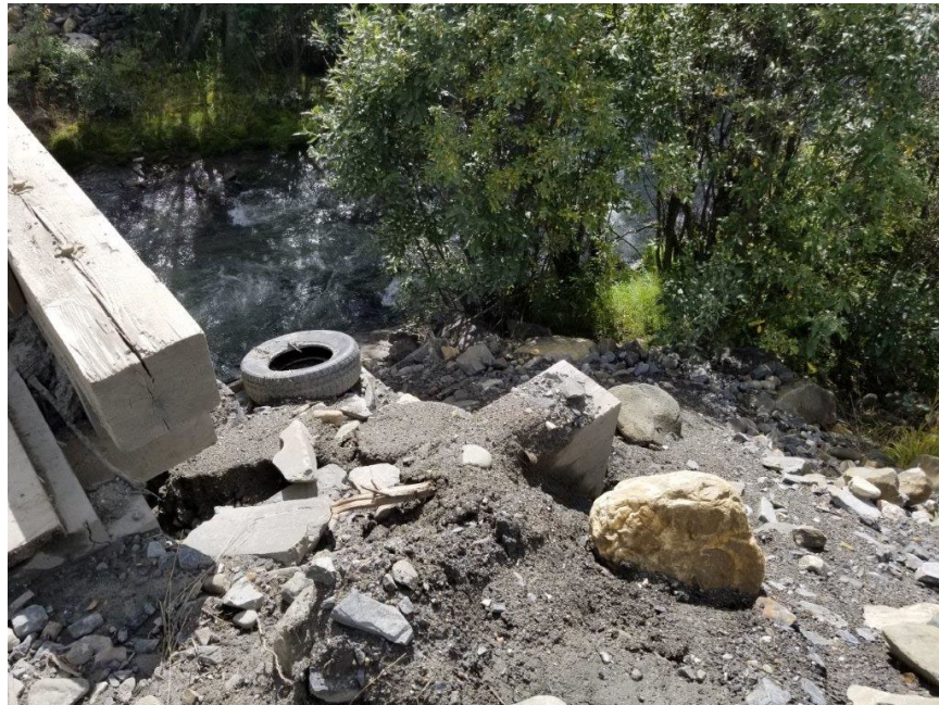
Photo 5 - Bellekeno Haul Road, Approach Erosion (August 08/20)
