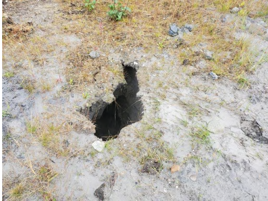
Photo 9: DSTF Sinkhole (August 26/21)
