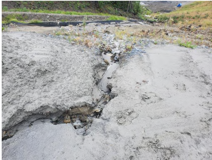
Photo 11: DSTF Tailings Erosion (August 26/21)
