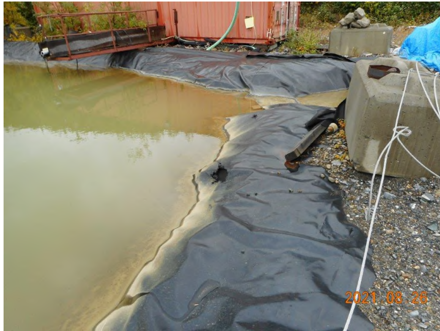
Photo 3: Small Rip in Liner at Bellekeno 625 Water Treatment Ponds (August 26/21)
