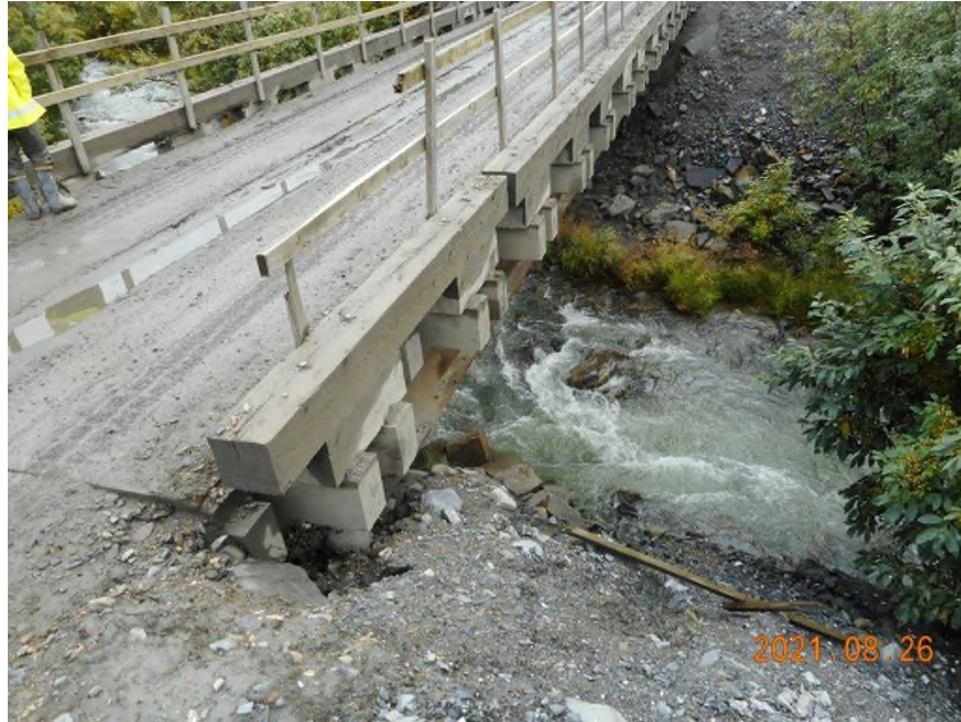
Photo 5: Bellekeno Haul Road, Approach Erosion (August 26/21)
