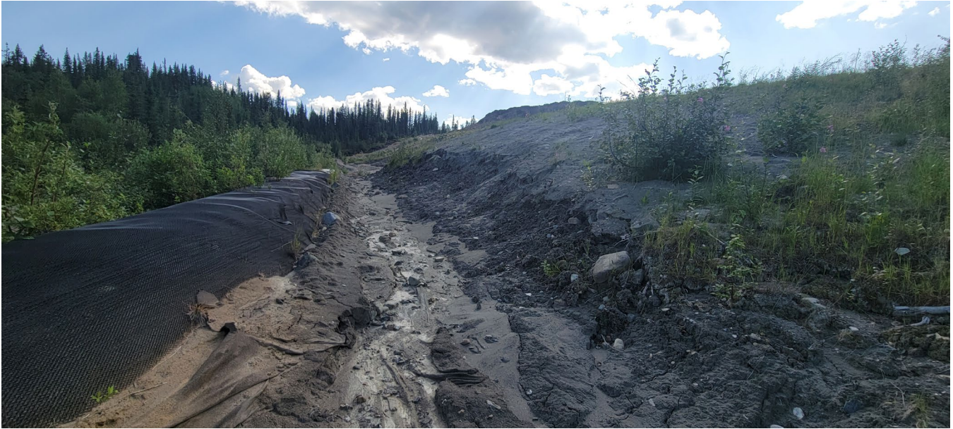
Photo 19: DSTF Phase 1 north perimeter runoff collection ditching, Facing North. Typical, showing exposed an unanchored liner and buildup of sediment. (I. MacIntyre, July 22, 2023)
