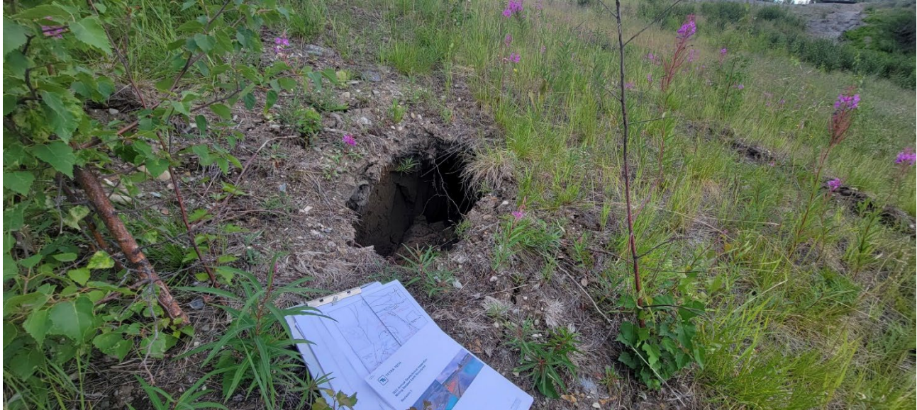
Photo 16: DSTF Phase 1A area, southwest slope. Small sink hole indicating migration of materials. Extends below cover into tailings. Erosion gully visible in background (I. MacIntyre, July 20, 2023)
