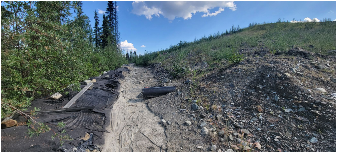
Photo 18: DSTF Phase 1 south west runoff collection ditching, Facing North. Typical, showing exposed an unanchored liner and buildup of sediment. (I. MacIntyre, July 20, 2023)
