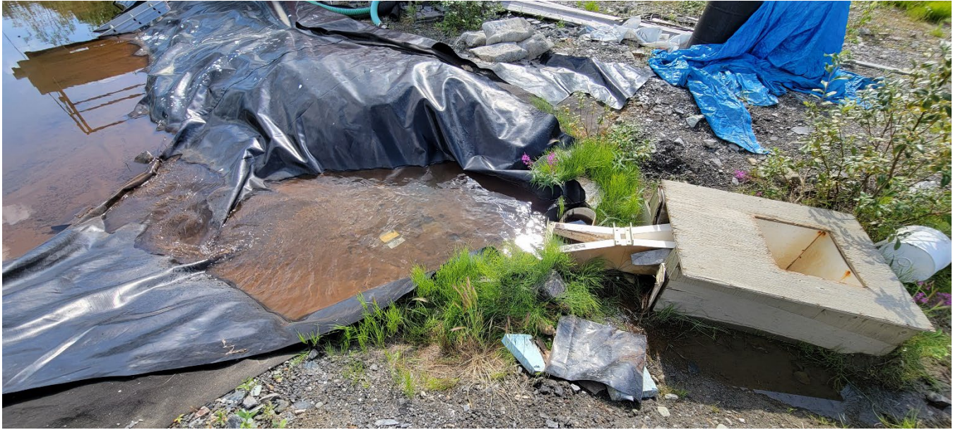
Photo 5: Bellekeno 625 Water Treatment Ponds, outlet structure. Note unsupported liner and flume. (I. MacIntyre, July 20, 2023)
