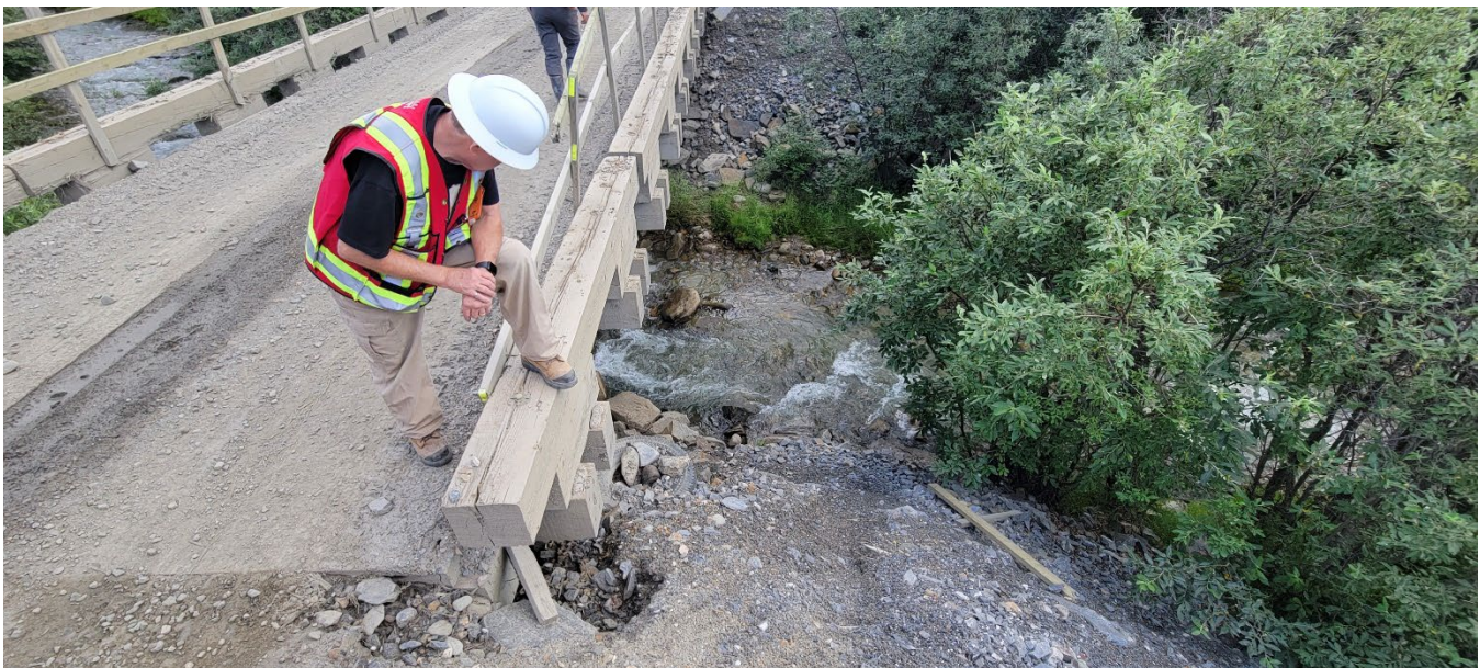
Photo 7: Lightning Creek Bridge – Bellekeno Haul Road, erosion along abutment (I. MacIntyre, July 20, 2023)
