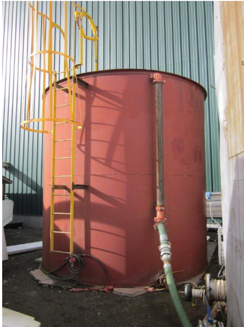
Figure 3-29 Fresh Water Tank
