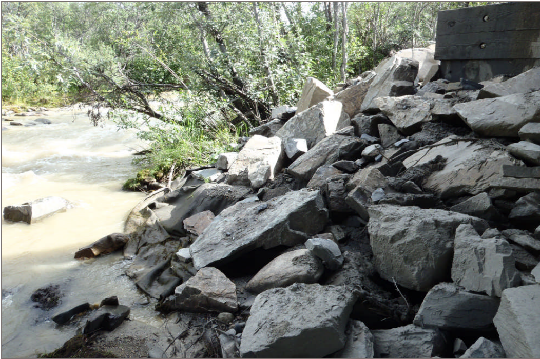
Photo 13: Exposed geotextile on south bank of Lightning Creek requiring additional riprap placement (Facing east – July 28, 2011)
