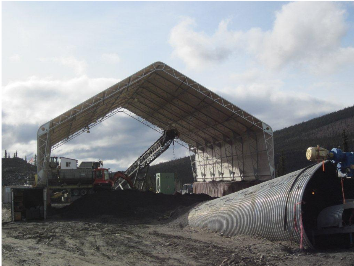
Figure 3-18 Fine Ore Stockpile
