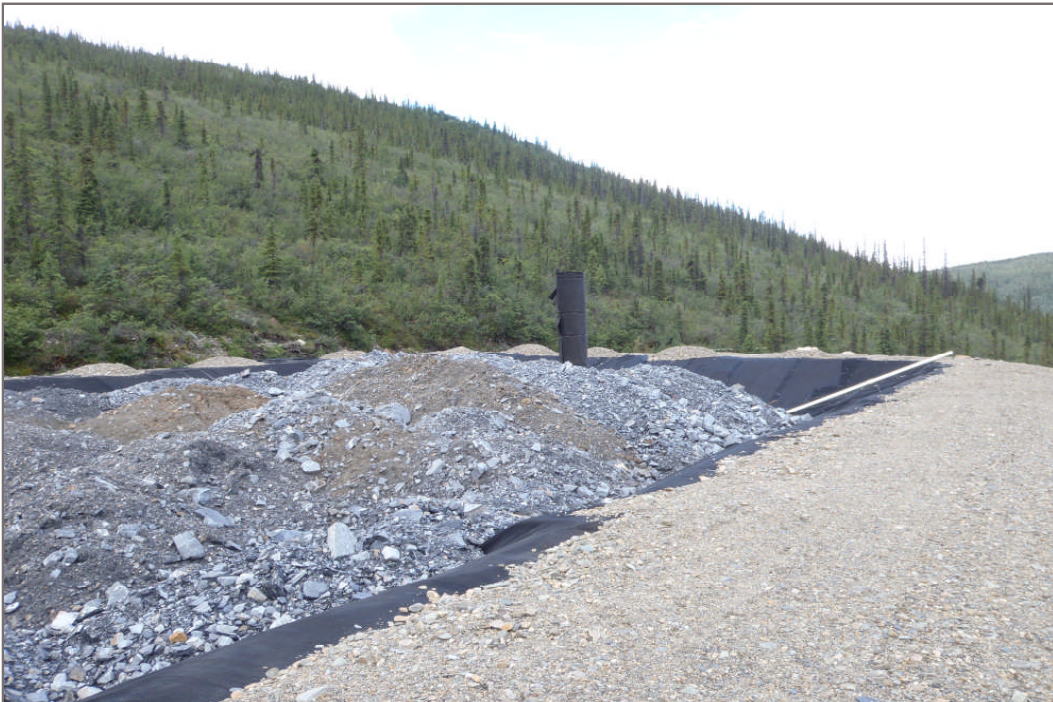
Photo 2: Geotextile wrapped vertical culvert, waste piles, completed portion of liner system (Facing north – July 28, 2011)
