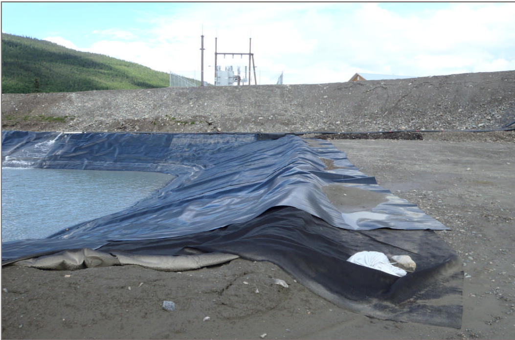
Photo 16: Incomplete liner anchoring trench at east end of mill water storage pond (Facing north – July 28, 2011)
