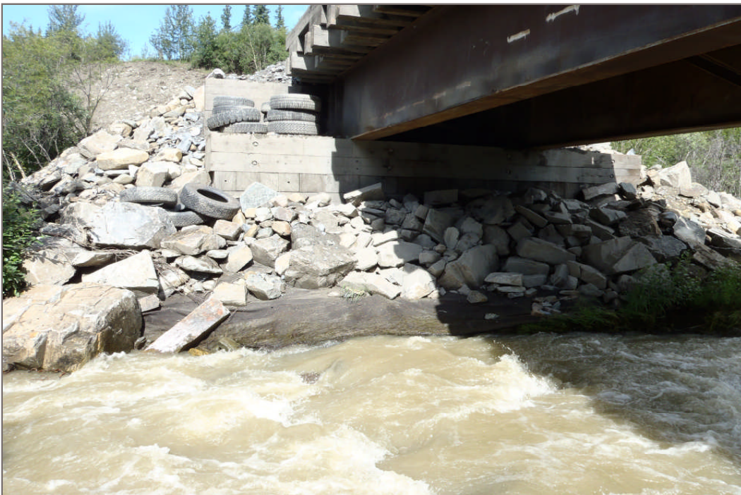
Photo 12: Exposed geotextile on north bank of Lightning Creek requiring additional riprap placement (Facing north – July 28, 2011)
