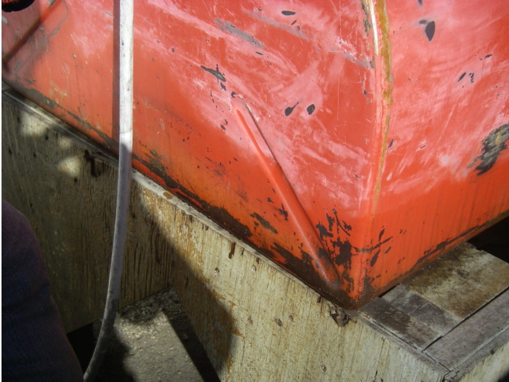
Photo 1: Source of leak
