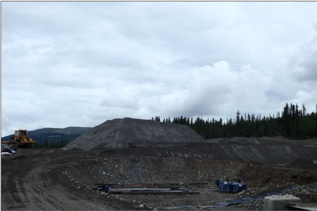
Photo 18: Existing pile crest exceeds design elevation; the pile should be reshaped to design dimensions (Facing north – July 28, 2011)
