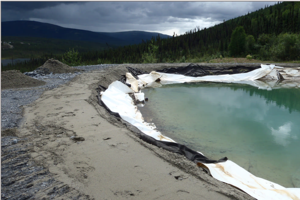
Photo 20: Exposed berm and liner system falling into pond (Facing south – July 28, 2011)
