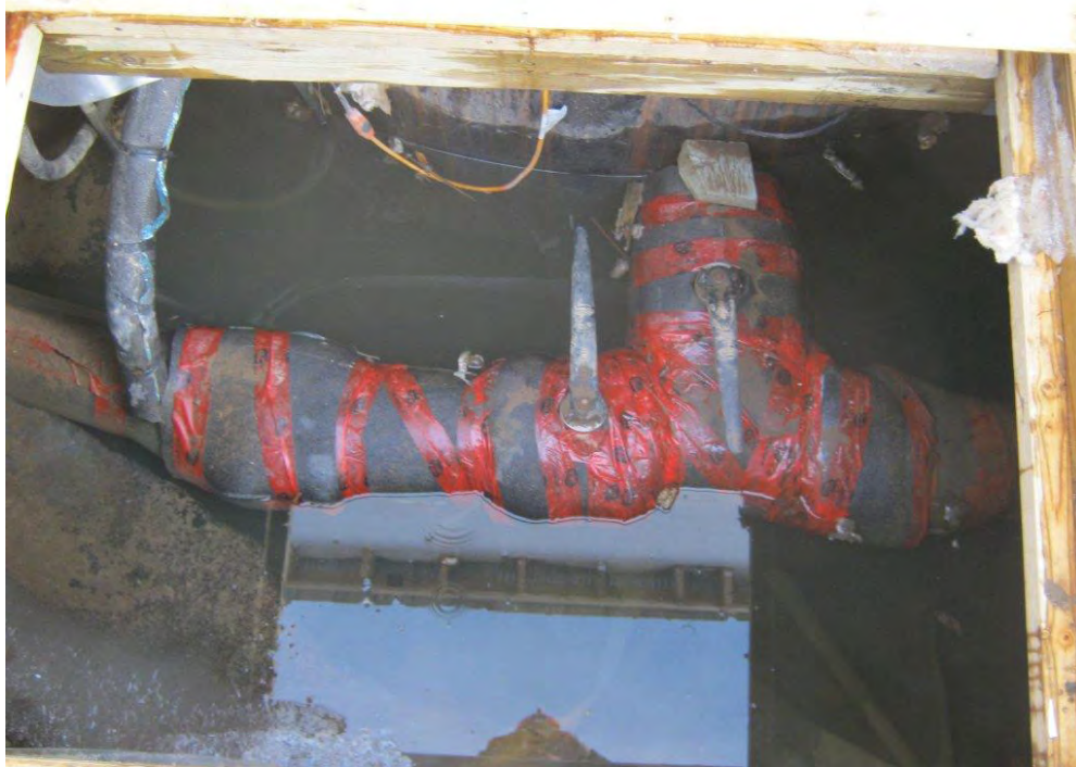
FIGURE 8 – BIOREACTOR DISCHARGE VALVES
