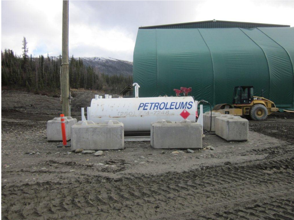
Figure 3-31 Diesel Storage Tanks
