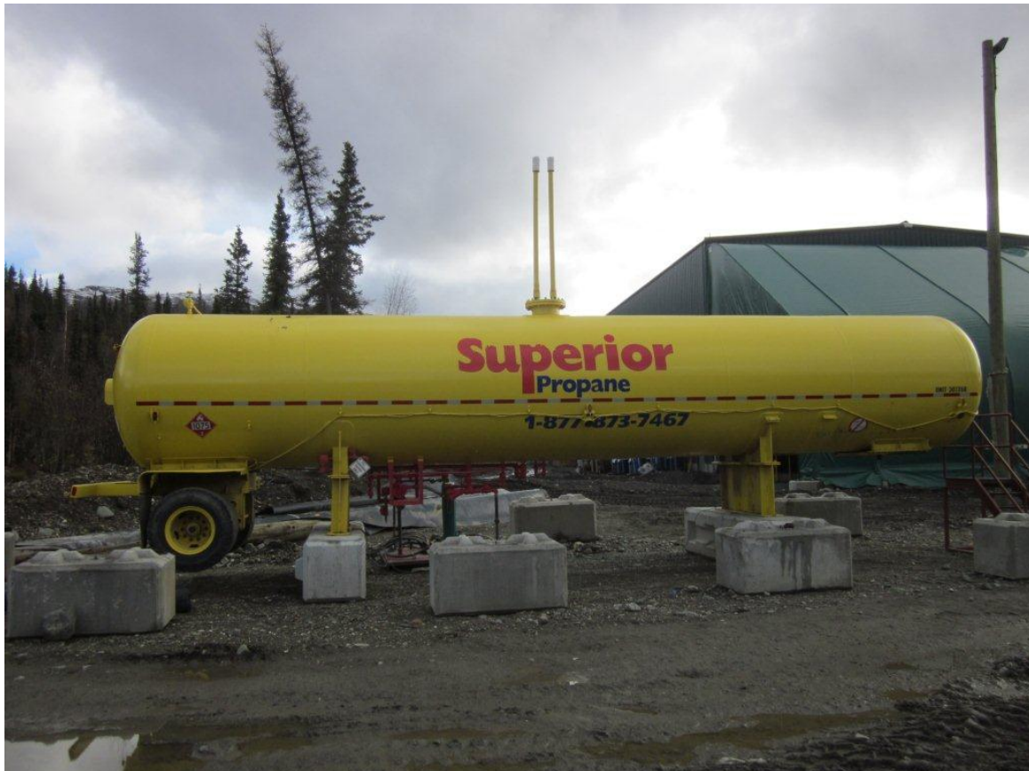
Figure 3-32 Propane Storage Tank
