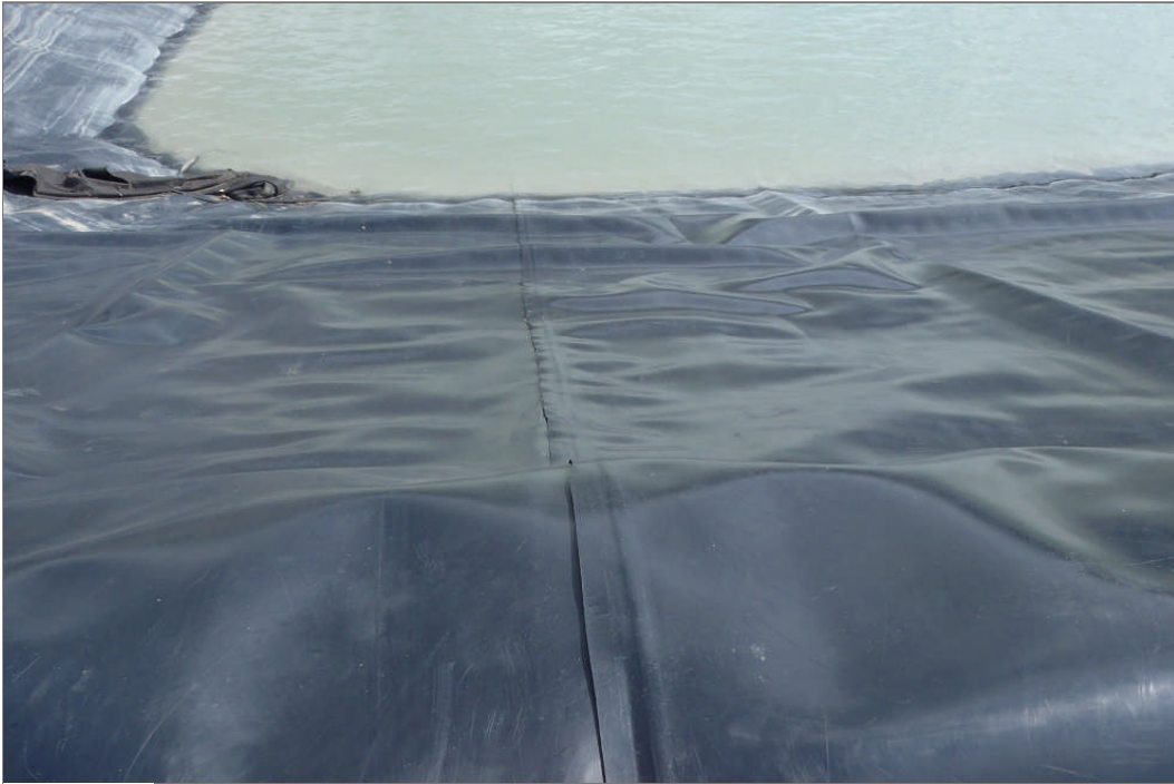
Photo 15: Typical seem in liner of mill water storage pond (Facing east – July 28, 2011)
