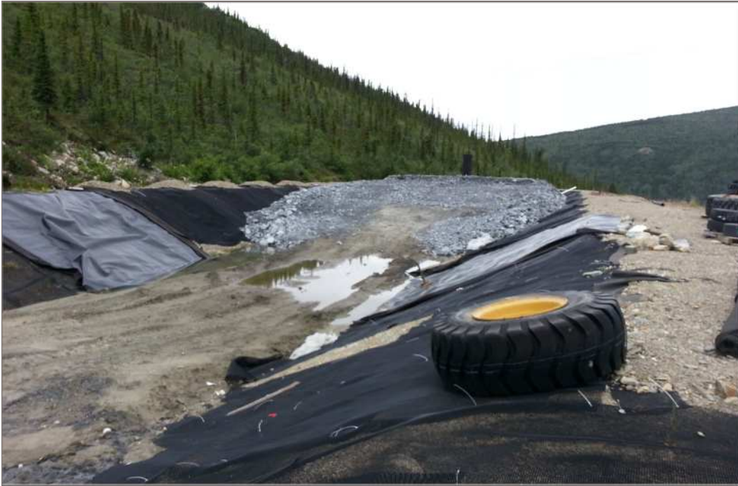
Photo 1: PAG Waste Storage Facility Completed and partially completed sections of liner. July 13, 2012
