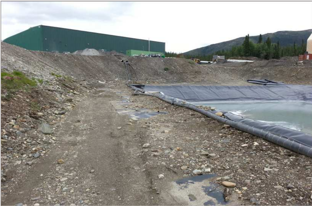
Photo 14: Mill Water Storage Pond Exposed liner along pond berm July 13, 2012
