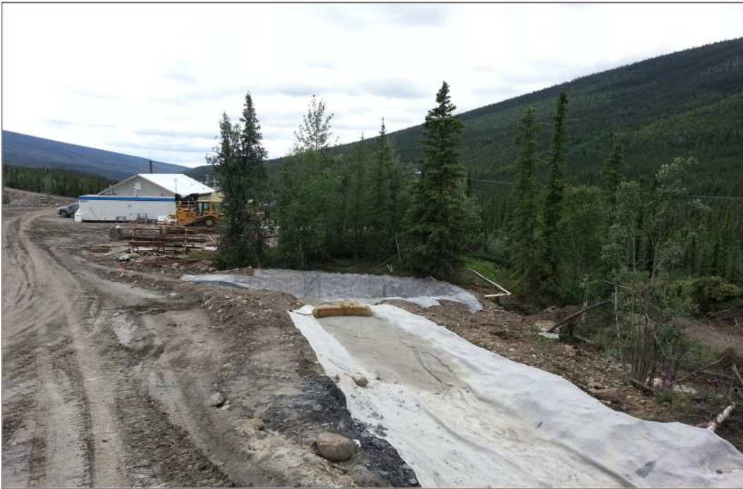
Photo 20: DSTF Lower Bench Seepage collection system July 13, 2012
