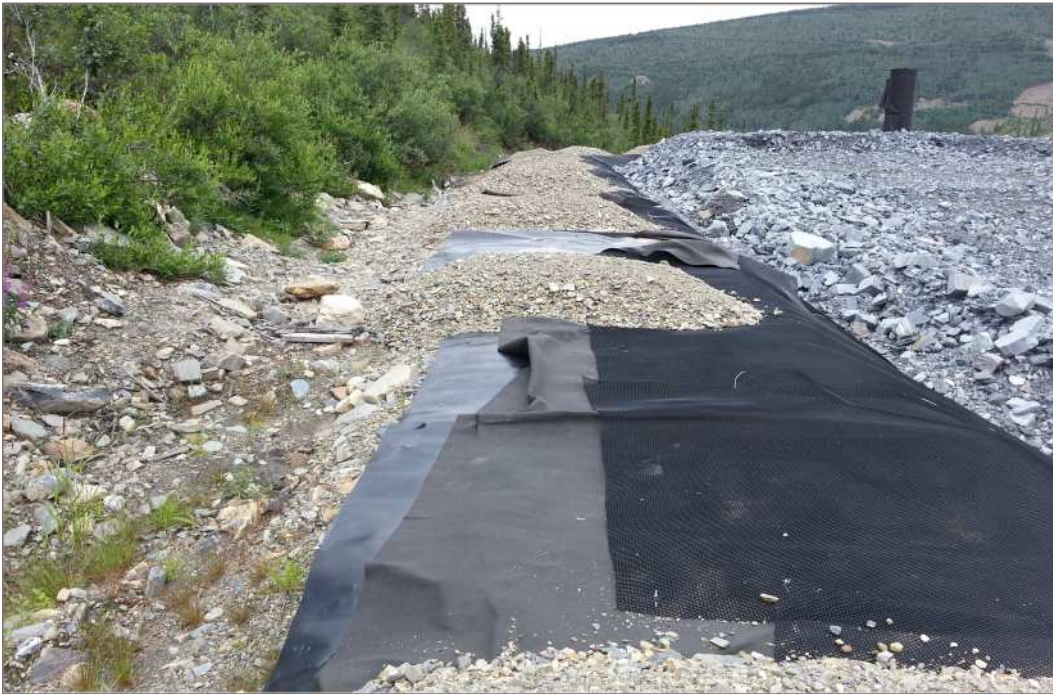
Photo 2: PAG Waste Storage Facility Liner not adequately anchored along west berm July 13, 2012
