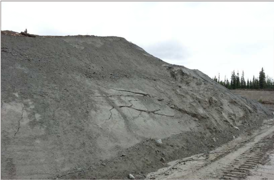
Photo 18: DSTF Lower Bench Cracking on south slope along haul road July 13, 2012
