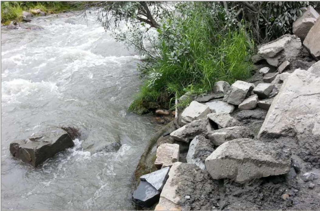
Photo 12: Lightning Creek Bridge Abutments Exposed geotextile on East Abutment July 13, 2012
