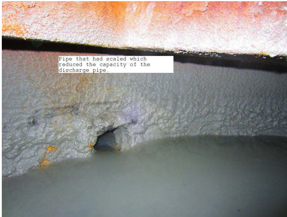
Spill Photo 6: Scaled pipe within Primary Mix Tank
